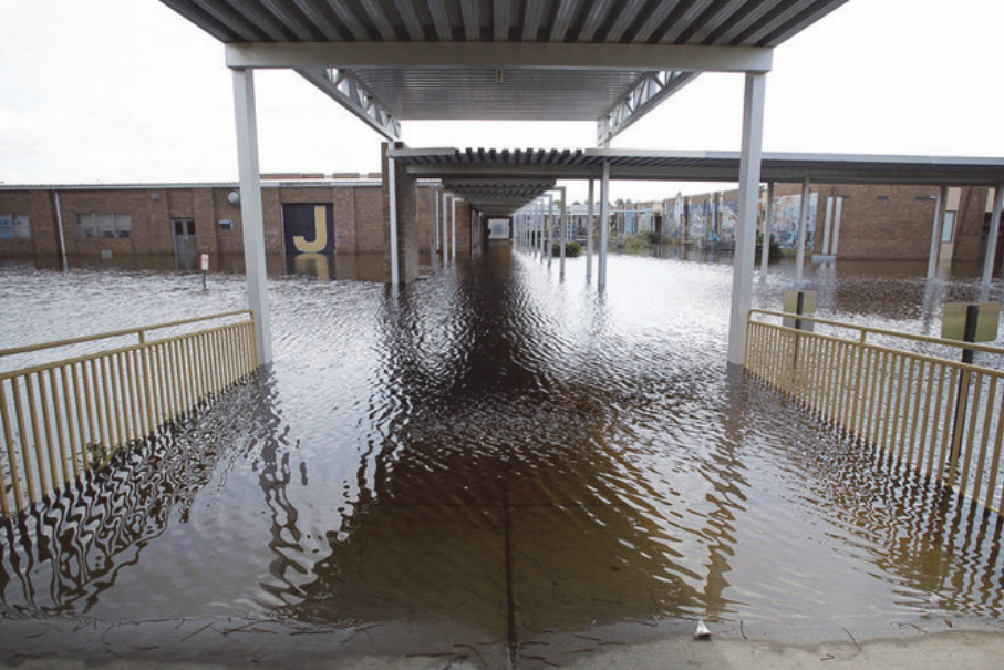
Figure H-5 Storm surge flooding in a high school in LaPlace, Louisiana during Hurricane Isaac in 2012. (Photo source: Rusty Costanza, The Times-Picayune )
