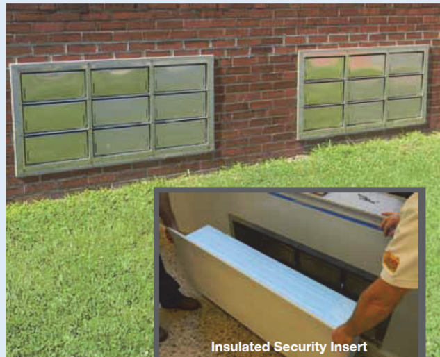
Figure F-8 Flood vents were installed throughout most of the school. Allowing floodwater to enter prevents structural failure of walls if water is outside but not inside (Smart Vent, 2016).
