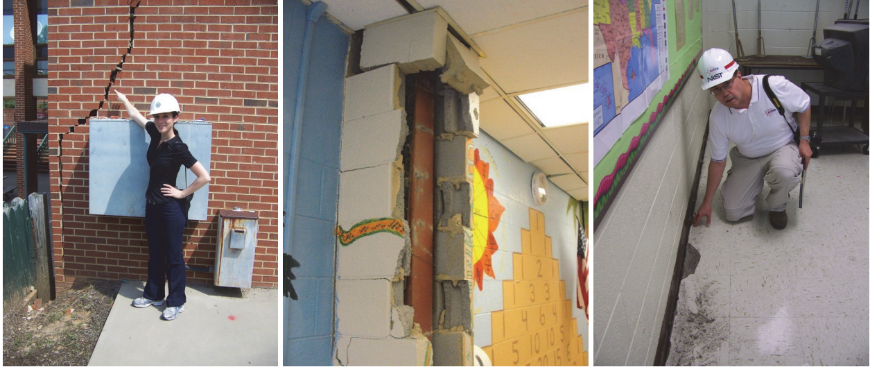
Figure 5-1 Photos documenting earthquake damage to school buildings. (Photo source: Michael Mahoney, FEMA)
