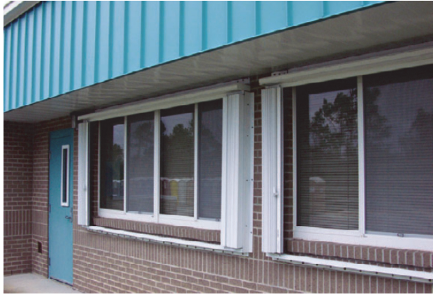
Figure H-15 This school was retrofitted with accordion shutters prior to a hurricane. The shutters successfully protected the windows from wind-borne debris during 2004 Hurricane Ivan (FEMA, 2010a).
