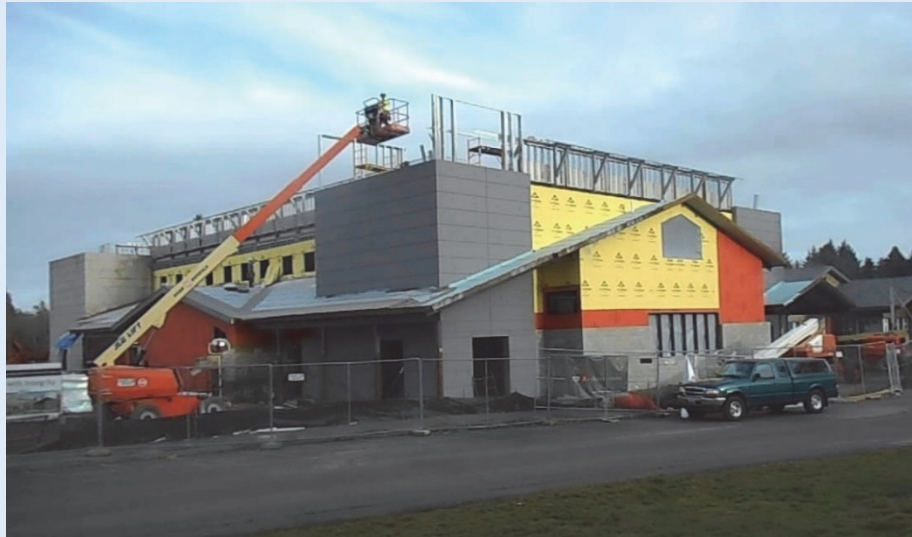
Figure TS-4 Ocosta Elementary School’s heavily reinforced vertical evacuation structure under construction in Westport, Washington (Magistrale, 2015).
