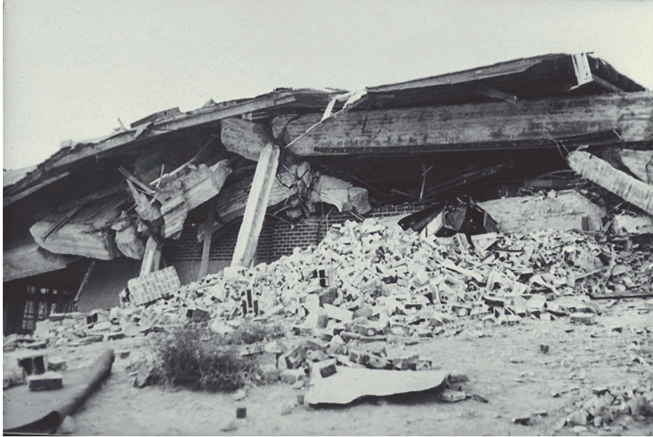
Figure E-5 Collapse of a portion of a concrete school in the Helena, Montana earthquake of 1935 (NISEE, 1935).
