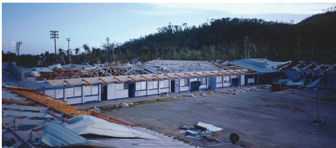
Figure H-19 Essentially the entire roof covering on this older school blew off (Typhoon Paka, Guam, 1997). It is often more economical to demolish an old school such as this and build a new school, rather than perform repairs and required upgrades.
