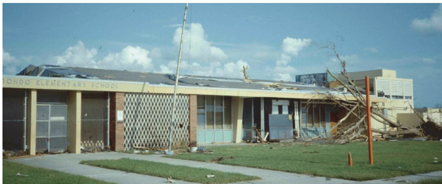
Figure H-12 Damage in a school in Florida during Hurricane Andrew in 1992. Several windows in this school were broken by wind-borne debris, and a large portion of the roof membrane blew off. Resulting interior water damage precluded quick resumption of school. (Photo source: Thomas Smith)
