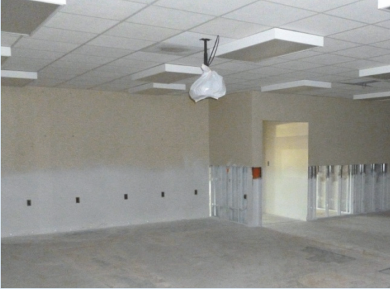
Figure F-6 Wall repair and reconstruction to resist future flood damage. (Photo source: Reynolds Restoration Services, Inc.)
