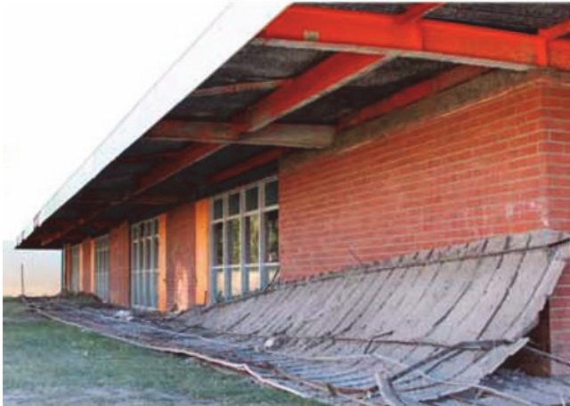
(a) Collapse of exterior soffit (i.e., exterior ceiling) at Jefferson Elementary School in the 2010 Baja, California earthquake. Soffit is made of plaster and is essentially the same weight as one inch of concrete.
