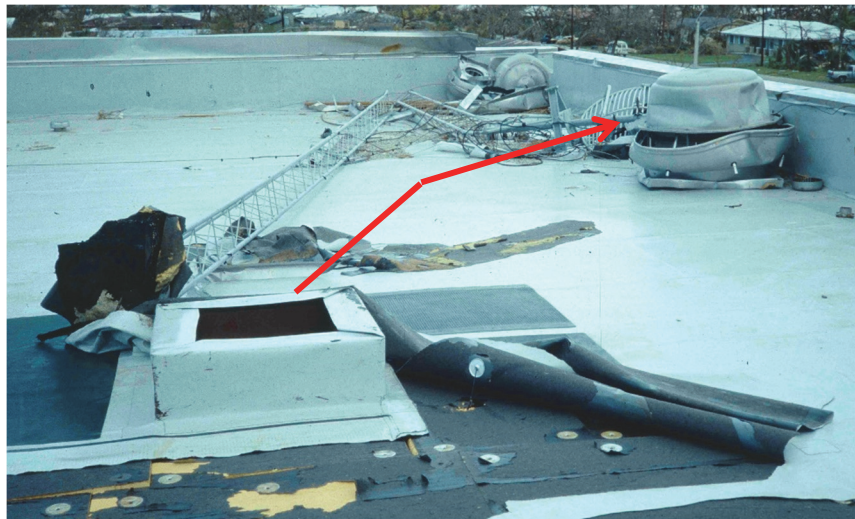
Figure H-14 Rooftop mechanical equipment is often inadequately attached (even on new schools). Several exhaust fans blew off their curbs, allowing rain to directly enter the school during Hurricane Andrew, Florida in 1992. It is very inexpensive to anchor equipment and avoid costly damage (FEMA, 2010a).
