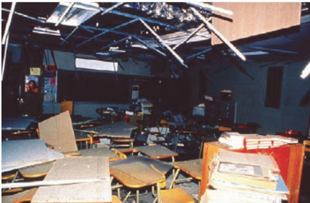
(b) Ceiling damage in a classroom in the 1994 Northridge earthquake.
