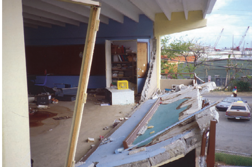
Figure H-13 Collapsed unreinforced masonry classroom wall in the U.S. Virgin Islands during Hurricane Marilyn in 1995 (FEMA, 2010a).
