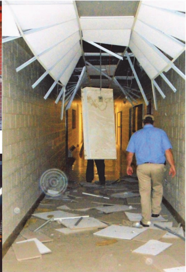
(c) Damage to Louisa County High School, Virginia. Ceiling and light fixture failure is very common in schools.
