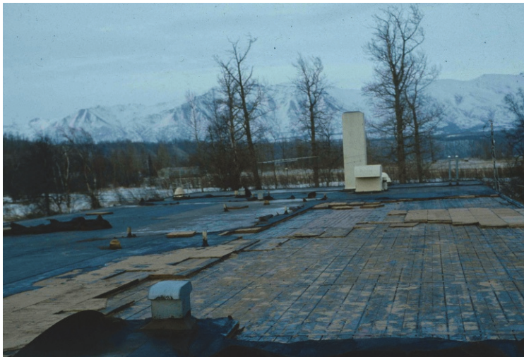
Figure W-2 The roof on this school blew off during cold weather, thus increasing the repair costs. (Photo source: Thomas Smith)
