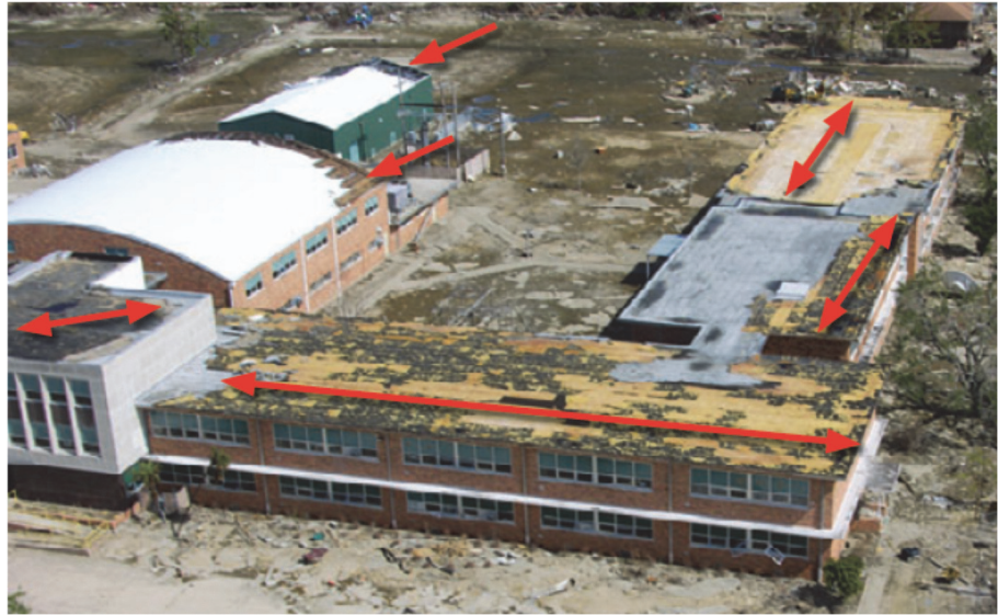
Figure H-3 Large portions of the school roof coverings blew off (indicated by red arrows) during 2005 Hurricane Katrina (FEMA, 2010a).
