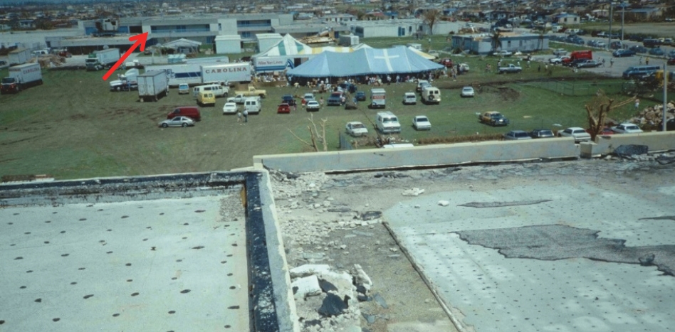
Figure H-17 View of aid tents between a damaged elementary school (red arrow) and high school (foreground) in Florida after Hurricane Andrew. (Photo source: Thomas Smith)
