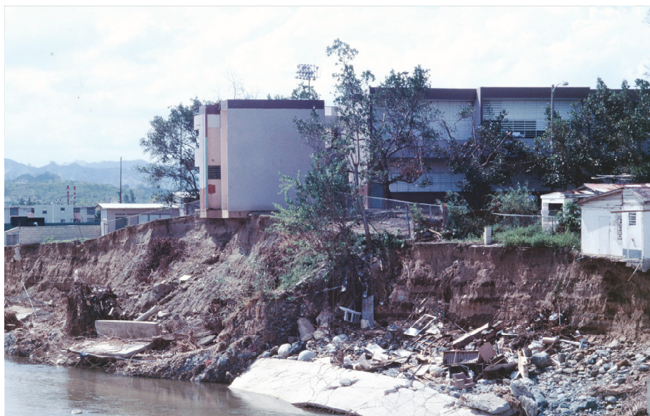
Figure F-3 This school in Puerto Rico was undermined by riverine erosion during Hurricane Georges in September 1998 (FEMA, 1999).
