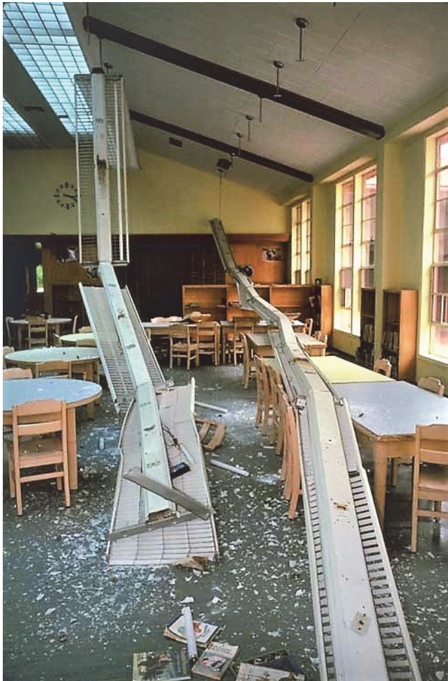
Figure E-7 Fallen light fixtures in a classroom after the Northridge earthquake. (Photo source: Earthquake Engineering Research Institute)
