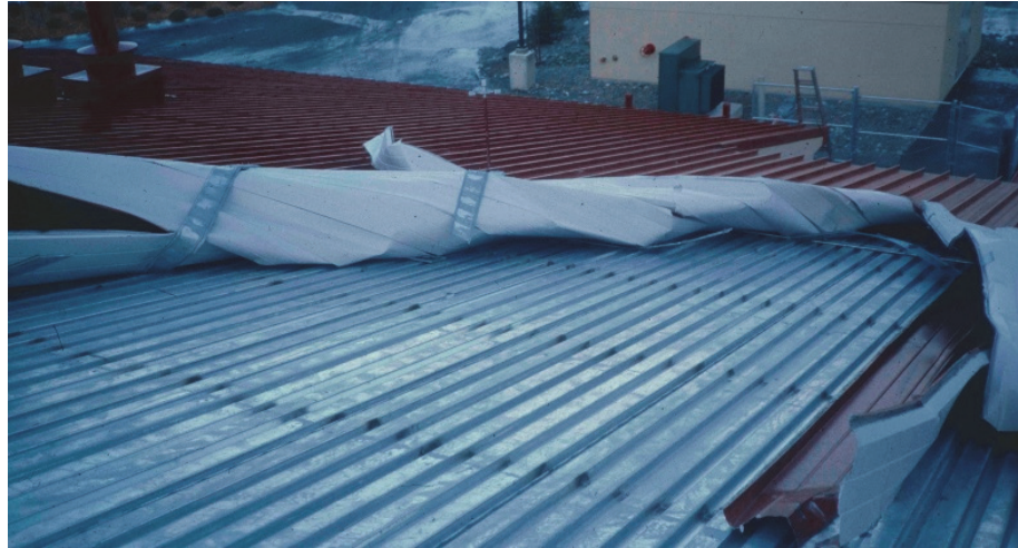
Figure W-1 The roof on this new school blew off during moderate winds soon after it was installed. It failed even though it was a robust system because of a major installation error. (Photo source: Thomas Smith)
