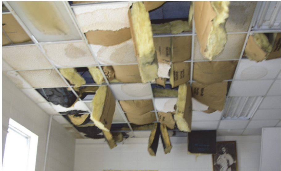
Figure H-4 Damage to school ceiling in Mississippi during 2005 Hurricane Katrina (FEMA, 2006b).
