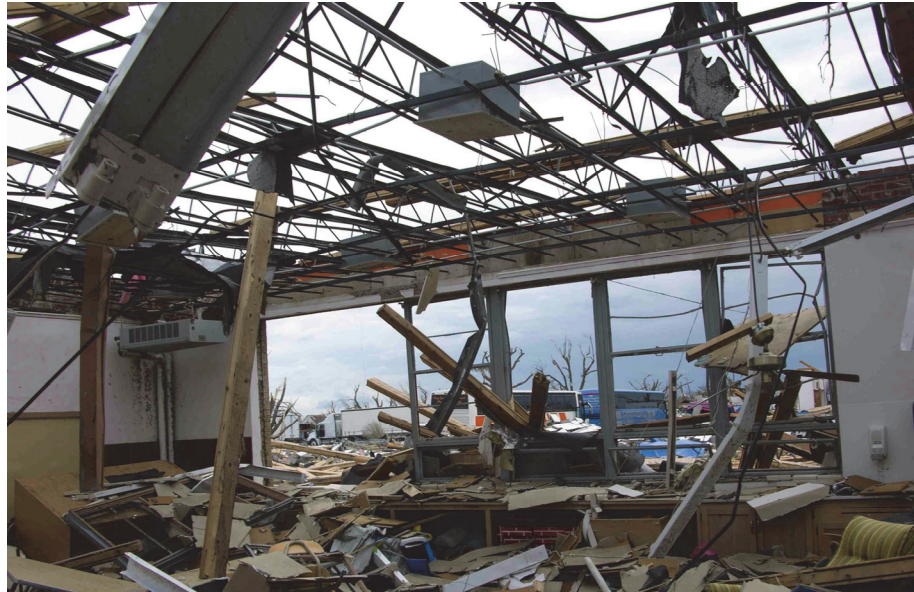
Figure TO-4 Wind-borne debris in a classroom in Greensburg, Kansas in 2007. Note that all of the exterior windows are broken and the roof deck was blown off. (Photo source: Thomas Smith, FEMA)
