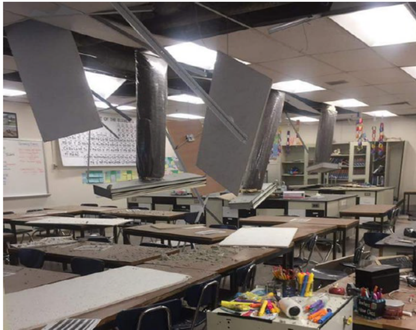
Damage to ceiling tiles in classroom of Eagle River Elementary School (EERI Earthquake Reconnaissance Report: M7.1 Anchorage Earthquake on November 30, 2018; photos: Chris Motter).
