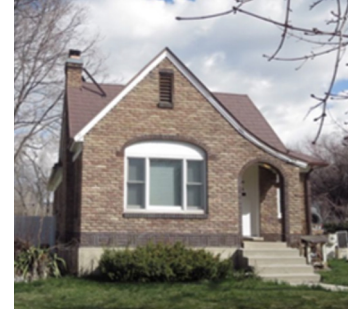
Salt Lake City home with braced chimney
