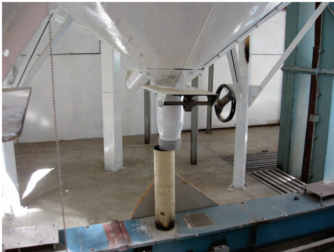
Figure 6.4.11.1-1 Misalignment between rice storage hopper and conveyor following the 2010 magnitude-8.8 Chile Earthquake (Photo courtesy of Rodrigo Retamales, Rubén Boroschek & Associates). Where various system components interface with a conveyor, the seismic restraints for the various parts should be coordinated to maintain alignment following an earthquake.
