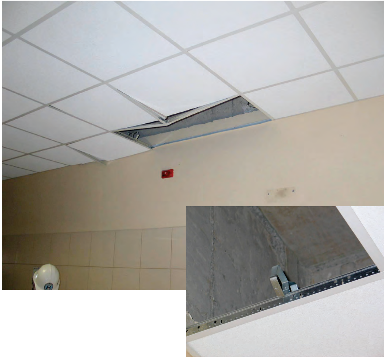
Figure 6.3.4.1-4 Fallen ceiling tiles at Talca Hospital in the 2010 Chile Earthquake, in spite of the use of clips as shown in detail at right. Most ceilings observed in Chile did not have seismic detailing (Photos courtesy of Bill Holmes, Rutherford & Chekene).
