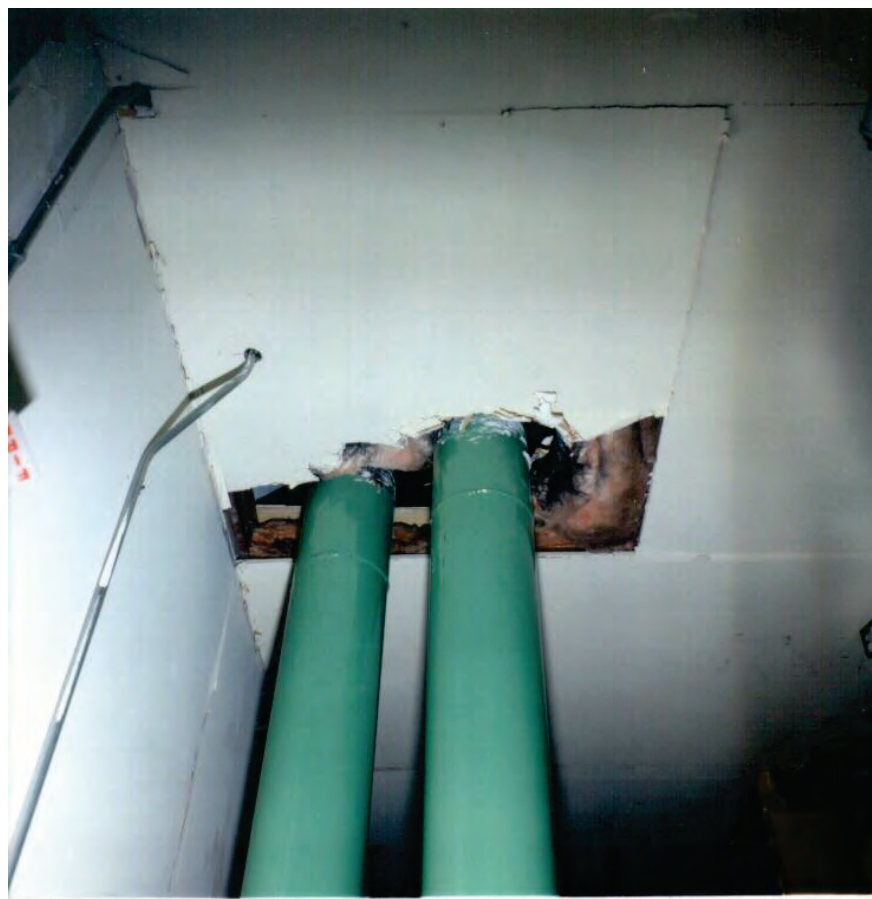
Figure 6.4.3.4-1 Movement of unbraced risers damaged ceiling finishes and insulation in the 1994 magnitude-6.7 Northridge Earthquake (Photo courtesy of Mason Industries).
