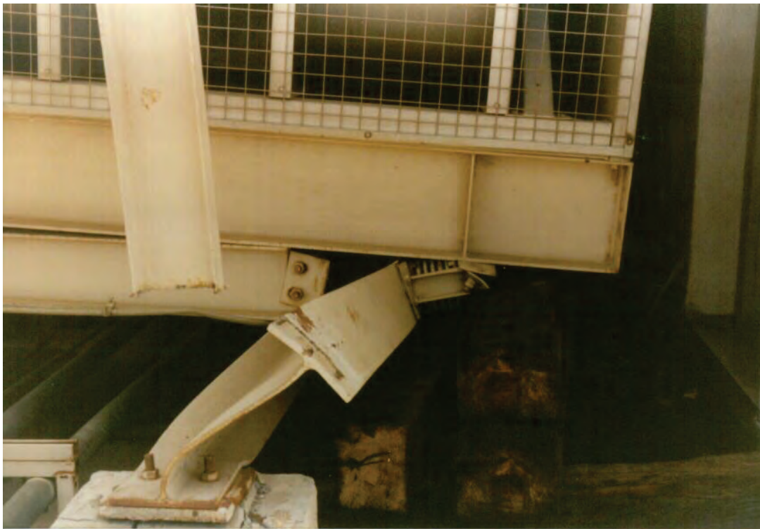
Figure 6.4.1.3-3 Failure of an entire support assembly including vibration isolators (Photo courtesy of Mason Industries).
