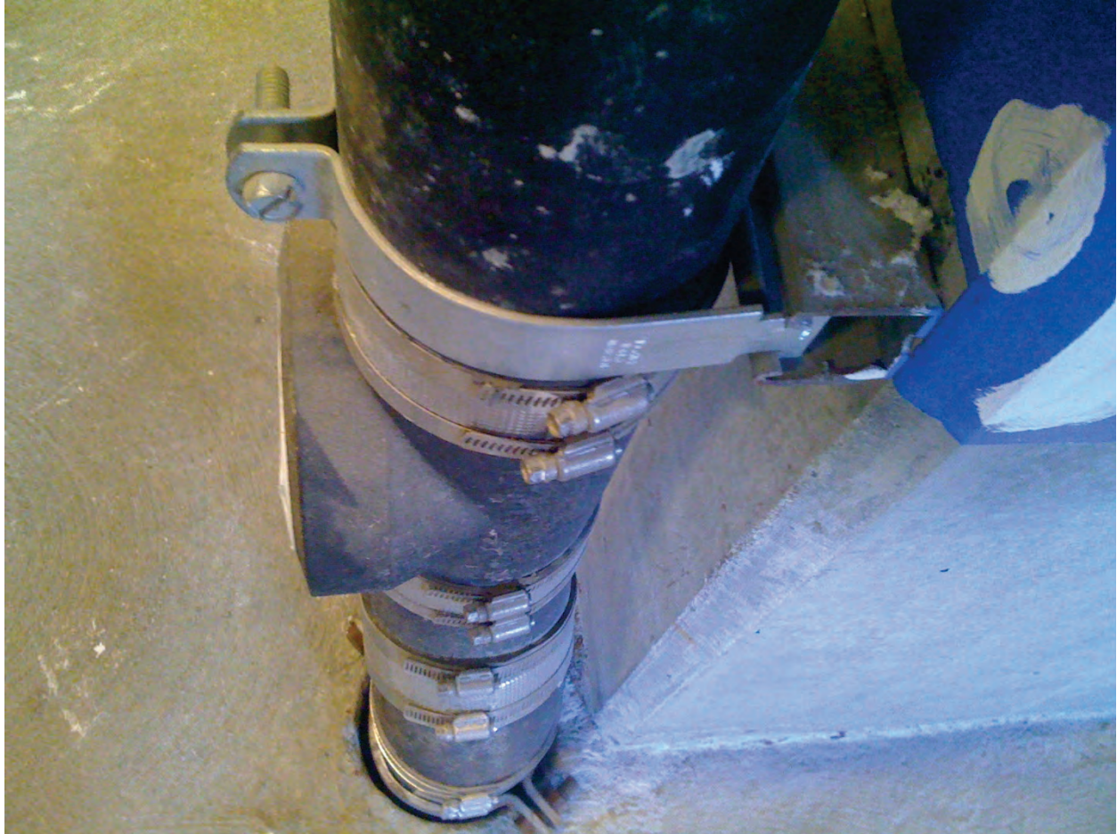
Figure 6.4.5.2-5 Poor example of sanitary sewer pipe support installed in San Francisco Bay Area in 2010; strut clamp has inadequate edge distance to end of strut and could slip off the end (Photo courtesy of Cynthia Perry, BFP Engineers).
