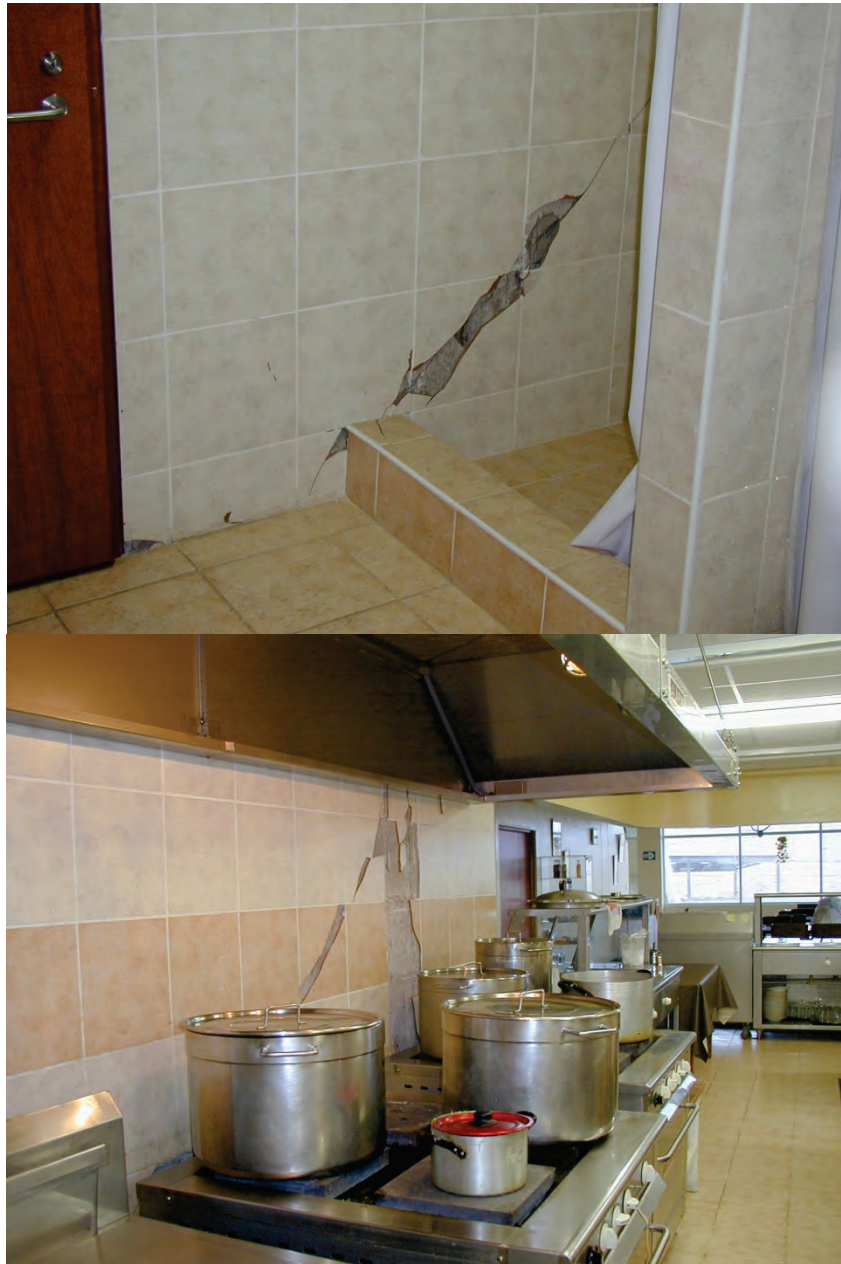
Figure 6.3.3.1-2 Damage to adhered tile veneer in locker room and kitchen at industrial facility in the 2001 Peru Earthquake (Photo courtesy of Eduardo Fierro, BFP Engineers). Tile was adhered to CMU partitions which were built integral with the concrete frame. While only a limited number of tiles were broken, equipment had to be disconnected and many tiles removed to repair cracks in the wall and facilitate the repair of the veneer.
