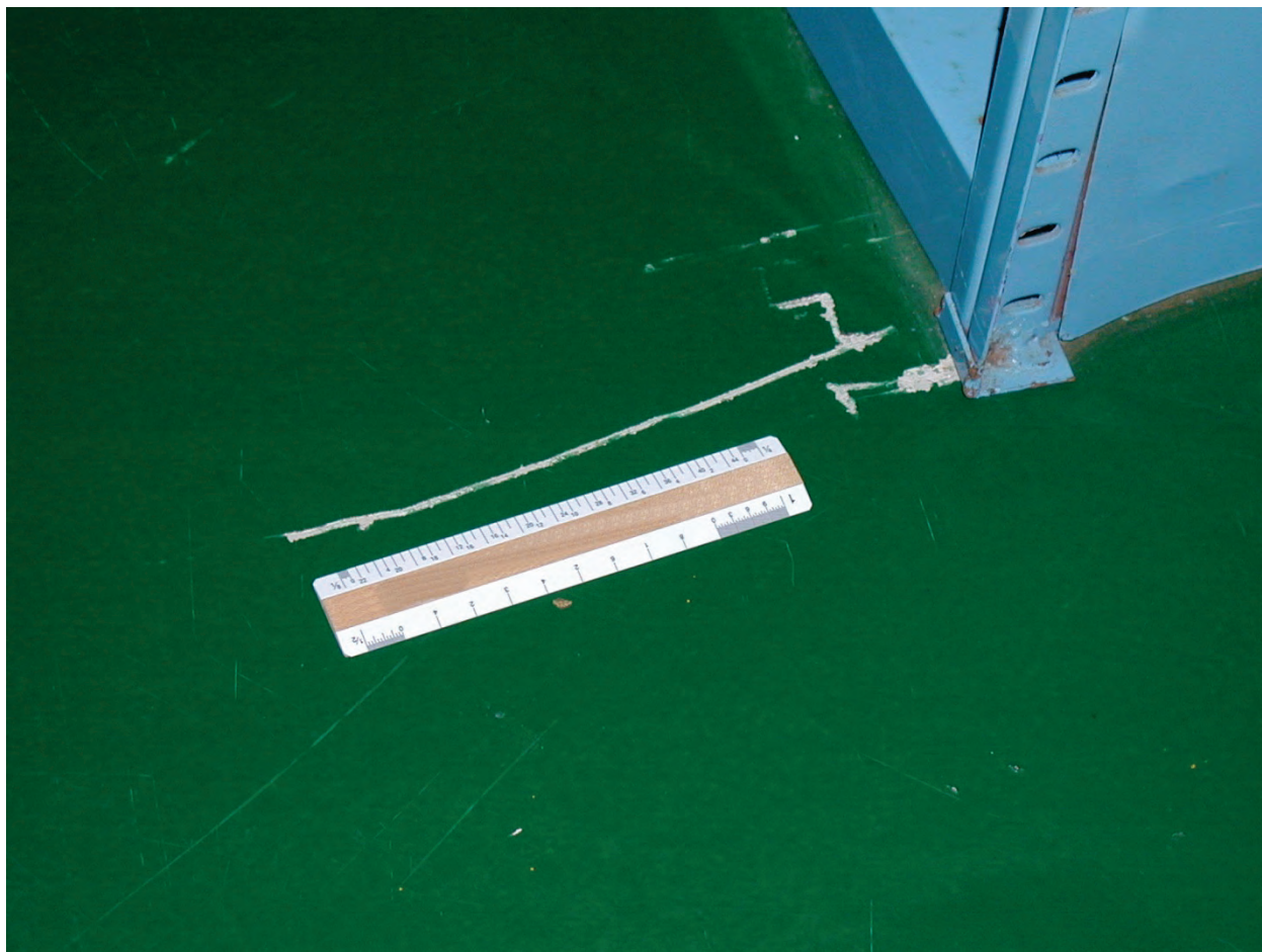
Figure 6.5.1.1-2 Unanchored storage shelving slid nine inches without falling but contents scattered in the 2001 magnitude-8.4 Peru earthquake; unit lifted to original position prior to photo (Photo courtesy of Eduardo Fierro, BFP Engineers).
