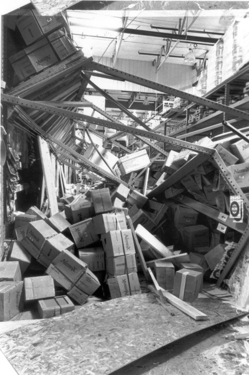
Figure 2.4.1-5 Damage to overloaded racks during the 1994 magnitude-6.7 Northridge Earthquake (FEMA 460, 2005).
