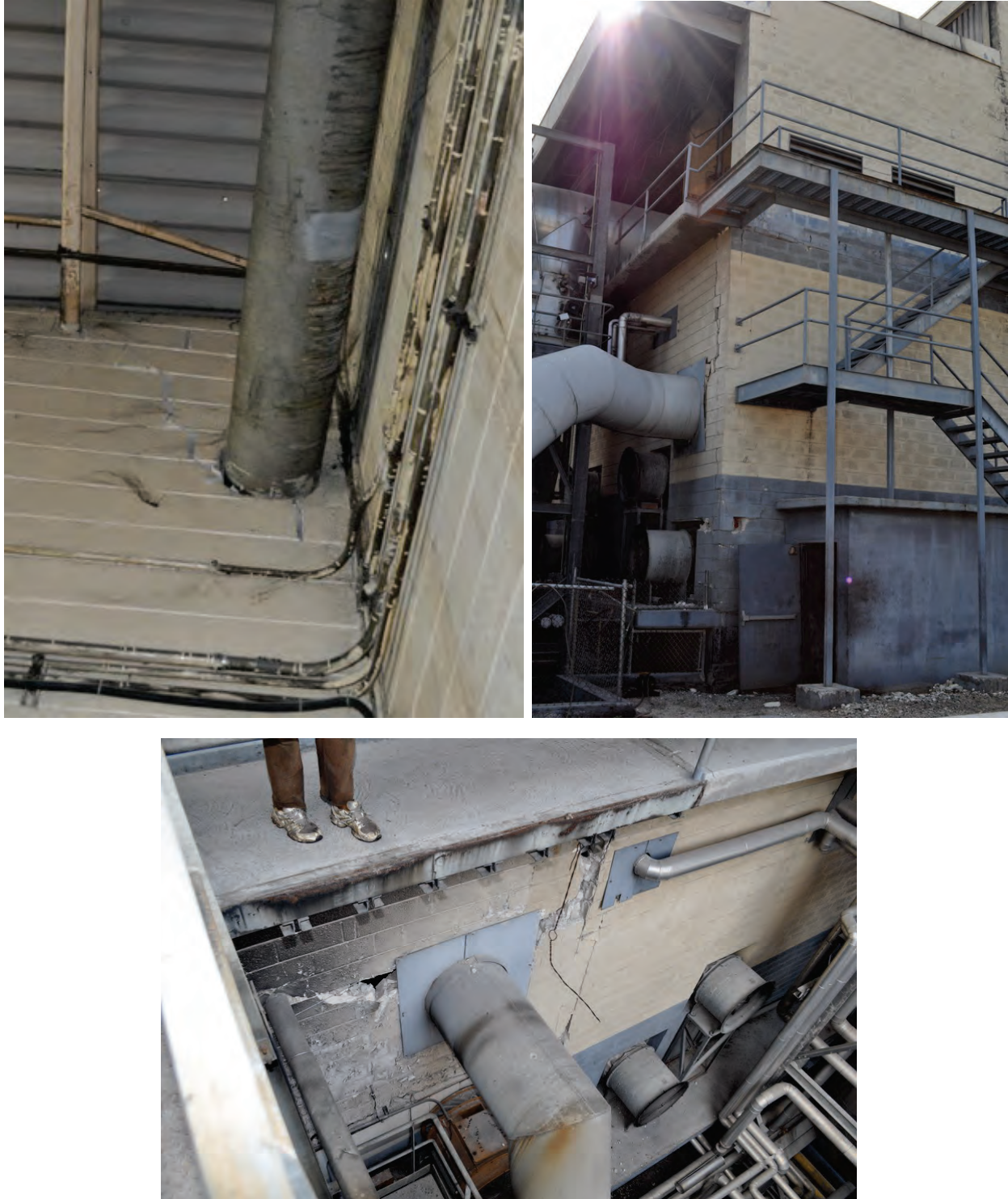
Figure 6.4.3.8-3 Wall penetrations for piping and ducts contributed to damage to unreinforced masonry walls at an industrial facility in the 2010 magnitude-7 Haiti Earthquake (Photos courtesy of Eduardo Fierro, BFP Engineers). The piping and ducts were not damaged but the walls cracked and will need to be repaired.
