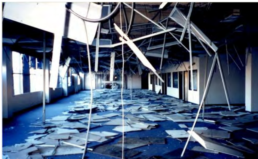
Figure 2.4.2-1 Complete loss of suspended ceilings and light fixtures in the 1994 Northridge Earthquake (FEMA 74, 1994).
