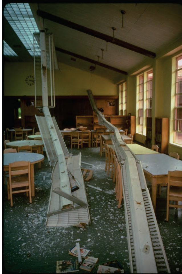
Figure 6.4.9.3-2 Failure of pendant light fixtures at Northridge Junior High School as a result of the 1994 Northridge Earthquake. In this example, the support stem failed at the fixture connection and the stem is still attached at the ceiling (Photo courtesy of Gary L. McGavin).
