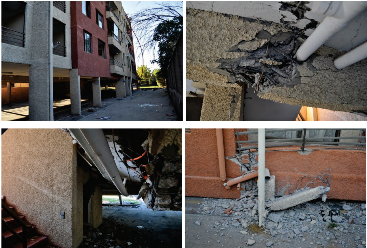
Figure 6.4.5.2-3 Photos displaying resilience of piping systems; this building suffered a partial structural collapse along one side in the 2010 Chile Earthquake. The only broken pipe (shown at lower right) was along the collapsed side; the other piping had broken pipe supports in some locations but the joints remained largely intact, even with these very large deformations (Photos courtesy of Eduardo Fierro, BFP Engineers).
