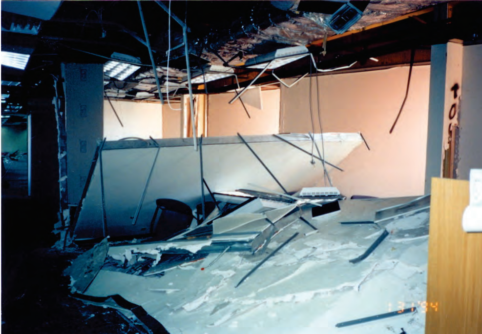
Figure 6.3.2.2-1 Out-of-plane failure of inadequately braced partial height metal stud partitions in the 1994 Northridge Earthquake (Photo courtesy of Wiss, Janney, Elstner Associates).
