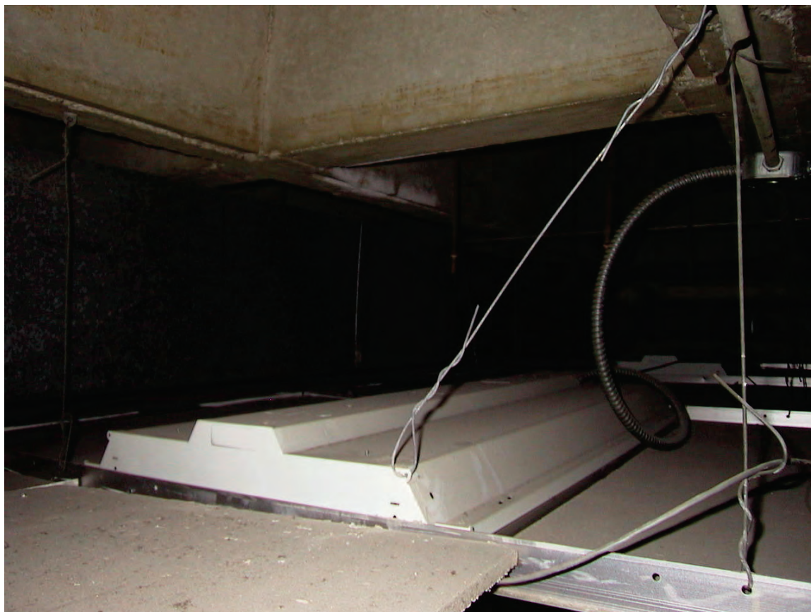
Figure 6.4.9.1-5 Example of light fixture with only one safety wire attached; the Salt Lake City schools require four wires for a fixture of this size and weight and also require tighter turns on the wire (Photo courtesy of Salt Lake City School District). Investigations in ceiling plenums often reveal missing wires.
