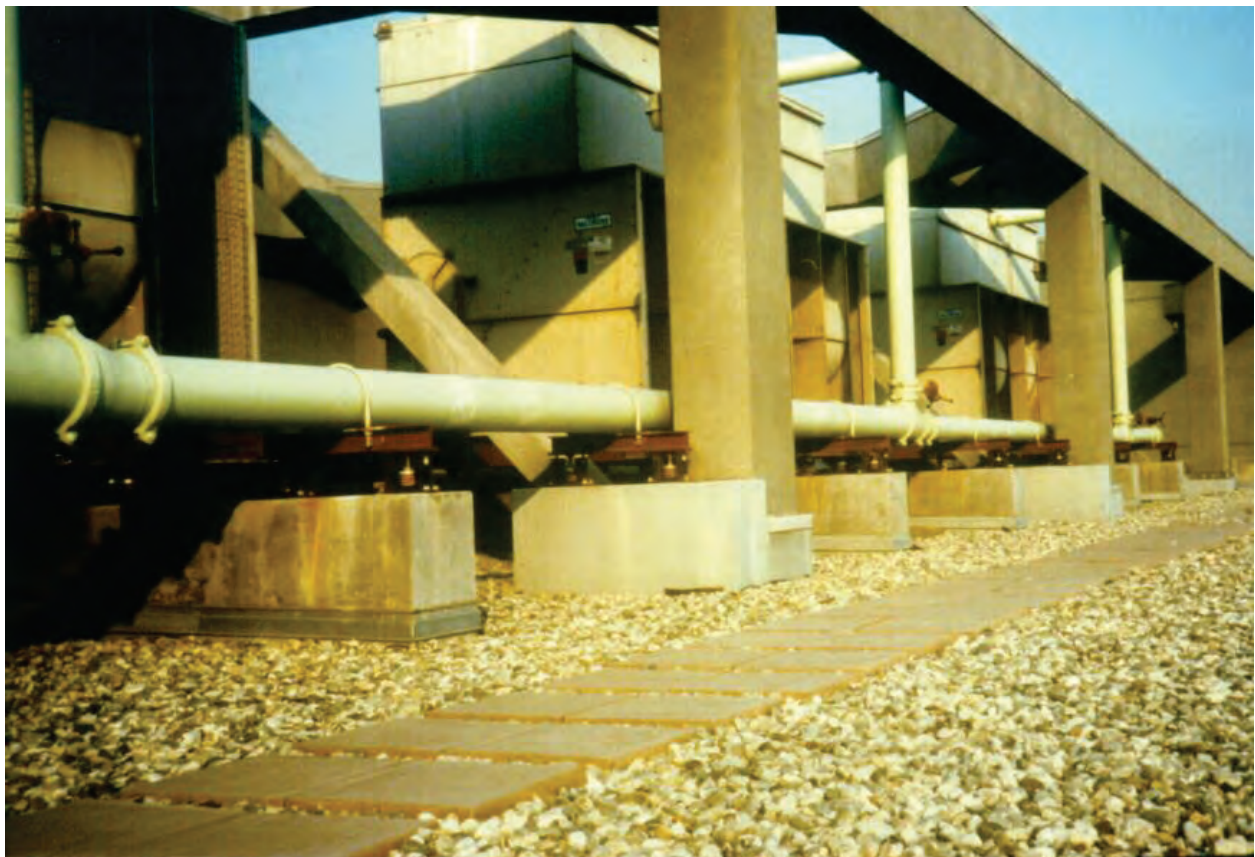
Figure 6.4.3.6-4 Roof-mounted supports with vibration isolation (Photo courtesy of Mason Industries).
