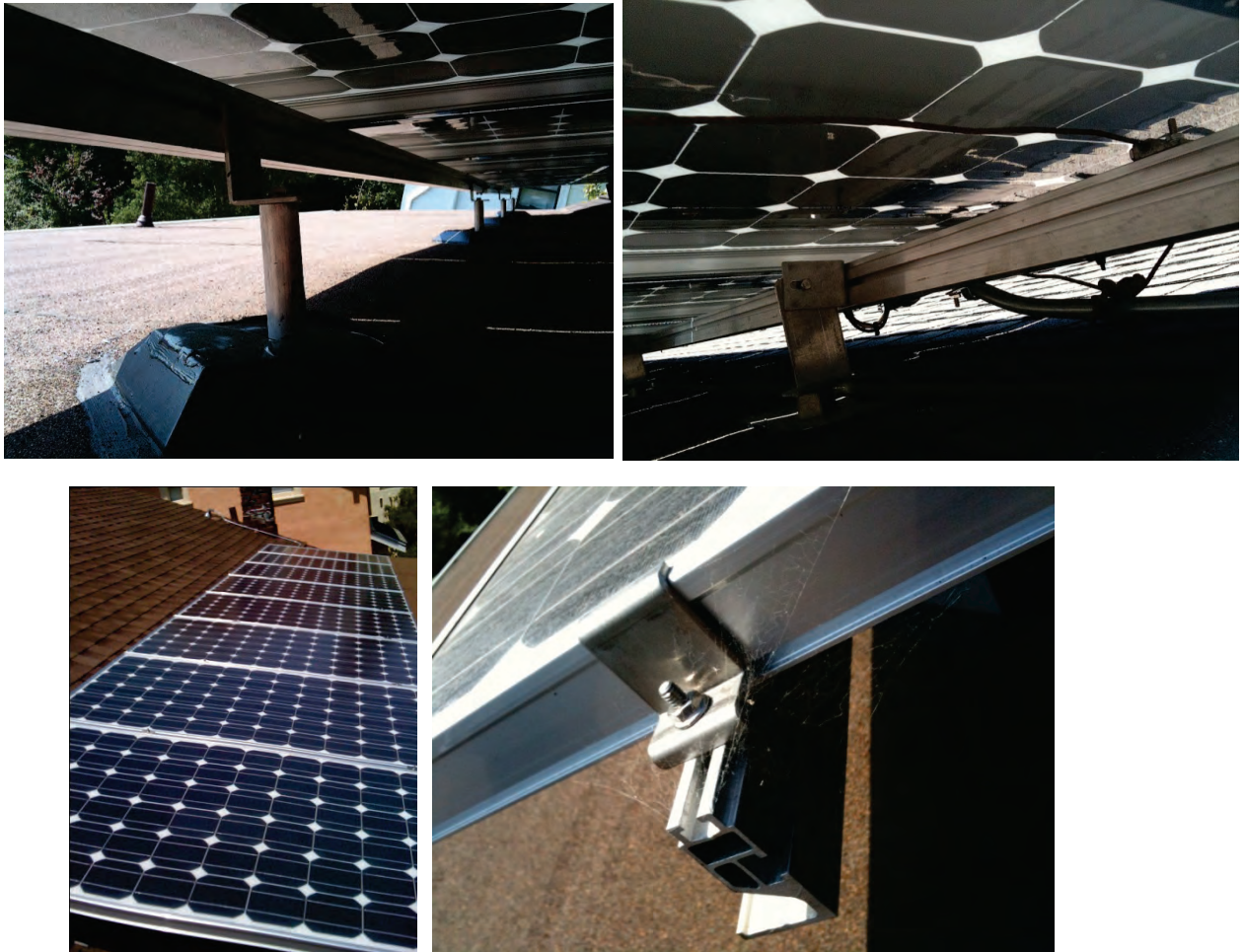
Figure 6.4.7.5-3 Residential photovoltaic system in Berkeley, California mounted over the transition between two different roof slopes (Photos courtesy of Heber Santos). Short standoff used on tar and gravel flat portion (upper left); aluminum flashing and mounting bracket used on sloped portion with composition tile roofing (upper right). The profile of one type of proprietary mounting track is seen at lower left.
