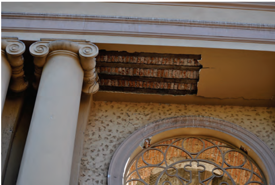
Figure 6.3.4.2-2 Damage to stucco soffit of historic church in the 2010 Chile Earthquake (Photo courtesy of Eduardo Fierro, BFP Engineers). Stucco applied directly to the underside of the slab above without furring; portion at left has fallen, portion at right delaminated.
