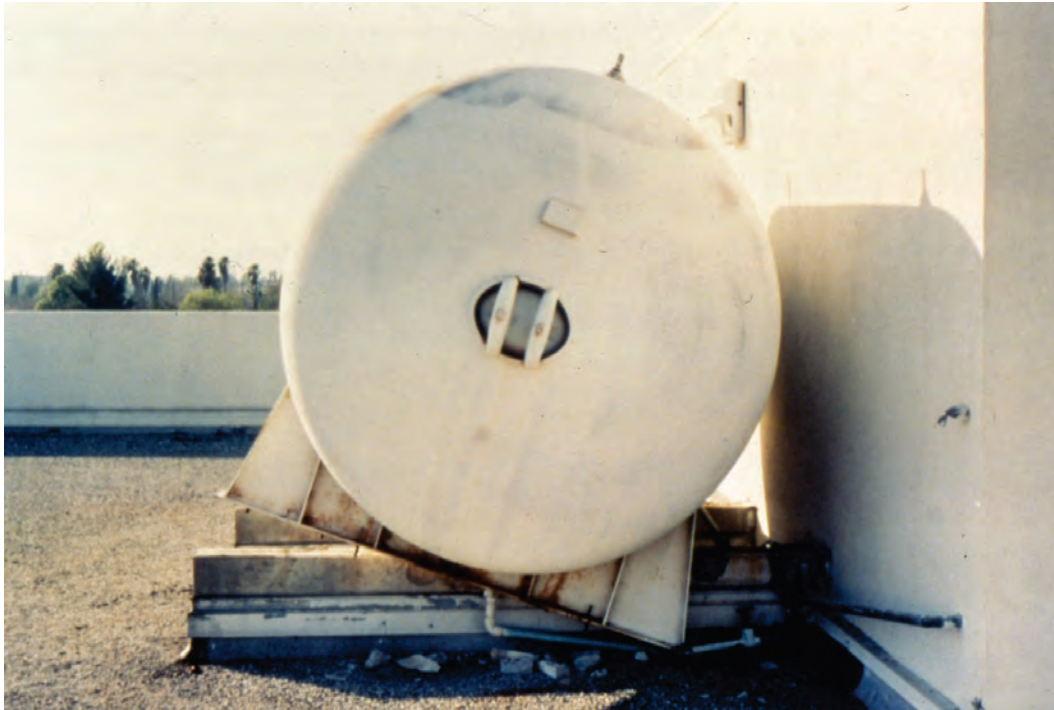
Figure 6.4.2.1-1 Tank shifted off support curb, Granada Hills Hospital in the 1994 magnitude-6.7 Northridge Earthquake (Photo courtesy of OSHPD).
