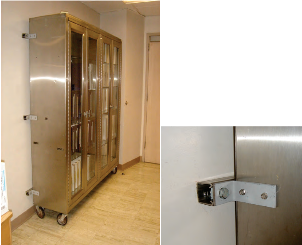
Figure 6.5.1.1-8 Mobile shelving unit restrained by connection to strut fastened to full height metal studs (Photo courtesy of Maryann Phipps, Estructure).
