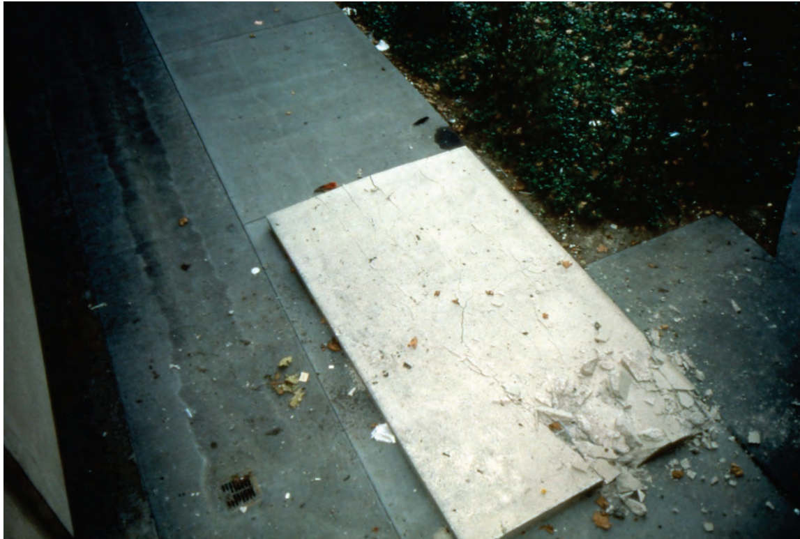
Figure 6.3.1.3-1 Failure of precast panel at parking garage that resulted in fatality in the 1987 magnitude-5.9 Whittier, California earthquake (Photo courtesy of Degenkolb Engineers).
