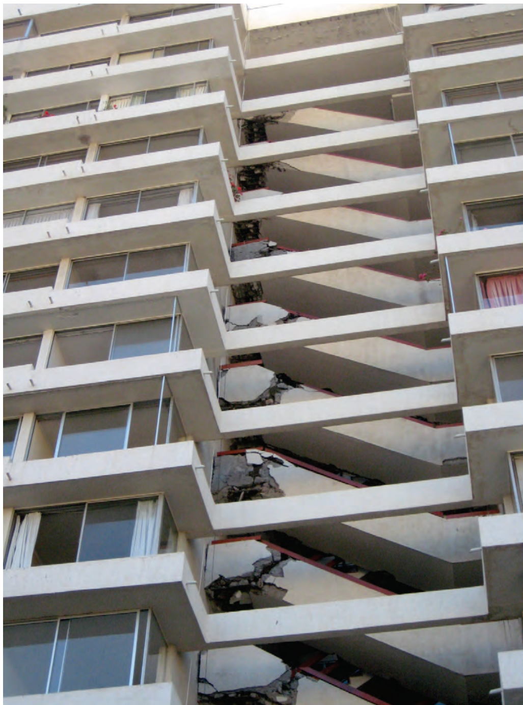
Figure 6.3.8.1-3 Stairs damaged up the full height of this apartment building in Viña del Mar in the 2010 magnitude-8.8 Chile Earthquake (Photo courtesy of Santiago Pujol, Purdue University). The stairs were rigidly attached at adjacent floors and behaved like diagonal braces although they were neither designed nor detailed to function as structural braces.
