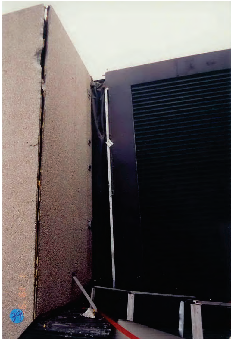
Figure 6.3.1.3-3 Precast panel damage at a building corner in the 1994 Northridge Earthquake (Photo courtesy of OSHPD).
