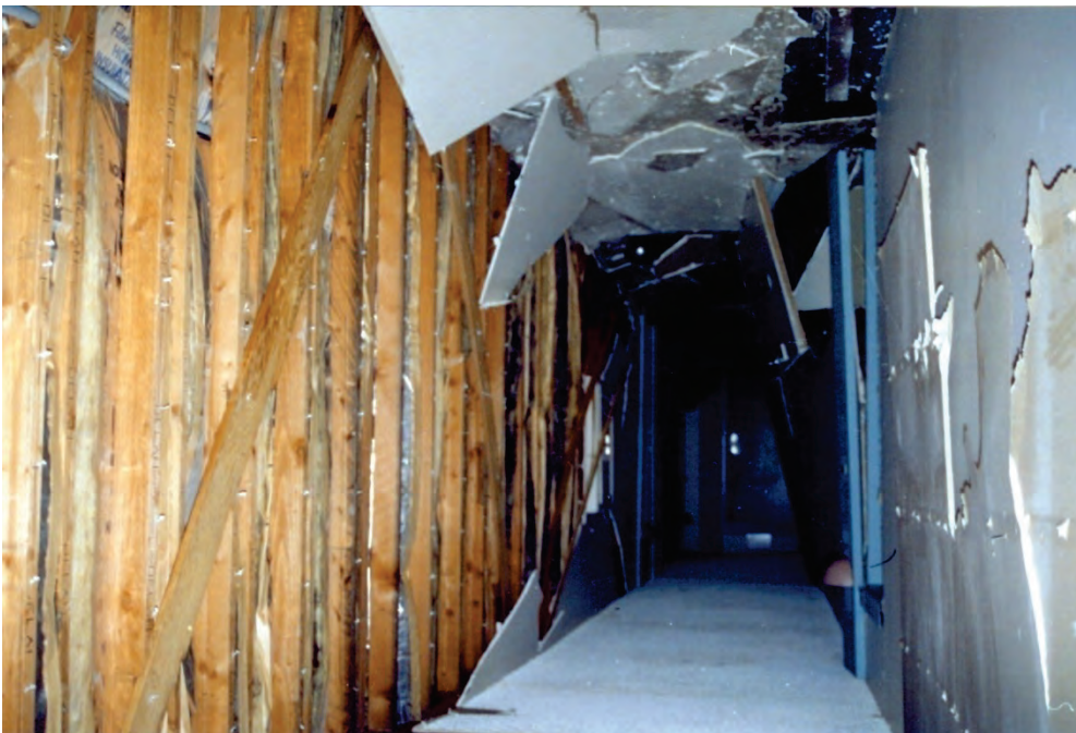
Figure 6.3.2.2-2 In-plane damage to wood stud wall spanning floor-to-floor caused by differential movement between the two floors in the 1994 Northridge Earthquake (Photo courtesy of Wiss, Janney, Elstner Associates).
