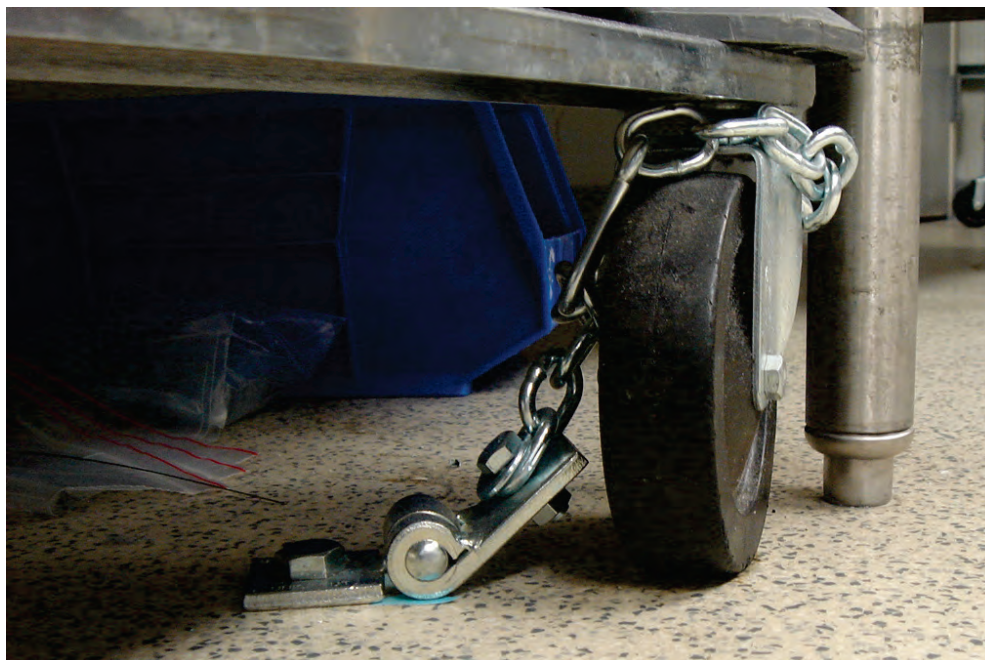
Figure 6.5.1.1-4 Alternate restraint at base of mobile shelving unit (Photo courtesy of Maryann Phipps, Estructure).
