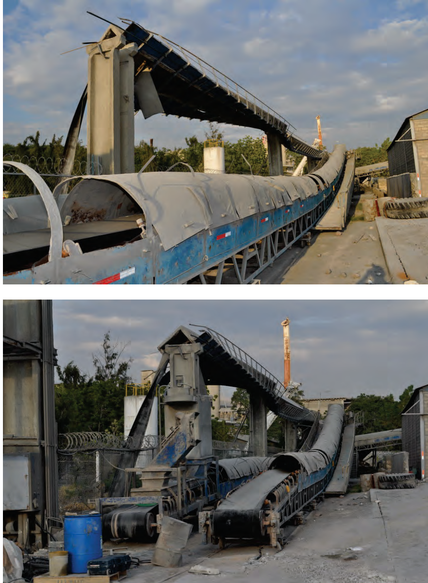
Figure 6.4.1.2-1 Damage to conveyors and equipment at a cement plant in the 2010 magnitude-7 Haiti Earthquake (Photos courtesy of Eduardo Fierro, BFP Engineers).
