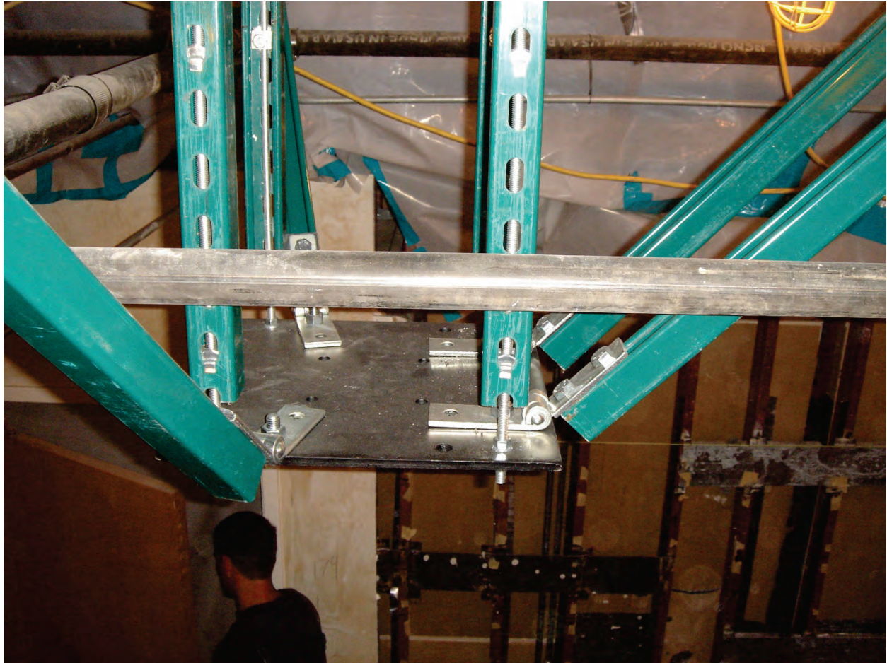
Figure 6.4.9.4-3 Engineered support and bracing for operating room lights located in California hospital. Steel plate has predrilled holes to receive fixture attachments (Photo courtesy of Maryann Phipps, Estructure).
