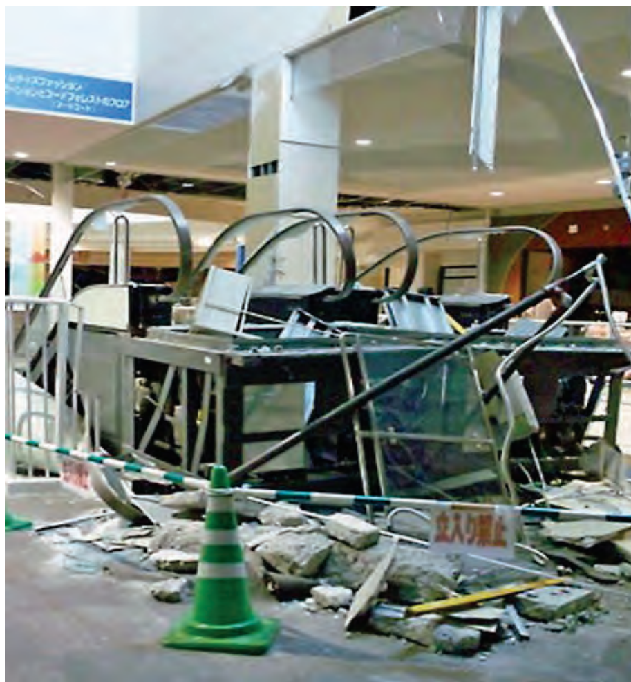
Figure 6.4.10.3-1 Photo of escalator, located in the Sendai area of Japan, which fell from the floor above onto the escalator on the floor below during the magnitude-9.0 Great Tohoku Earthquake of March 11, 2011. The probable cause of this collapse was that the relative displacements between floors exceeded the connection bearing width capacity of the escalator. This type of failure creates a serious life safety hazard (Photo source: Nekkei Architecture).
