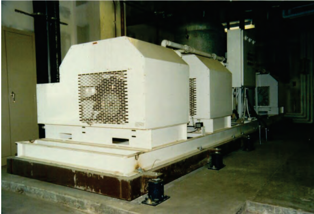
Figure 6.4.1.3-5 Restrainted springs used to support heavy equipment (Photo courtesy of Mason Industries).
