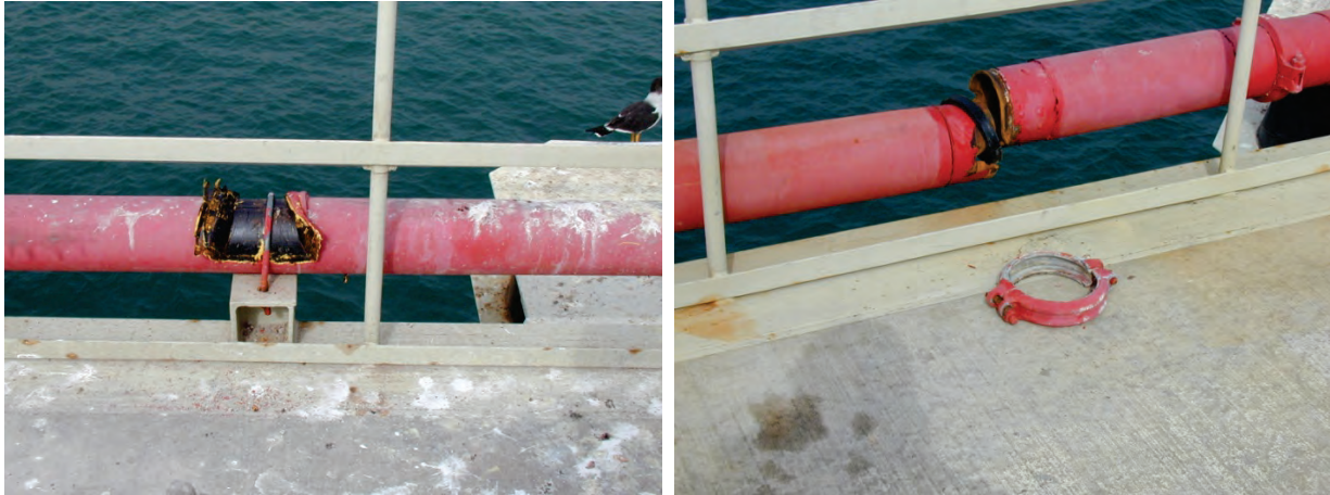
Figure 6.4.4.1-6 Damage to industrial fire protection piping located on jetty in 2001 Peru Earthquake. Longitudinal slip at U-bolt shown at left; this U-bolt still intact but other U-bolts broke and fell off the jetty. Failure of joint coupling and crushing of pipe shown at right (Photo courtesy Eduardo Fierro, BFP Engineers).
