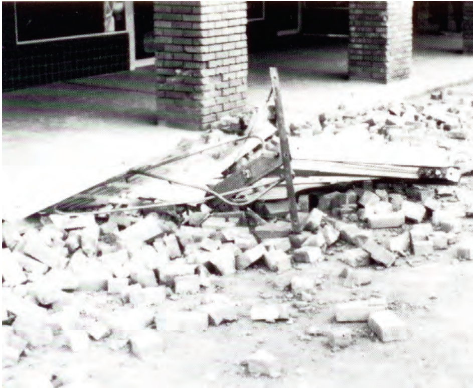
Figure 6.3.6.1-1 Failure of commercial sign in the 1979 Imperial Valley, California earthquake (Photo courtesy of Robert Reitherman).
