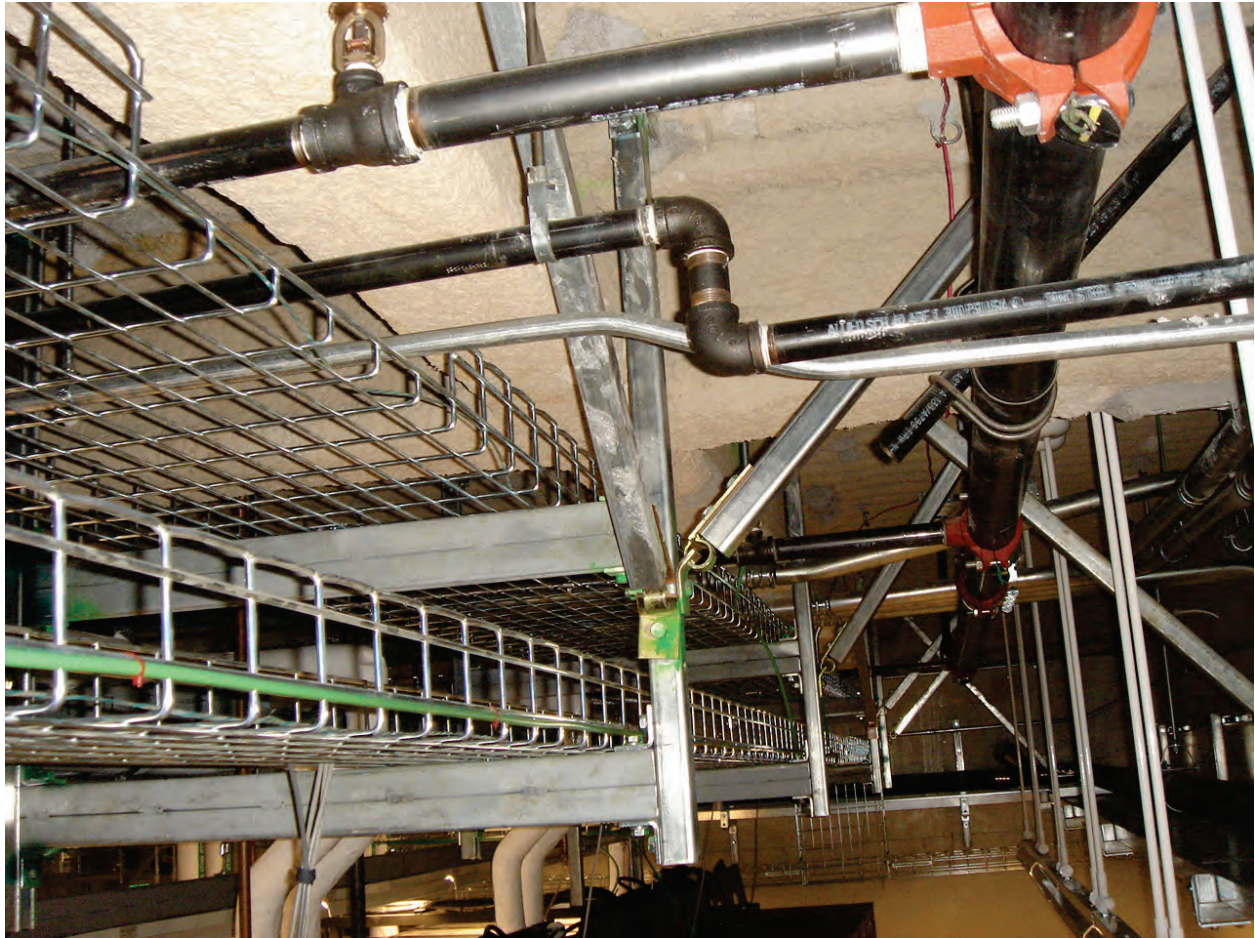
Figure 6.4.8.1-4 Lateral and longitudinal rigid strut bracing for trapeze supporting electrical raceways (Photo courtesy of Maryann Phipps, Estructure).
