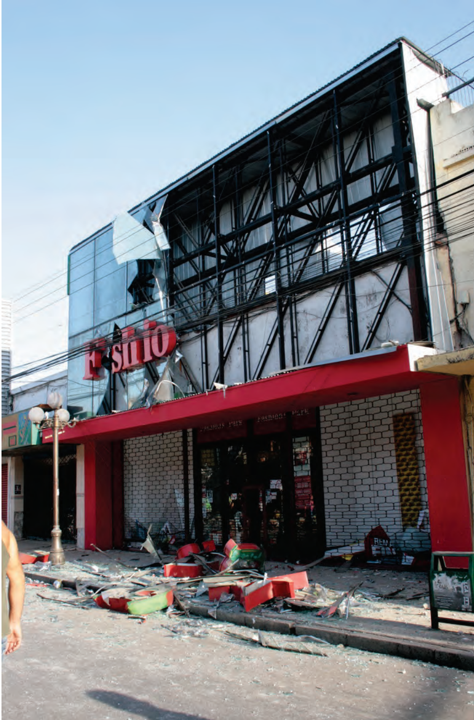
Figure 6.3.1.4-4 Glazing damage, due in part to pounding with the structure at right during the 2010 Chile Earthquake (Photo courtesy of Antonio Iruretagoyena, Rubén Boroscheck & Associates).
