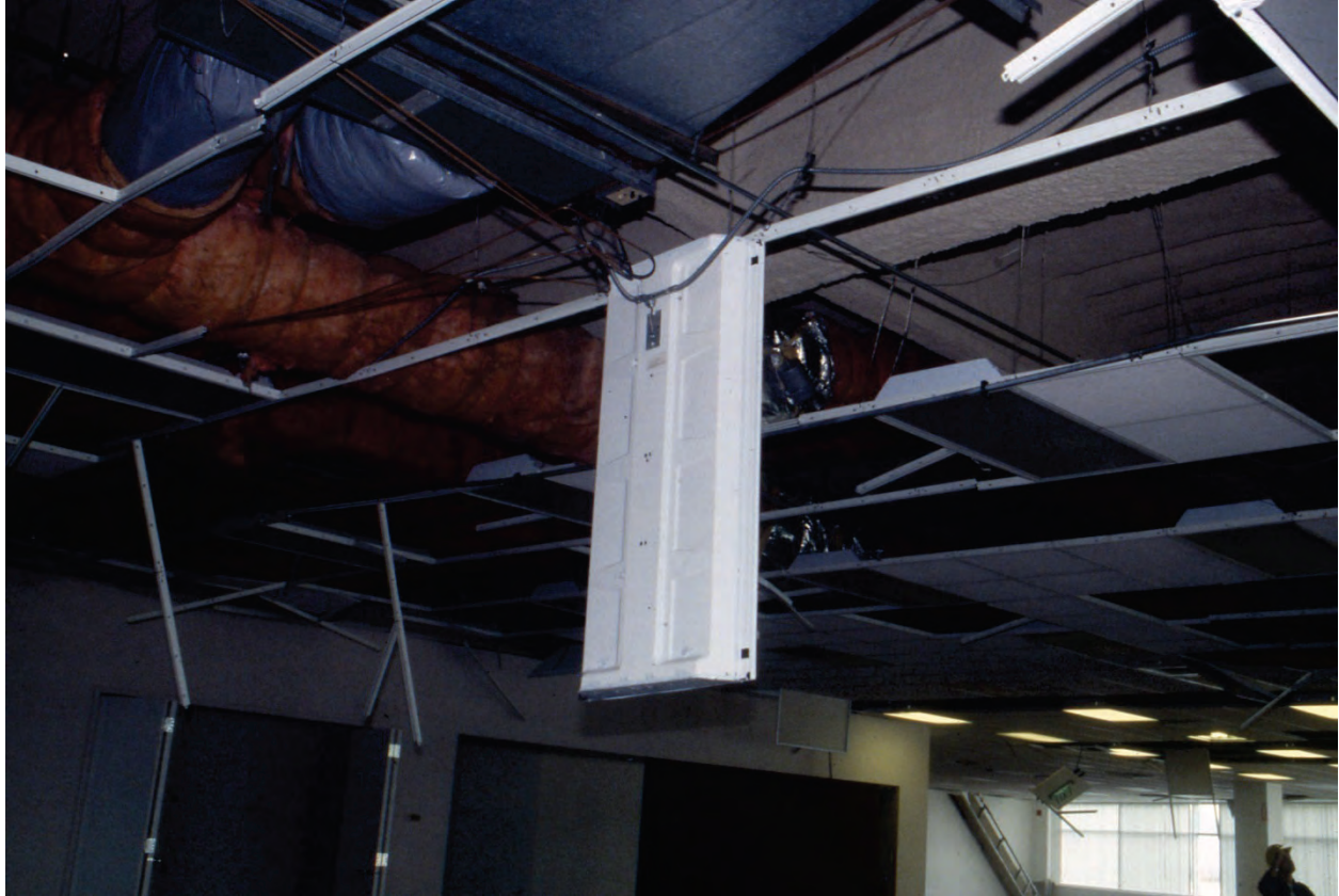
Figure 6.4.9.1-3 Light fixture without adequate independent support dangling along one edge from ceiling grid, damaged in the 1994 magnitude-6.7 Northridge Earthquake (Photo courtesy of Degenkolb Engineers).
