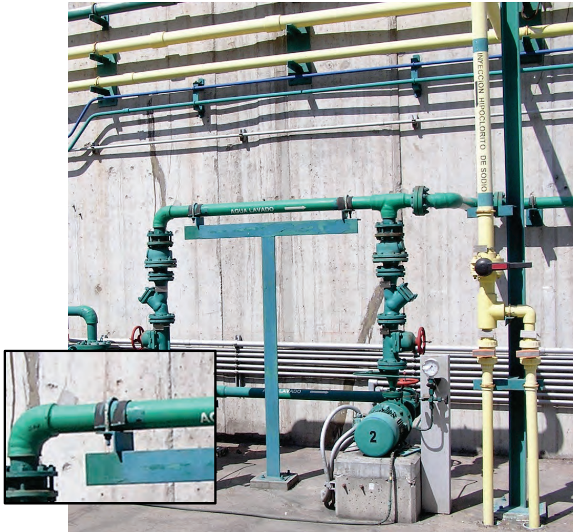
Figure 6.4.3.5-1 Pipe and support assembly seem intact but photo shows evidence of longitudinal movement of the pipe in the U-bolts (Photo courtesy of BFP Engineers). A rubber pad was installed between the U-bolt and pipe in order to increase the friction coefficient, but was not sufficient to provide longitudinal restraint.
