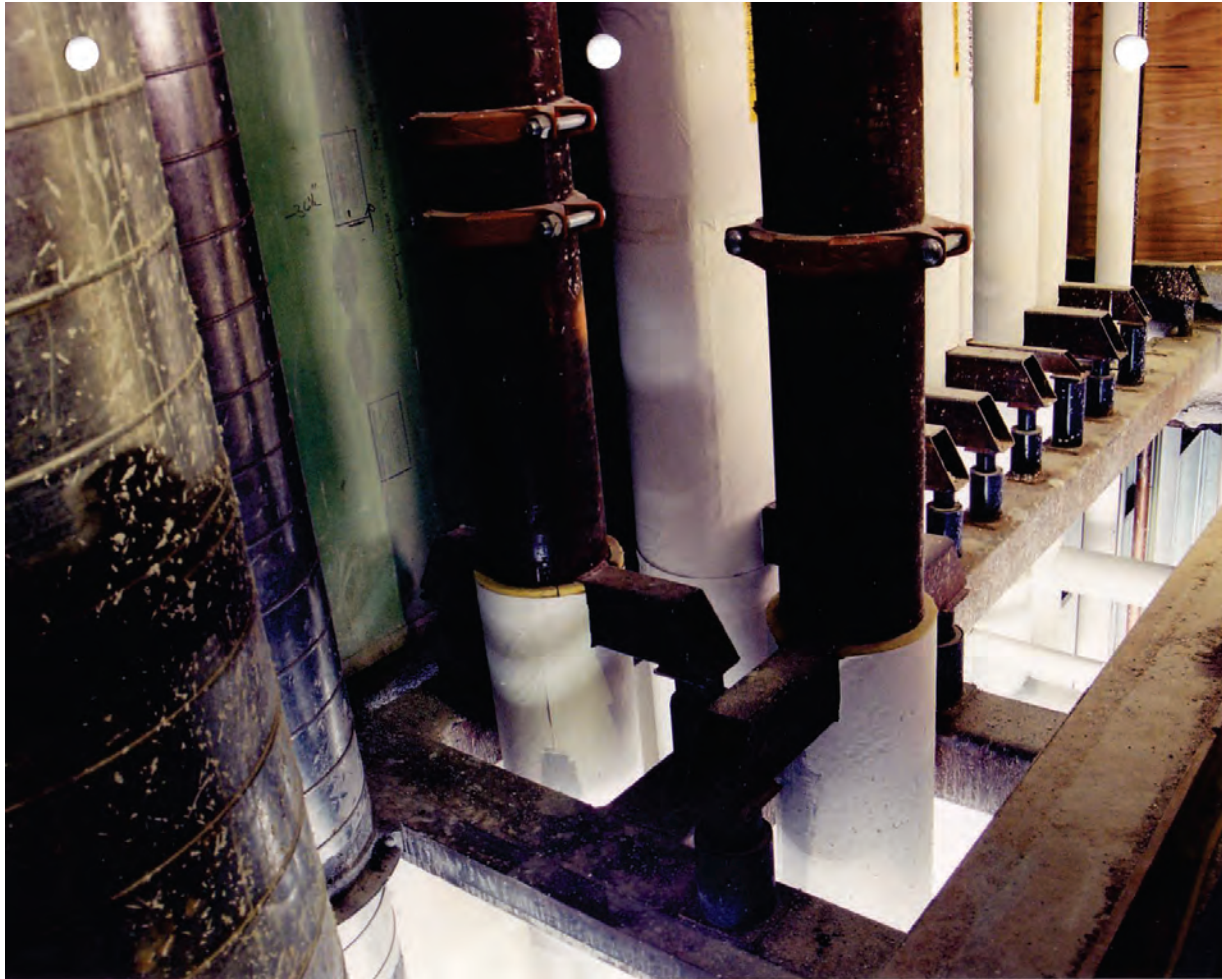
Figure 6.4.3.4-2 Riser supports provide lateral restraint with vertical sliding guides that allow thermal movement; restraint hardware consisting of tube sections is welded to either side of pipe (Photo courtesy of Mason Industries).
