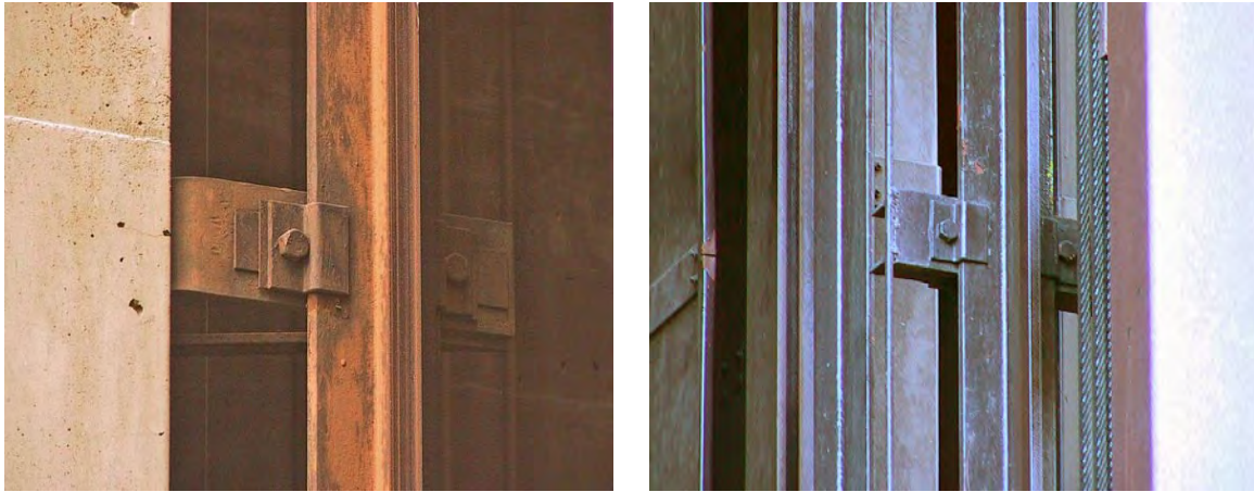
Figure 6.4.10.2-2 Examples of brackets and clips attaching the elevator guide rails to the structure (Photo courtesy of Eduardo Miranda, Stanford University).
