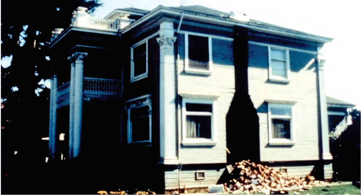
Figure 6.3.7.1-3 Chimney collapse (Photo courtesy of Earthquake Engineering Research Institute).
