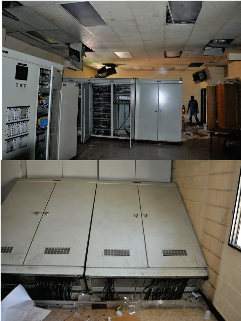
Figure 6.4.7.1-3 Damage to unanchored electrical cabinets at power plant in Port-au-Prince in the 2010 magnitude-7 Haiti Earthquake (Photos courtesy of Eduardo Fierro, BFP Engineers).
