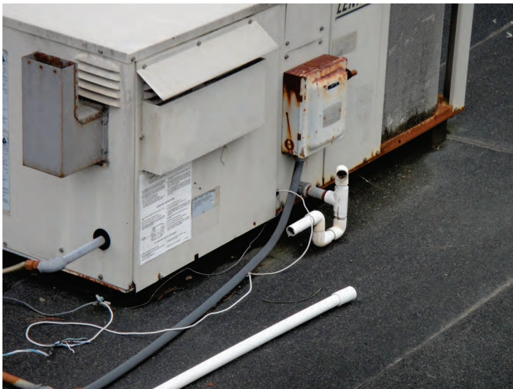
Figure 6.4.3.6-3 Unrestrained roof-mounted piping broke at the connection to the equipment in the 2010 Eureka Earthquake. Piping mounted on wood sleepers should typically be restrained to the roof, not free to slide (Photo courtesy of Maryann Phipps, Estructure).
