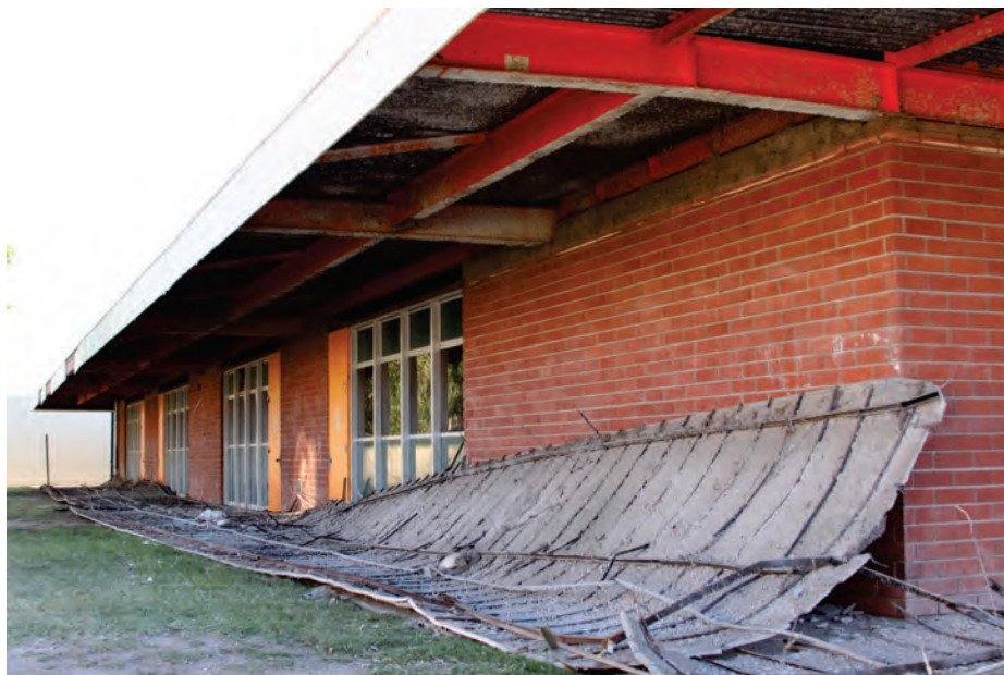
Figure 6.3.4.3-3 Collapse of exterior soffit at Jefferson Elementary School in Calexico in the 2010 Baja California Earthquake; approximately 1200 sq ft of soffit collapsed at this school built in the 1960's (Photo courtesy of Baja Earthquake Reconnaissance Team, Earthquake Engineering Research Institute (EERI), published in the EERI July 2010 Newsletter).
