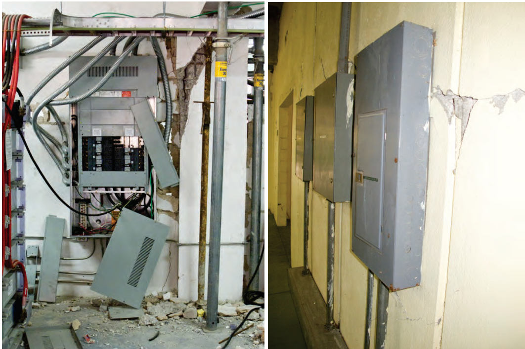
Figure 6.4.7.3-8 Example of rugged equipment. Post earthquake photos of two different essential facilities which sustained significant structural damage during the 2010 M 7.0 Haiti Earthquake. Wall mounted electrical power distribution panels were undamaged and remained functional even though the walls they were mounted to were severely damaged during the earthquake (photos courtesy of Philip J. Caldwell).
