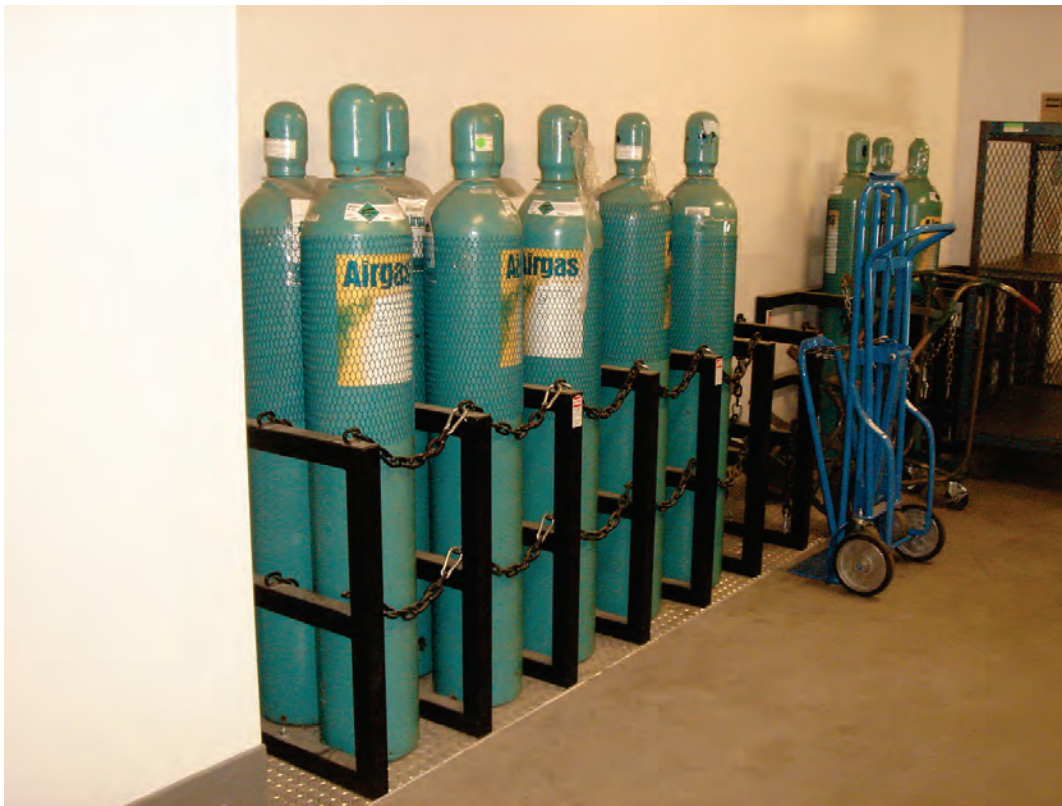
Figure 6.4.2.3-7 Detail of enclosures for air gas tanks in a hospital; chains attached with quick release hooks (Photo courtesy of Maryann Phipps, Estructure).
