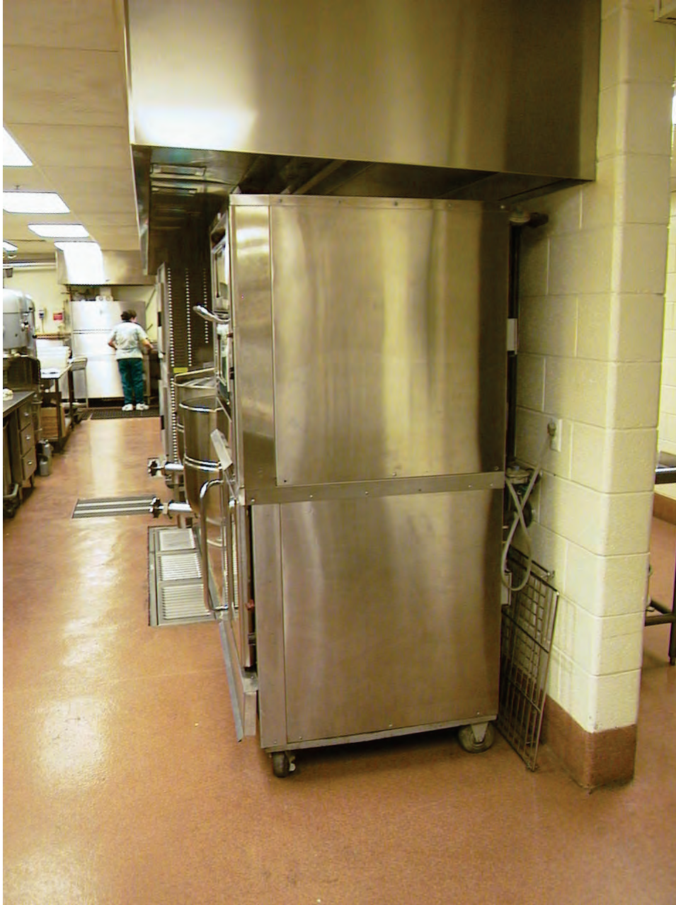
Figure 6.5.5.3-2 Existing condition: Unrestrained kitchen equipment (Photo courtesy of EQE for the Salt Lake City School District).
