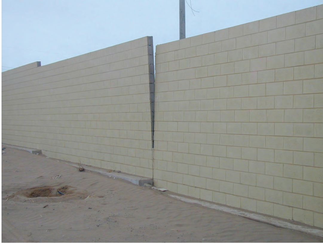
Figure 6.3.9.1-3 Damage to reinforced masonry boundary fence at industrial facility in Southern Peru; out-of-plane movement at construction joint in wall without sufficient reinforcing for the level of shaking experienced at this location in the 2001 magnitude-8.4 Peru Earthquake (Photo courtesy of Eduardo Fierro, BFP Engineers). Additional boundary steel or reinforced concrete boundary columns located either side of construction joints would improve the performance of this type of fence.
