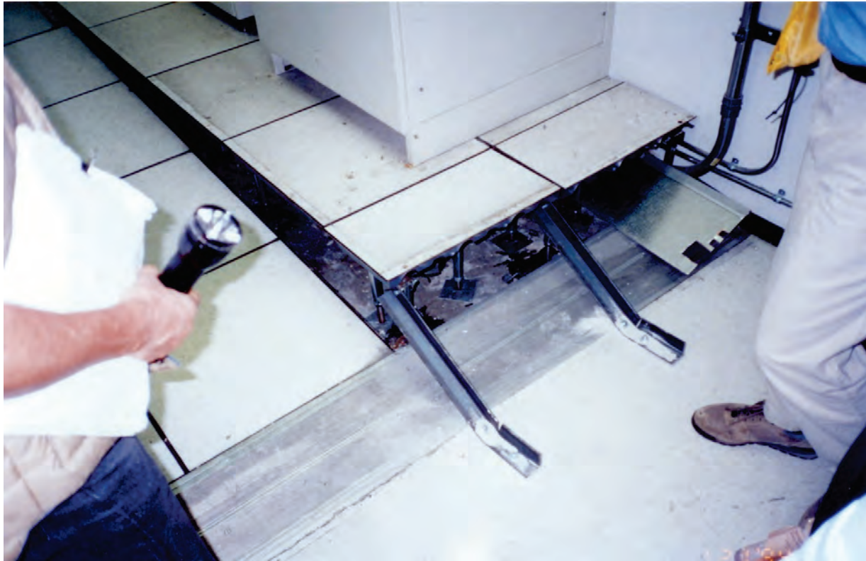
Figure 6.5.3.1-1 Temporary bracing for access floor collapsed in the 1994 magnitude-6.7 Northridge Earthquake (Photo courtesy of Wiss, Janney, Elstner Associates).
