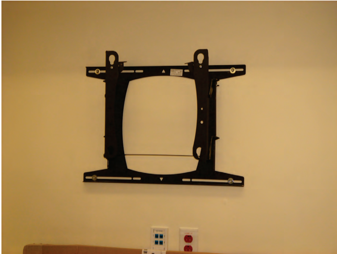
Figure 6.5.3.4-2 Wall-mounted television bracket anchored with sheet metal screws to wall studs at four locations. Bracket must be rated for the weight of television or monitor and that the unit must be securely attached to the bracket (Photo courtesy of Maryann Phipps, Estructure).
