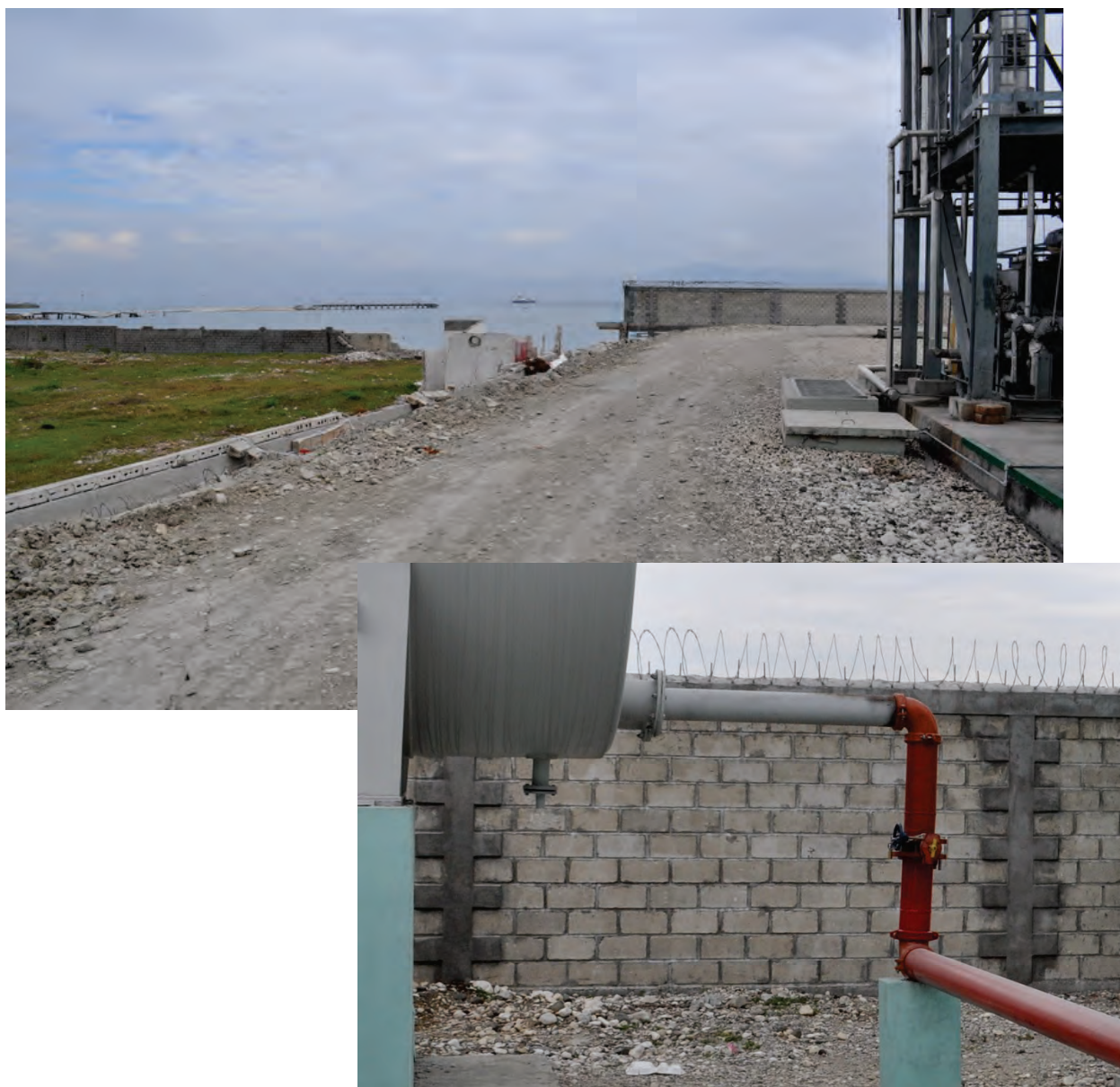
Figure 6.3.9.1-4 Photo at top shows complete collapse of poorly detailed confined masonry fence in foreground; partial collapse of poorly detailed confined masonry fence in distance at left; no damage to well detailed confined masonry fence in distance at right in the 2010 Haiti Earthquake. Close-up view of well-detailed confined masonry fence in bottom photo with concrete columns and bond beam at top (Photos courtesy of Eduardo Fierro, BFP Engineers). Fences in foreground and at right formed the security perimeter at an electric power plant in Port-au-Prince.
