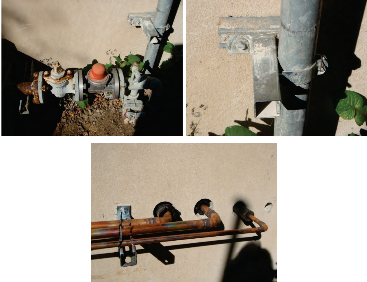
Figure 6.4.3.7-3 Wall-mounted pipe restraint examples using standard strut shapes and connectors (Photo courtesy of Cynthia Perry, BFP Engineers). Bottom view still under construction; pipes temporarily attached with plastic ties.
