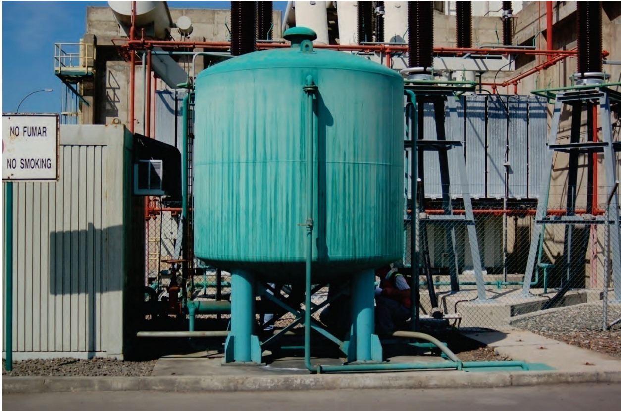
Figure 6.4.2.1-7 Gusset plates and cross bracing added at base of vertical tank on four legs following the 2001 magnitude-8.4 Peru Earthquake (Photo courtesy of Eduardo Fierro, BFP Engineers).
