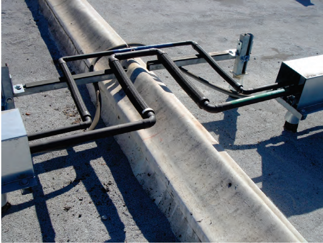
Figure 6.4.3.3-4 Flexible pipe connections at rooftop expansion joint (Photo courtesy of Maryann Phipps, Estructure).
