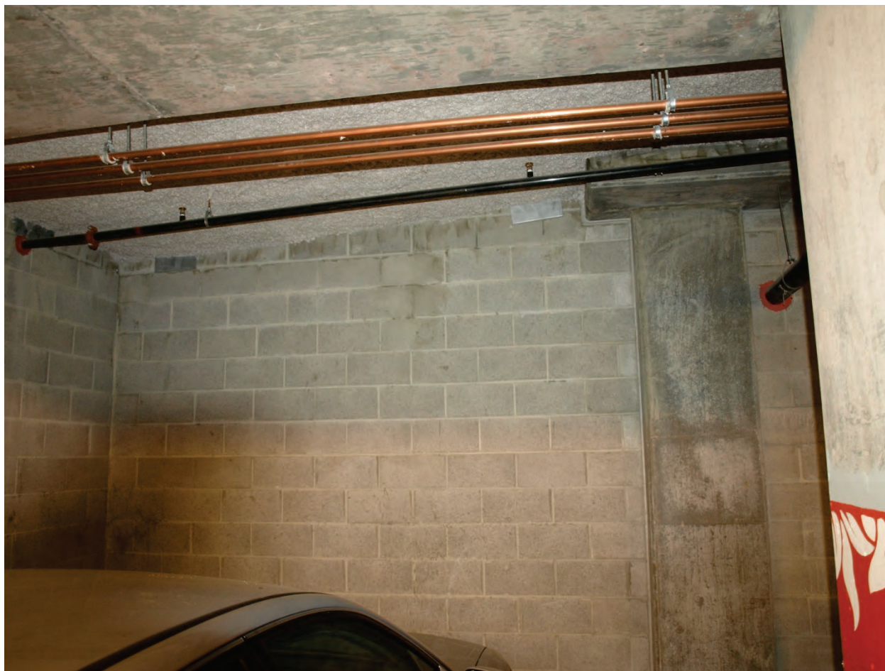
Figure 6.3.2.1-8 Full-height concrete masonry unit walls detailed with steel clip angles (3 angles visible in photo). Configuration shown includes perpendicular walls, sloping ramp above, and column with column capital. Although wall detailed with sealant joints along edges of column and column capital, it is not clear that the concrete frame can move independently of these CMU walls (Photo courtesy of Cynthia Perry, BFP Engineers).
