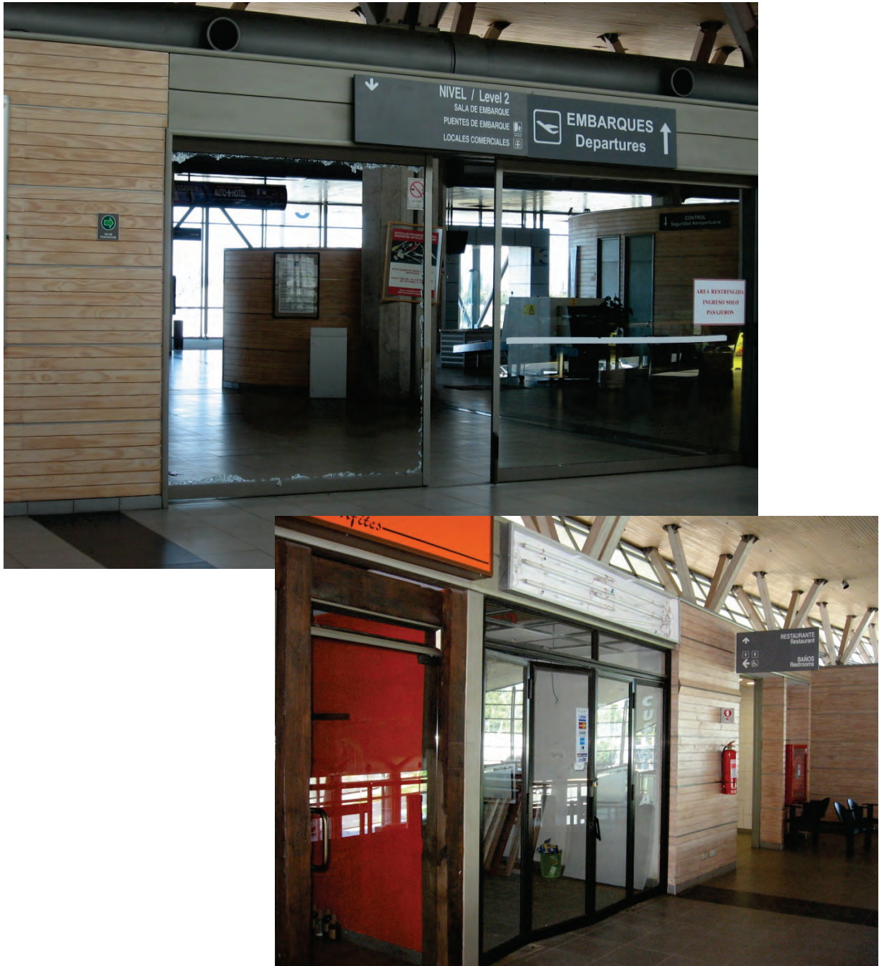
Figure 6.3.2.3-2 Damage to glazed doors at the Concepción airport in the 2010 Chile Earthquake. In the top photo the glazing in the sliding glass door shattered; in the lower photo the glass is intact but the door frames are misaligned (Photos courtesy of Rodrigo Retamales, Rubén Boroschek & Associates).
