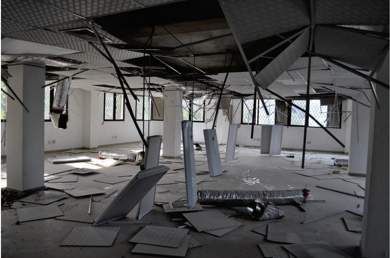
Figure 6.4.9.1-1 Numerous fluorescent fixtures dangling from electrical conduit; installed without safety wires in unbraced suspended acoustical ceiling and damaged in the 2010 magnitude-7 Haiti Earthquake. Loose bulbs, lenses, ceiling panels, diffusers and ducts also on the floor (Photo courtesy of Ayhan Irfanoglu, Purdue University).
