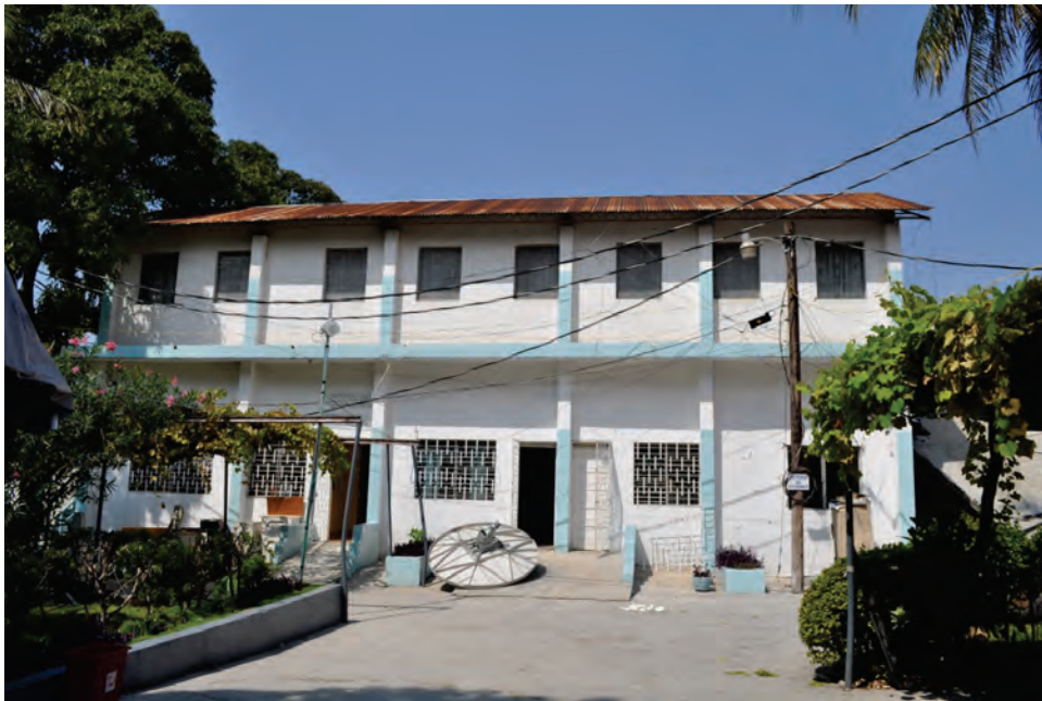
Figure 6.4.7.6-2 Antennae retrieved from roof of adjacent collapsed wing of the Hôpital Saint-François de Sales in the 2010 magnitude-7 Haiti Earthquake (not known if antenna suffered earthquake damage; photo courtesy of Ayhan Irfanoglu, Purdue University). Hospital communications depend on the functionality of antennae such as this.
