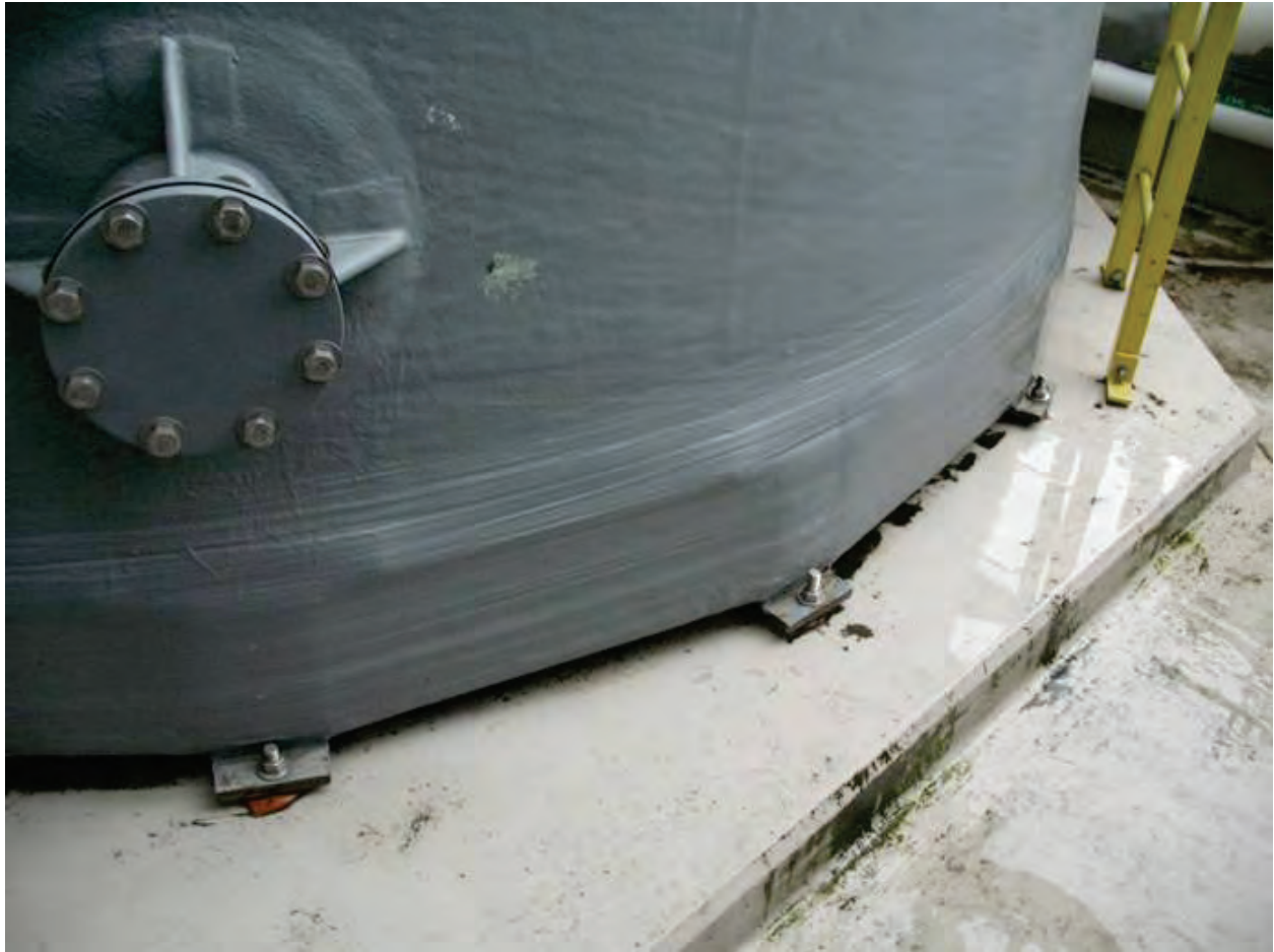
Figure 6.4.2.2-6 Anchors at base of fiberglass reinforced plastic tank (Photo courtesy of Jeffrey Soulages, Intel).
