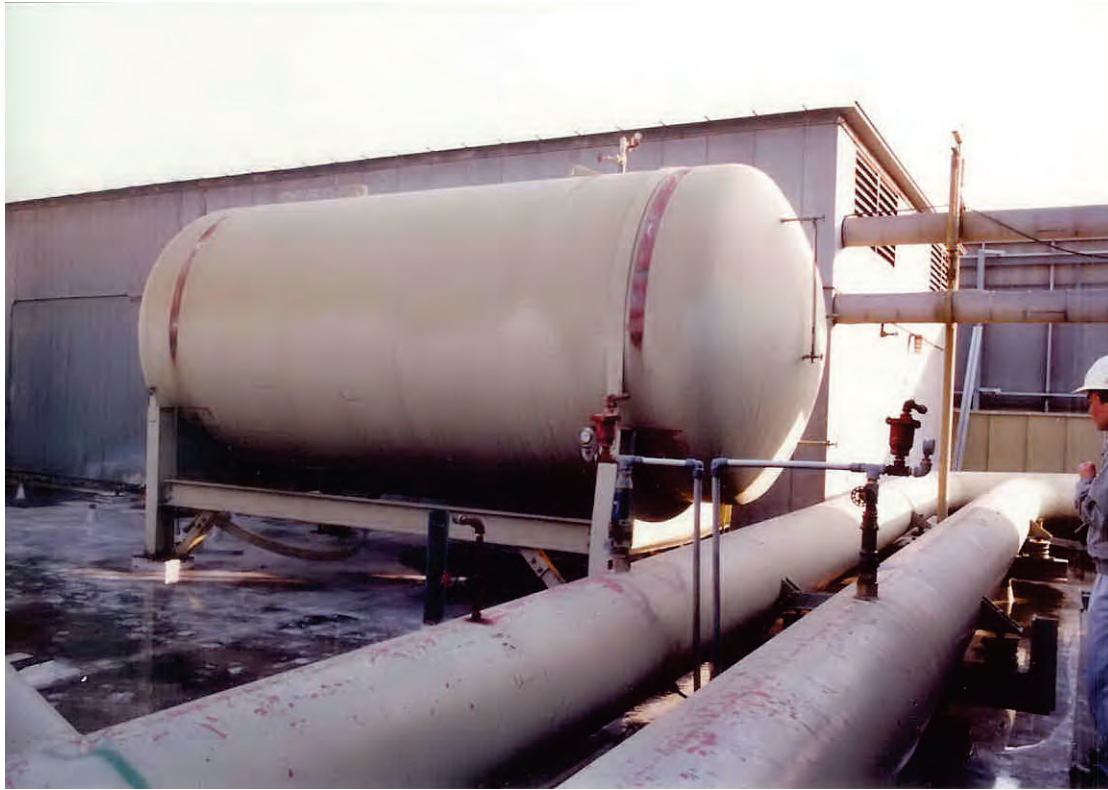
Figure 6.4.2.1-3 Horizontal tank strapped to structural support frame on hospital roof; one strap failed and tank slid six inches in the 1994 Northridge Earthquake (Photo courtesy of OSHPD).
