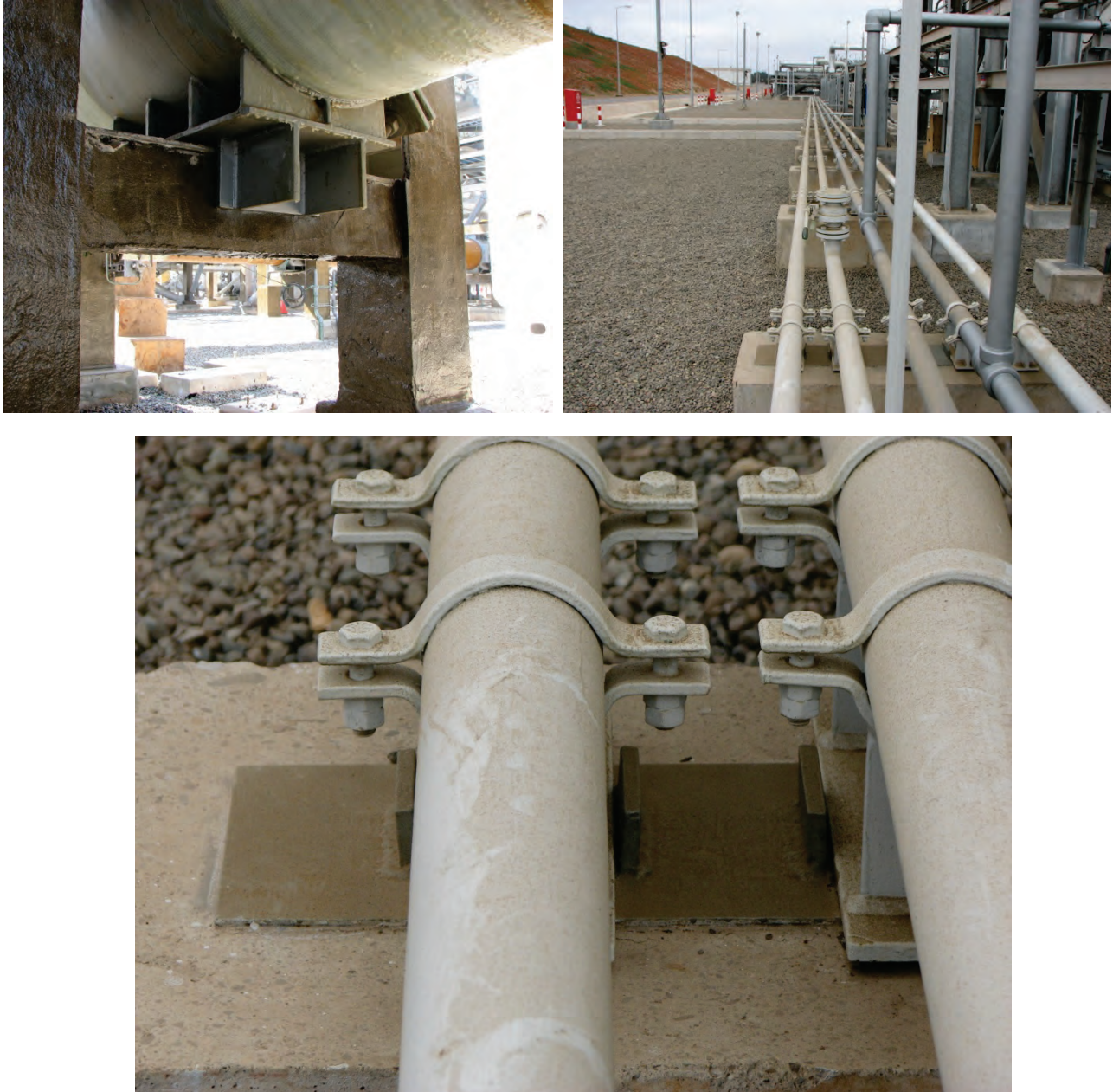
Figure 6.4.3.5-5 Floor-mounted supports for industrial piping in Chile; piping undamaged in the 2010 Chile Earthquake. The Chilean Industrial Code (Norma Chilena 2369) requires that shear forces be resisted by shear keys as shown; lower photo is detail of piping at upper right (Photos courtesy of Antonio Iruetagoiena, Rubén Boroschek & Associates).
