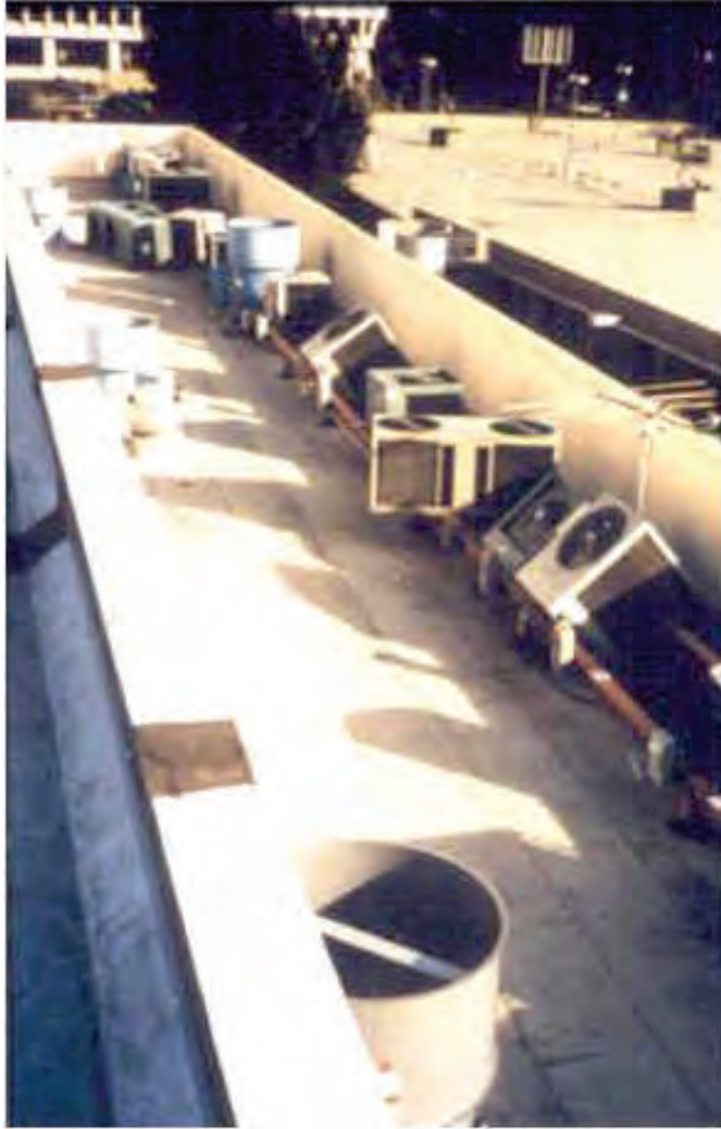
Figure 6.4.1.4-2 Unanchored rooftop units thrown off their supports during an earthquake (Photo courtesy of Maryann Phipps, Estructure).
