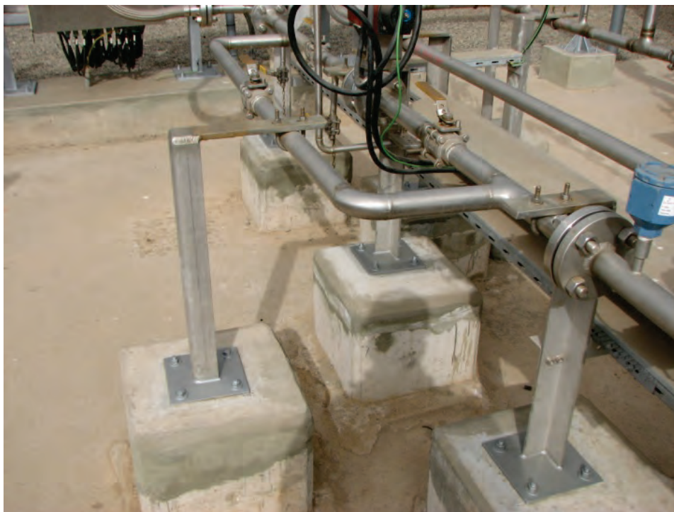
Figure 6.4.3.5-4 Floor/ground-mounted supports for industrial piping in Chile; piping undamaged in the 2010 magnitude-8.8 Chile Earthquake. Pipe supports include concrete pedestal, base plate, and built-up welded support stand. (Photos courtesy of Antonio Iruretagoyena, Rubén Boroschek & Associates).
