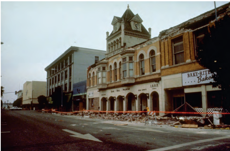
Figure 6.3.5.1-2 Unreinforced masonry parapet failures along Beach Street, Watsonville in the 1989 magnitude-6.9 Loma Prieta Earthquake (NGDC, 2009).
