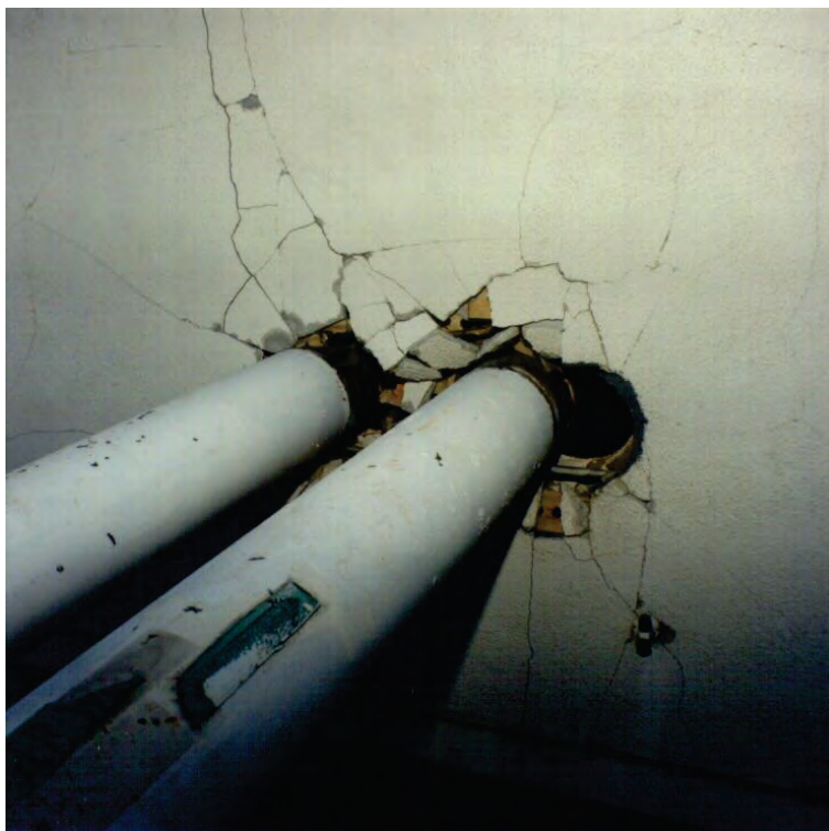
Figure 6.4.3.5-2 Damage to piping, stud wall and finishes due to movement of poorly restrained floor-mounted piping in the 1994 magnitude-6.7 Northridge Earthquake (Photo courtesy of Mason Industries).
