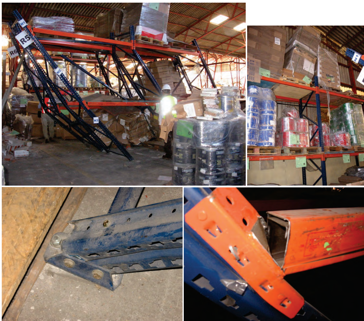
Figure 6.5.1.2-4 Failure of anchored racks in the 2010 magnitude-8.8 Chile Earthquake. The racks are leaning precariously due to inadequate bracing in the longitudinal direction and weak connections between the components. The welded fitting at the end of the beam failed at the weld in many places. Note that most items were shrink wrapped so merchandise did not scatter (Photos courtesy of Rodrigo Retamales, Rubén Boroschek & Associates).
