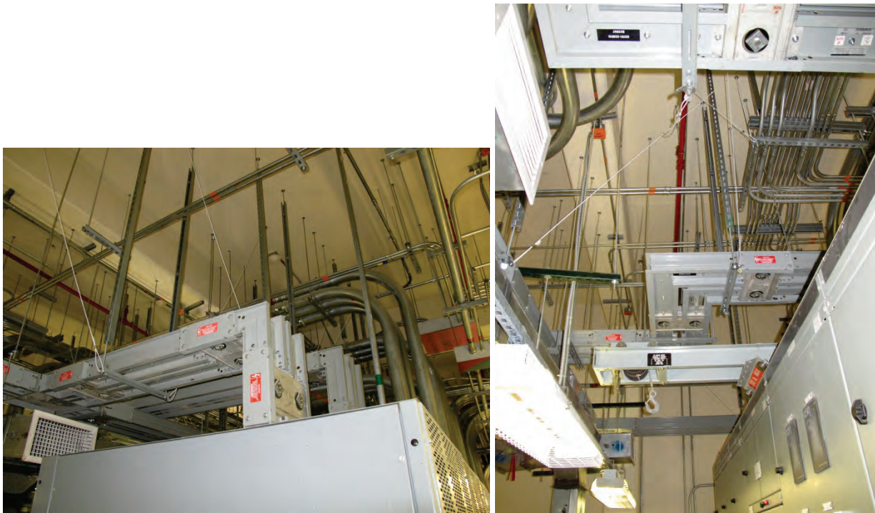
Figure 6.4.7.3-3 High ampacity power busway routing power from generator paralleling switchgear to facility. Note use of lateral restraints in addition to gravity hanger. Supplied uninterrupted power to critical facility during the 2010 M 7.0 Haiti earthquake. (photos courtesy of Philip J. Caldwell)
