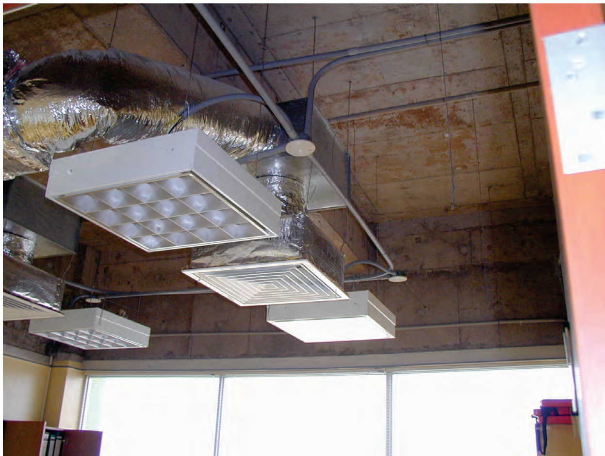
Figure 6.4.6.2-2 HVAC diffuser attached to the structure with four vertical hangers; ceiling system was damaged beyond repair in the 2001 Peru Earthquake but none of the diffusers or lights fell. Ceiling was demolished prior to photo (Photo courtesy of Eduardo Fierro, BFP Engineers).
