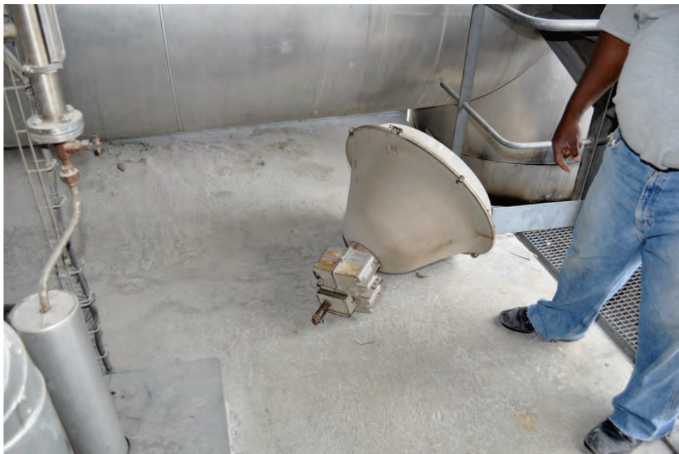
Figure 6.4.9.3-3 Failure of pendant light fixture in the 2010 magnitude-7 Haiti Earthquake; stem of fixture broke and conduit pulled loose (Photos courtesy of Eduardo Fierro, BFP Engineers).
