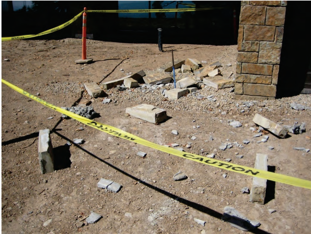
Figure 6.3.1.2-2 Fallen sandstone veneer as a result of a magnitude-4.4 earthquake (Photo courtesy of Simpson Gumpertz and Heger).
