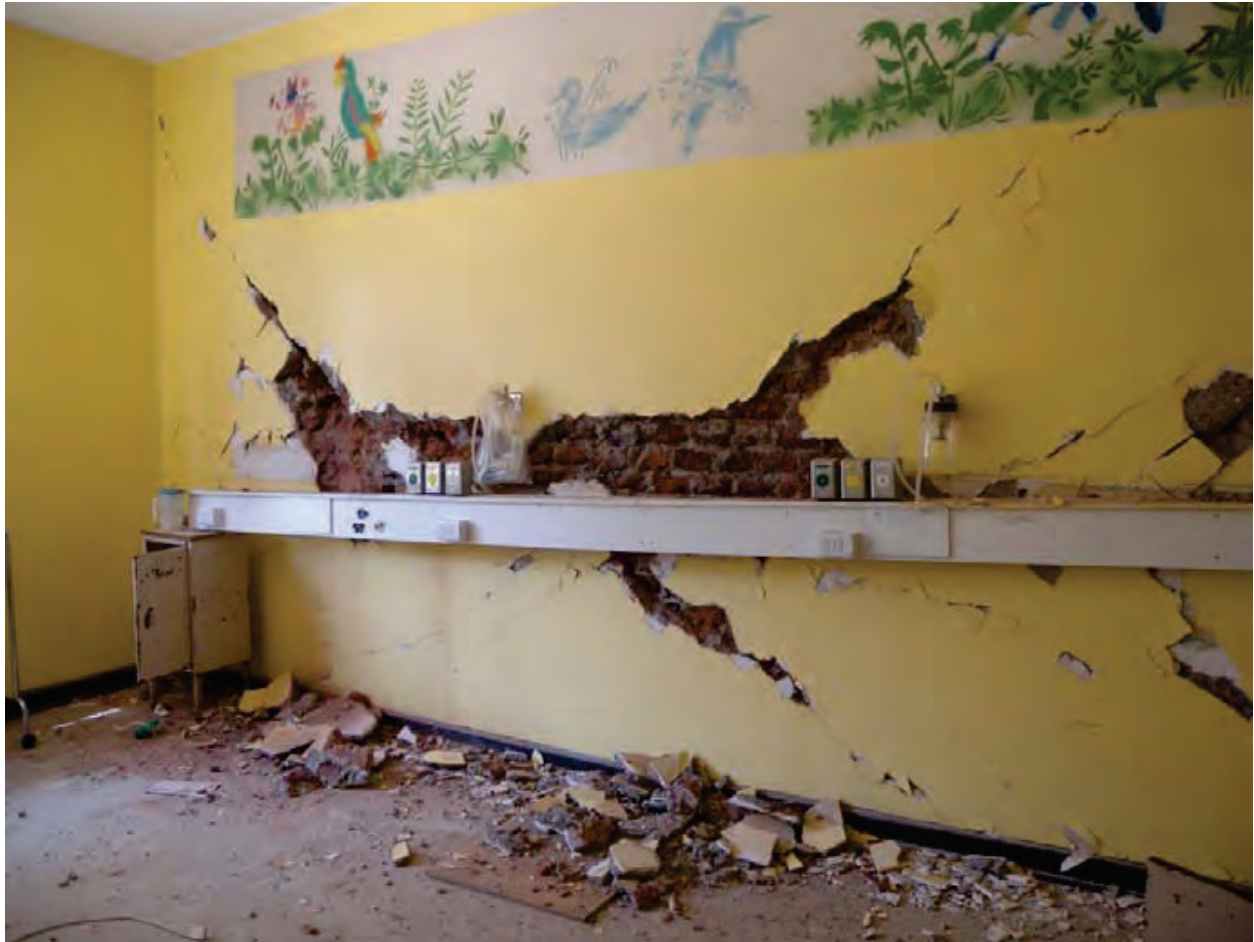
Figure 6.3.2.1-5 Damage to unreinforced brick partitions in patient rooms, and other mostly nonstructural damage, resulted in the evacuation of the Felix Bulnes Hospital in Santiago in the 2010 magnitude-8.8 Chile Earthquake (Photo courtesy of Gilberto Mosqueda, University of Buffalo, SUNY).
