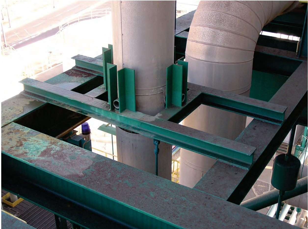
Figure 6.4.3.4-4 Insulated boiler pipe risers with welded lugs (small pipe sections) which travel vertically in guides providing lateral seismic restraint (Photo courtesy of Eduardo Fierro, BFP Engineers).
