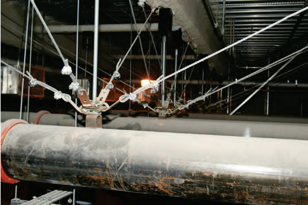
Figure 6.4.3.1-6 All-directional cable bracing of suspended piping (Photo courtesy of ISAT).
