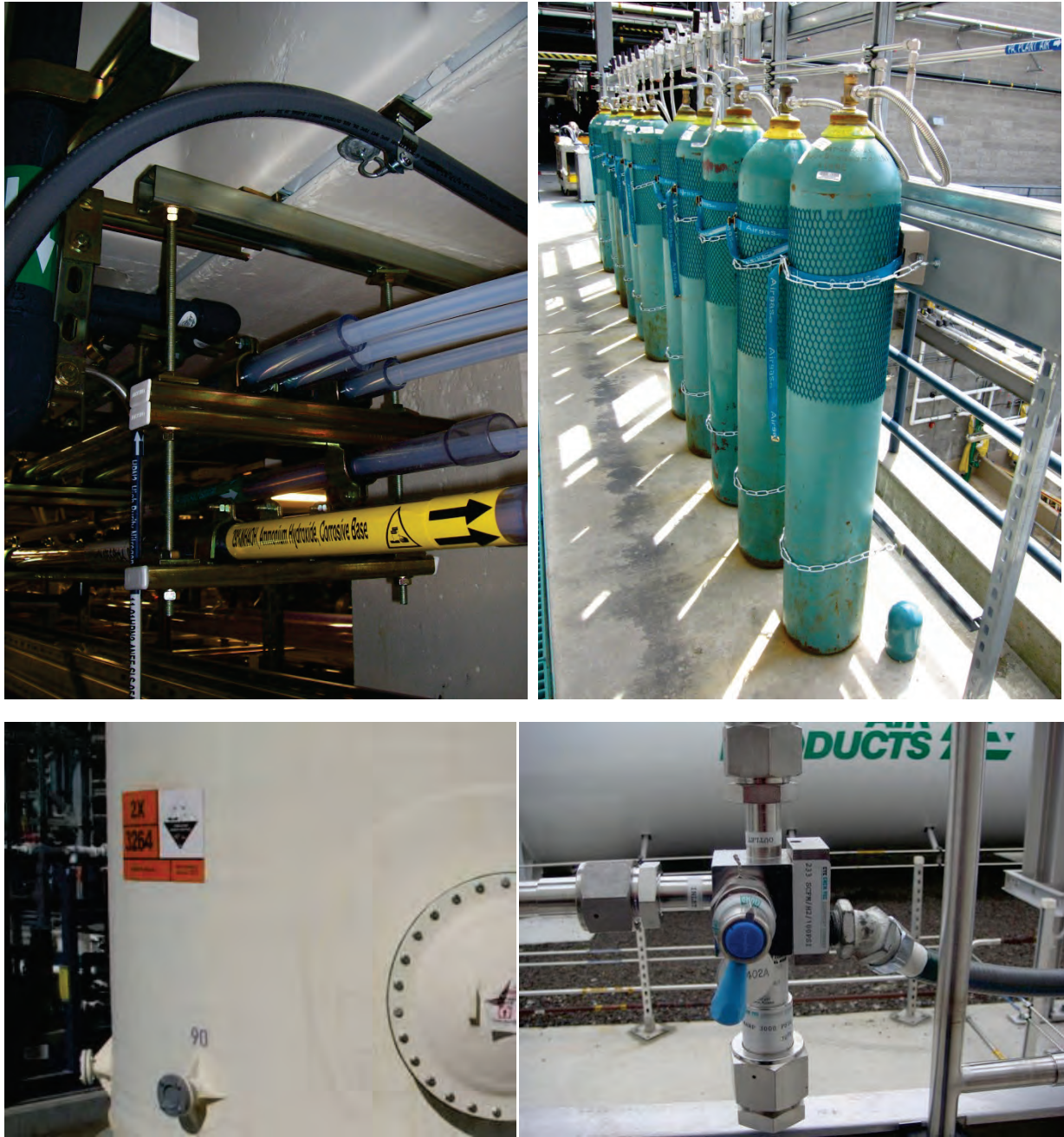
Figure 6.4.5.1-6 Clockwise from top: a) Sleeved pipe connections where seismic anchorage consists of cushioned pipe clamp attached around outer sleeve and inner pipe not restrained longitudinally. b) Airgas canisters chained and strapped to supports, fitted with flexible hose, stainless steel piping (note blue label), and a row of valves. c) Label on tank shows example of European ADR danger labeling scheme. d) Excess flow valve for large gas tank (Photos courtesy of Jeffrey Soulages, Intel Corporation).
