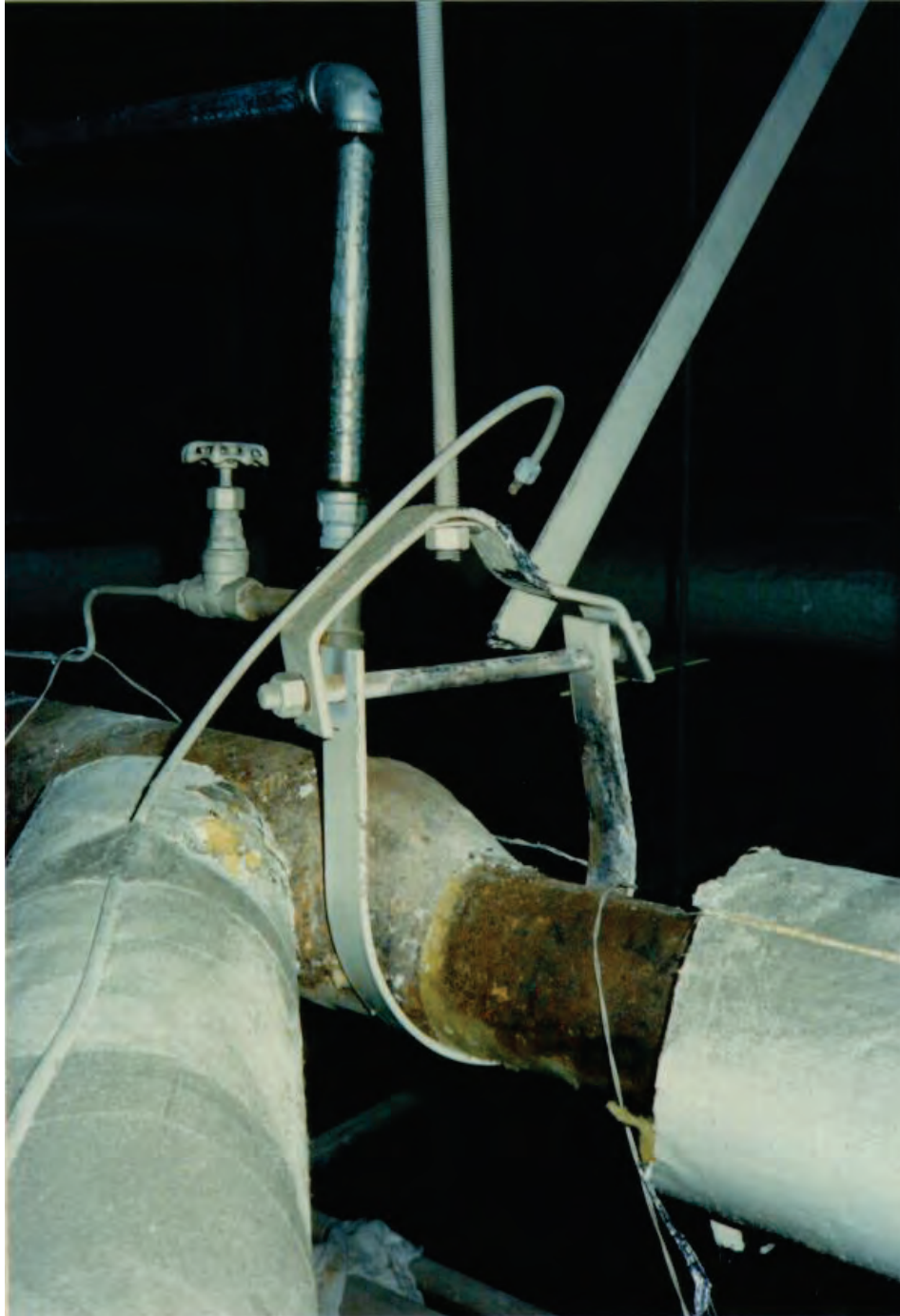
Figure 6.4.3.1-3 Pipe brace failed at connection in 1994 Northridge Earthquake; insulation removed prior to photo (Photo courtesy of Mason Industries).
