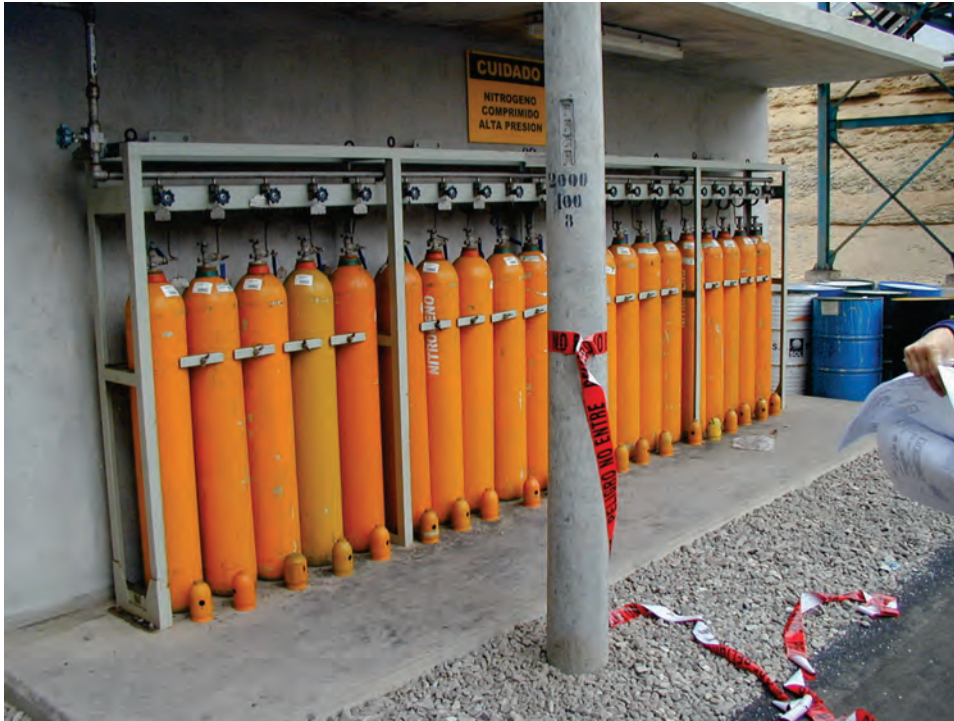
Figure 6.4.2.3-2 Gas cylinder anchorage with attached gas lines undamaged in the 2001 magnitude-8.4 Peru Earthquake (Photo courtesy of Eduardo Fierro, BFP Engineers).
