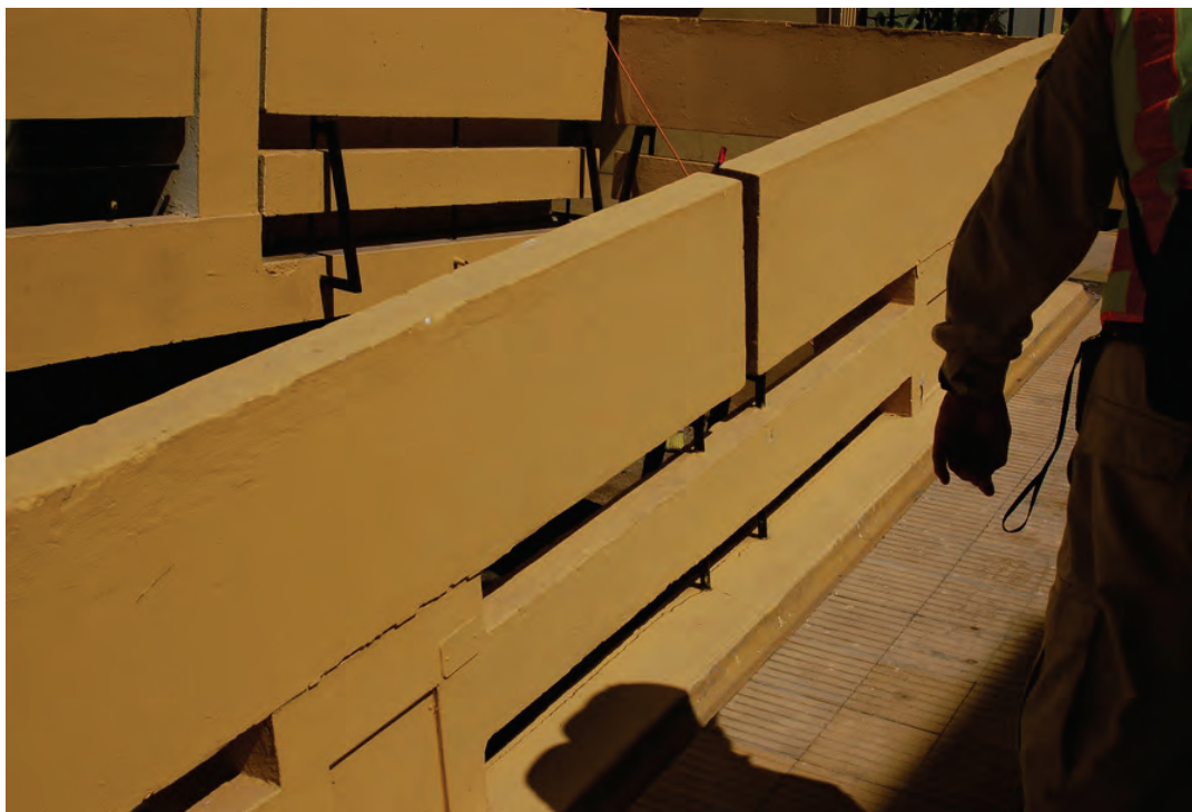
Figure 6.3.1.3-6 Residential building with precast concrete corridor and balcony railing panels. Some panels were damaged and subsequently many were removed to prevent falling. Location in Rancagua, Chile 154 miles northeast of the epicenter; estimated PGA of 0.3g during the 2010 magnitude-8.8 Chile Earthquake (Photo courtesy of Antonio Iruretagoyena, Rubén Boroschek & Associates).
