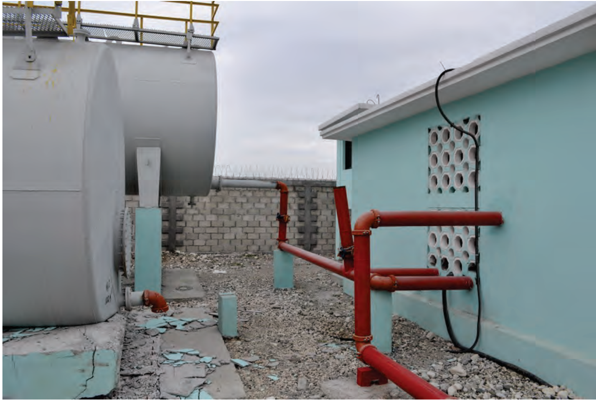
Figure 6.4.4.1-4 Collapse of water tank at left and broken piping disabled the fire protection system at this power plant in Port-au-Prince and led to the temporary plant closure in the 2010 magnitude-7 Haiti Earthquake (Photo courtesy of Eduardo Fierro, BFP Engineers).
