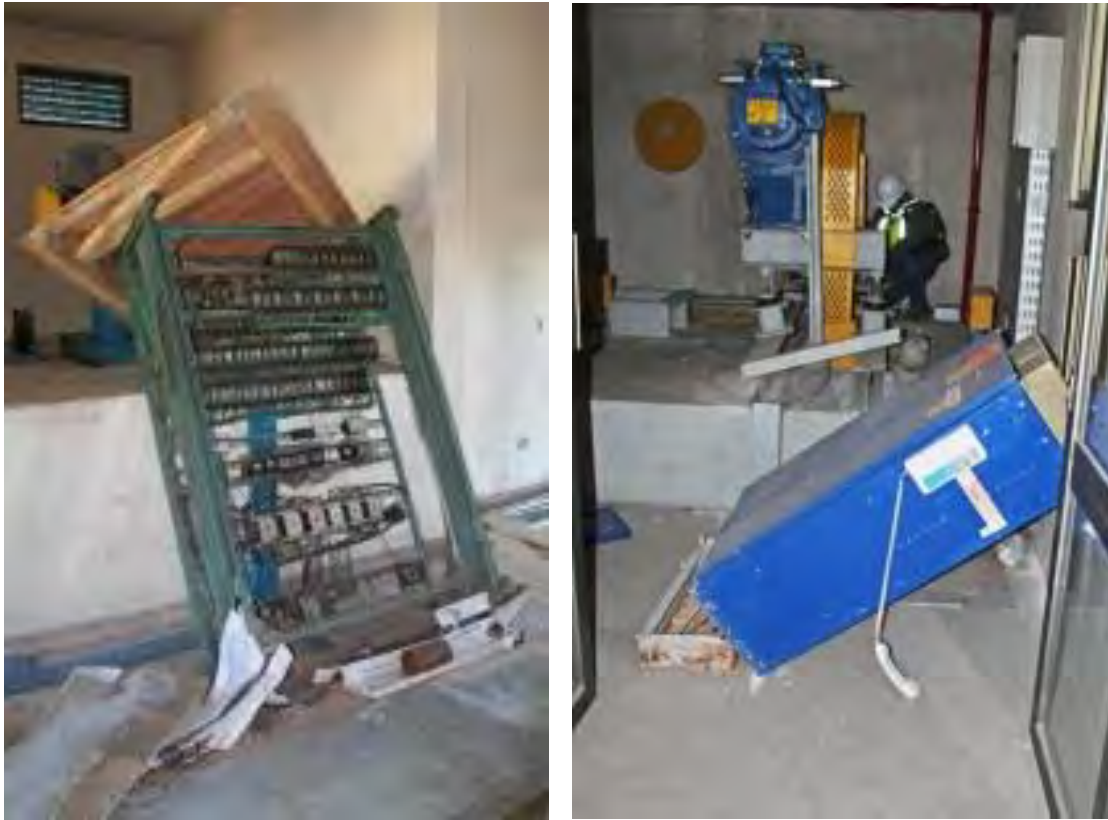
Figure 6.4.10.2-6 Overturned control panels in the 2010 Chile earthquake (Photos courtesy of Eduardo Miranda, Stanford University).
