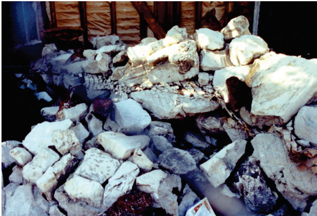
Figure 6.3.1.2-3 Rubble from failed anchored veneer as a result of the 1994 Northridge Earthquake (Photo courtesy of Robert Reitherman).
