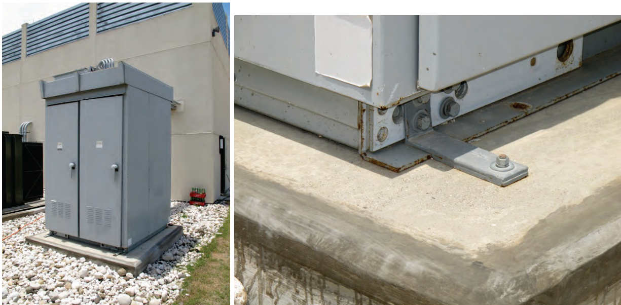
Figure 6.4.7.3-4 Outdoor low voltage switchgear supplying incoming utility power to critical facility. Note equipment frame seismic anchorage load path is bolted at both equipment frame and pad with a continuous rigid load path. Post earthquake photo from the 2010 M 7.0 Haiti earthquake. (photos courtesy of Philip J. Caldwell)
