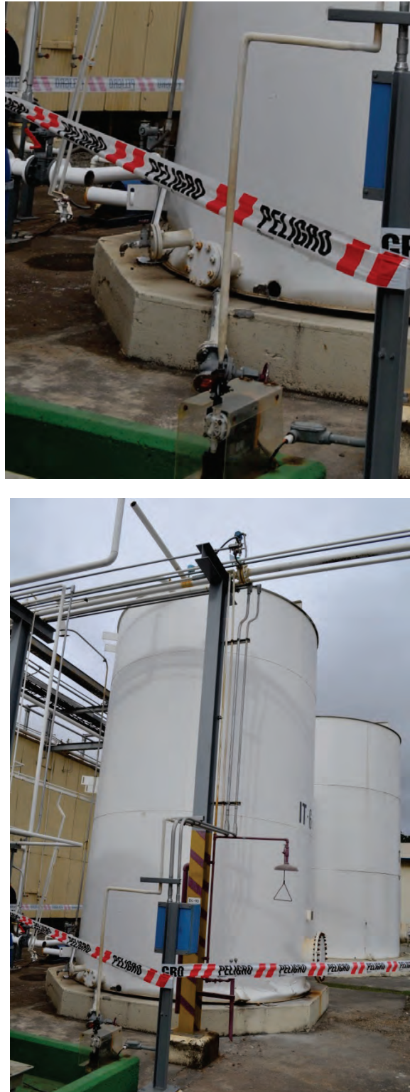
Figure 6.4.5.1-3 Elephant foot damage to inadequately anchored fuel tank in the 2010 Chile Earthquake also resulted in damage to fuel lines. Close-up photo shows failed pipe at welded joint (left) and pipe segment with attached valve (foreground) tore out of the tank wall (Photos courtesy of Eduardo Fierro, BFP Engineers).
