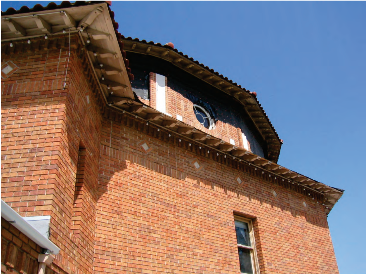
Figure 6.3.1.1-1 Failure of adhered masonry veneer at the Atascadero City Hall in the 2003 magnitude-6.5 San Simeon Earthquake (Photo courtesy of Mike Mahoney, FEMA).
