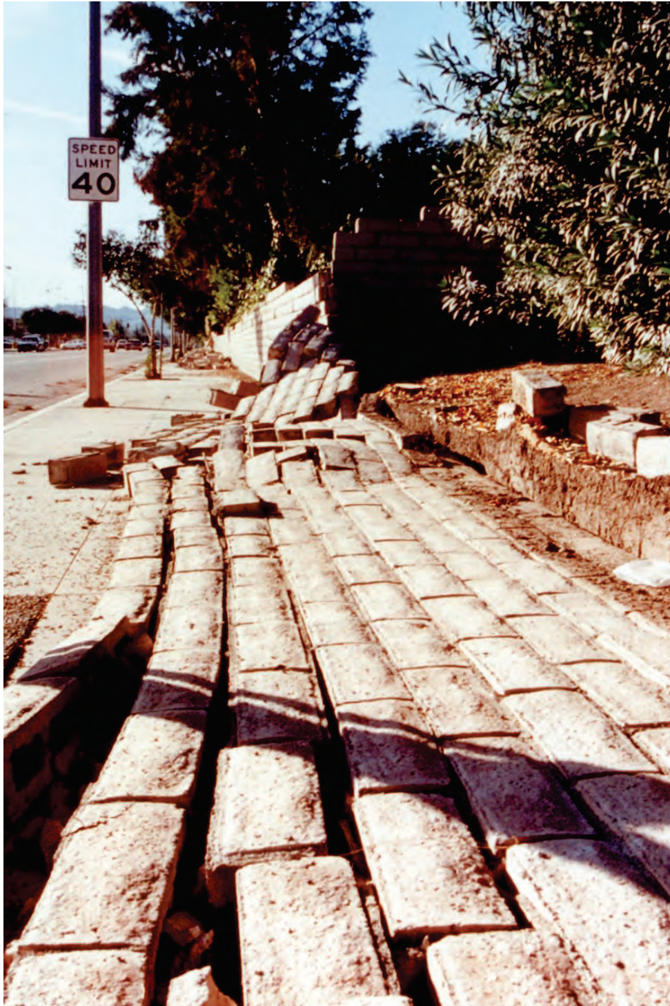
Figure 6.3.9.1-1 Collapse of freestanding CMU walls covering much of the sidewalk in the 1994 magnitude-6.7 Northridge Earthquake (Photo courtesy of Robert Reitherman). The rubble reveals that the wall was unreinforced.
