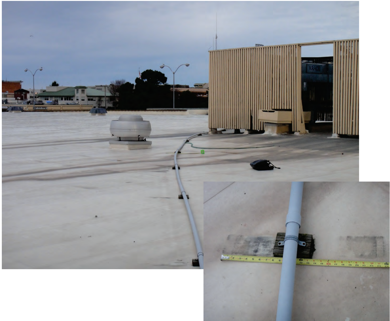
Figure 6.4.3.6-2 Unrestrained wood sleepers on roof-mounted piping slid a foot in either direction in 2010 magnitude-6.5 Eureka Earthquake (Photos courtesy of Maryann Phipps, Estructure).
