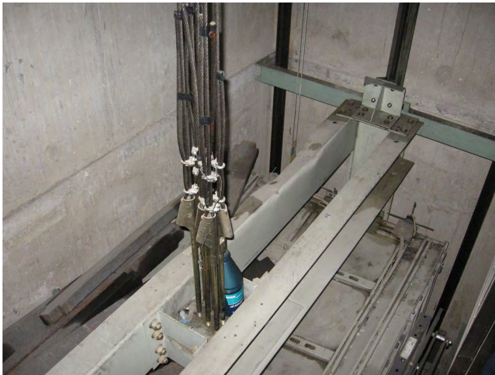
Figure 6.4.10.2-11 Unrestrained movement of the counterweights damaged the counterweight assembly and bent the counterweight guide rails; over half the subweights dropped onto the top of the cab and damaged the cab framing in the 2010
