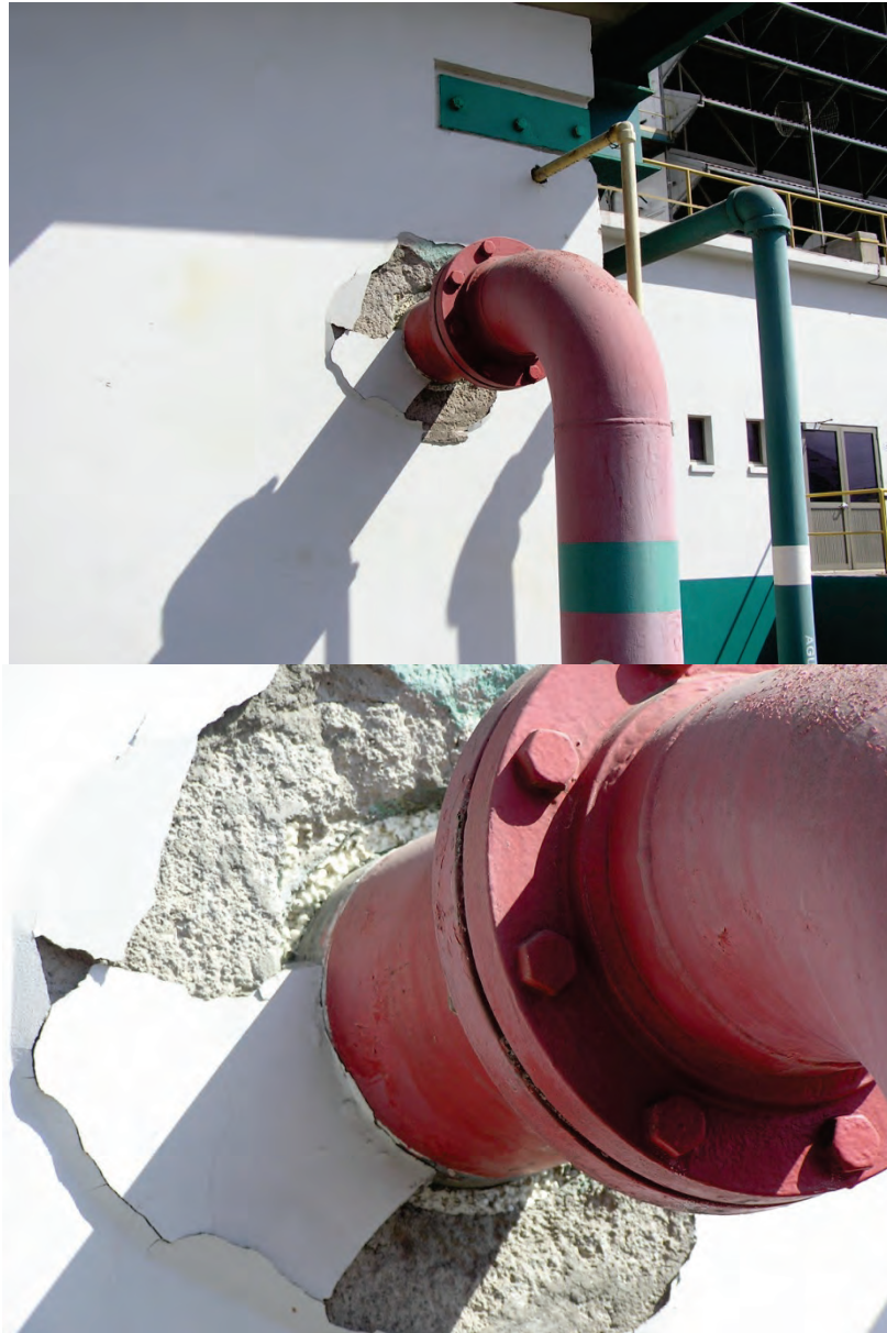
Figure 6.4.3.8-2 Exterior stucco damage at wall penetration for fire protection piping in the 2001 magnitude-8.4 Peru Earthquake (Photos courtesy of Eduardo Fierro, : BFP Engineers).
