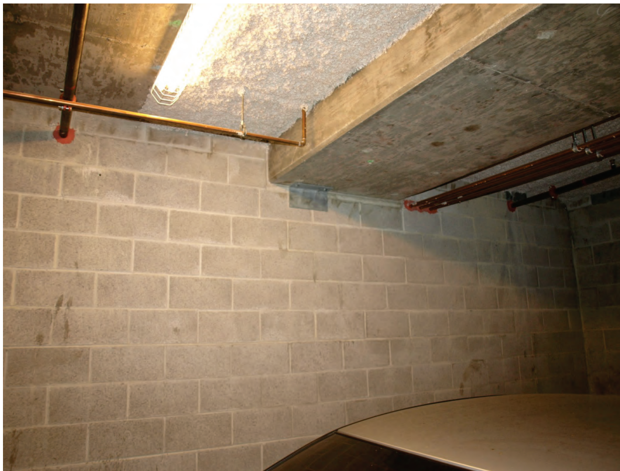
Figure 6.4.3.8-6 Series of pipe penetrations through a full-height CMU partition wall. Note pipe suspended from floor above; partition anchored to floor below and detailed with steel clip angles intended to provide lateral restraint for the wall but allow relative slip between the wall and slab above. The hangers will move with the floor above and the pipe at penetration will move with the wall. Lateral restraints are located immediately above floor (Photo courtesy Cynthia Perry, BFP Engineers).
