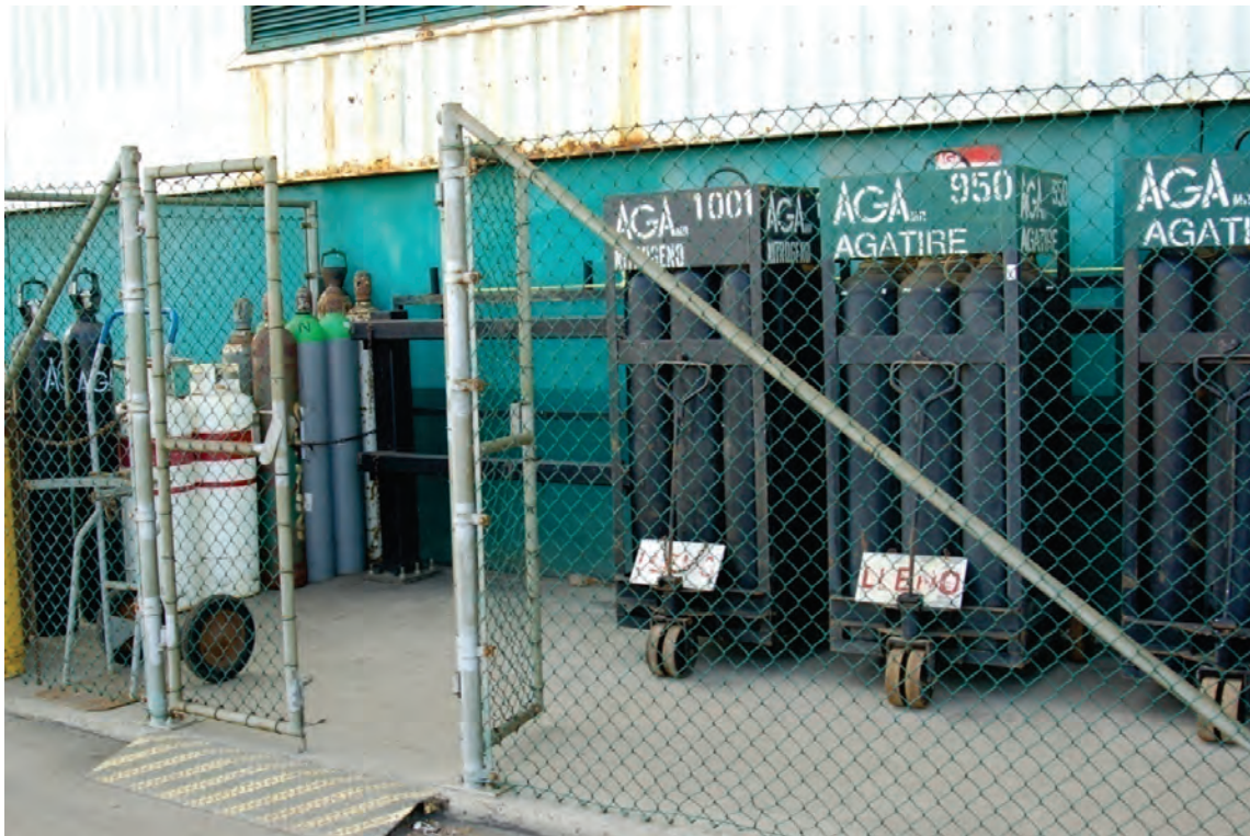
Figure 6.4.2.3-5 Steel tube supports for mobile gas cylinder carts (Photo courtesy of Eduardo Fierro, BFP Engineers).
