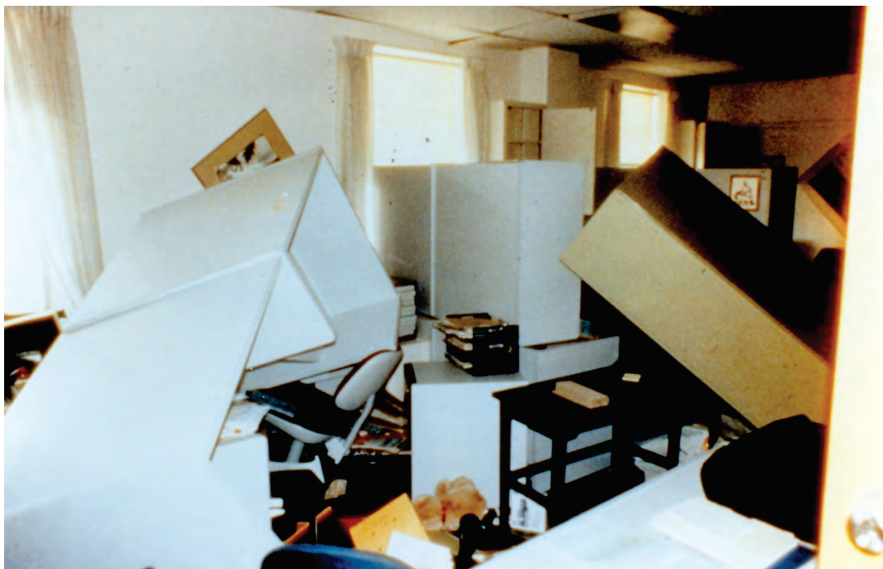
Figure 6.5.5.2-1 Damage to demountable partitions at the Veterans Administration Medical Center in Sepulveda as a result of the 1994 magnitude-6.7 Northridge Earthquake (Photo courtesy of James O. Malley).
