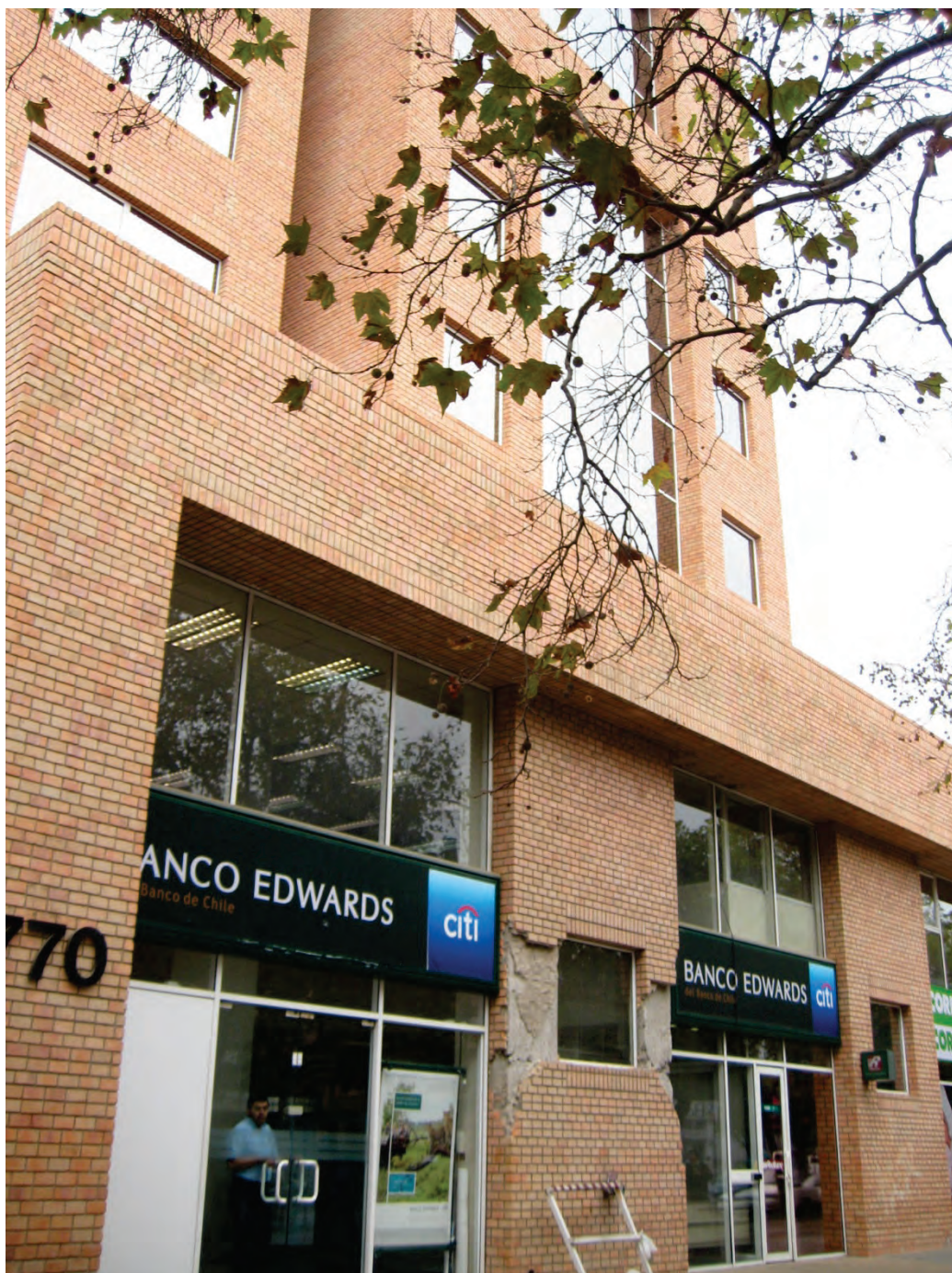
Figure 6.3.1.1-3 Cracked and spalled adhered veneer reveals incipient structural damage to concrete piers in Viña del Mar following the 2010 magnitude-8.8 Chile Earthquake. In this case, the areas of structural and nonstructural damage coincide; the adhered veneer remained intact over portions of the shear wall that did not deform significantly (Photo courtesy of Santiago Pujol, Purdue University).
