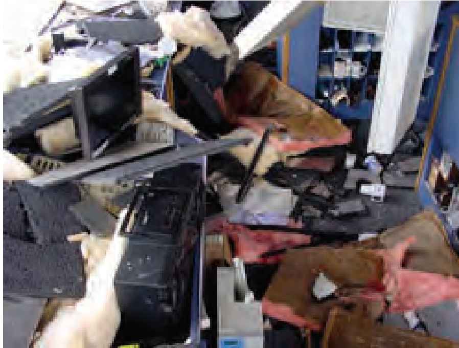
Figure 6.5.3.3-2 Damage to control tower at the SeaTac Airport in the 2001 Nisqually Earthquake (Photo courtesy of JCP Geologists).
