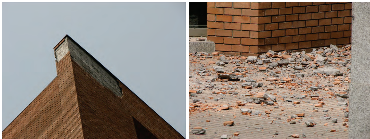
Figure 6.3.1.1-4 Failed adhered veneer fallen from parapet in Santiago following the 2010 magnitude-8.8 Chile Earthquake. (Photos courtesy of Antonio Iruretagoyena, Rubén Boroscheck & Associates)
