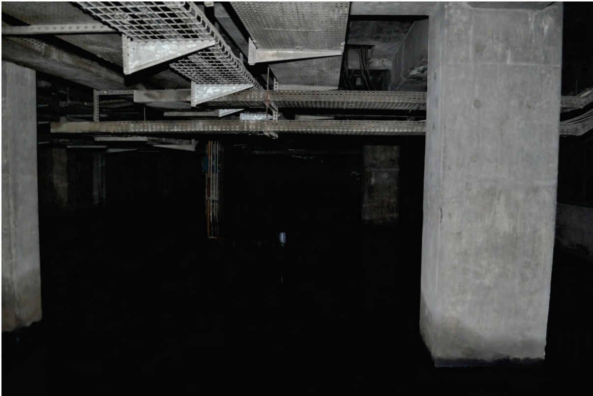
Figure 6.4.5.1-2 Basement level at power plant in Port-au-Prince flooded with oil and water in the 2010 magnitude-7 Haiti Earthquake creating hazardous conditions for inspection and clean-up (Photos courtesy of Eduardo Fierro, BFP Engineers).
