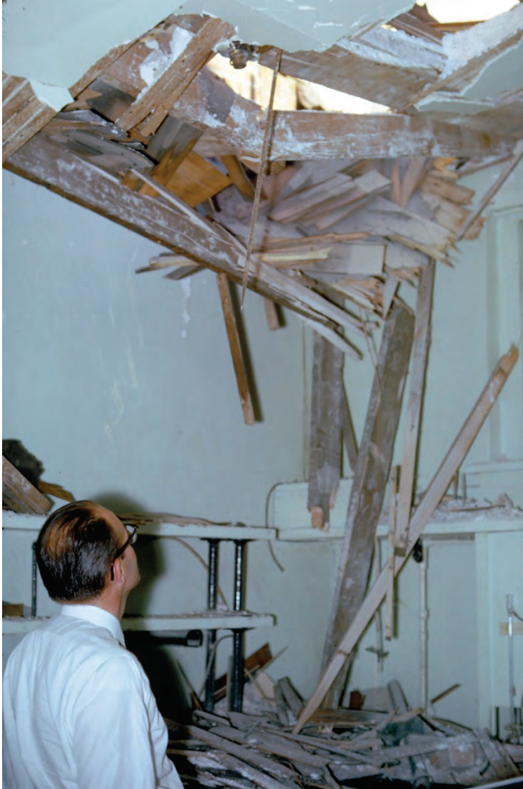
Figure 6.3.5.1-3 Damage to roof framing caused by failure of overhanging brick masonry during the 1962 magnitude-5.8 Cache Valley, Utah earthquake (Photo courtesy of PEER Steinbrugge Collection, No. S828).
