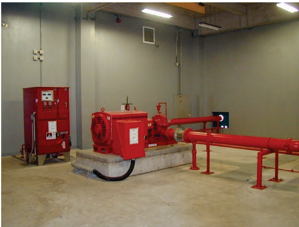
Figure 6.4.4.1-8 There was no damage to the fire suppression equipment in this control room in the 2001 Peru Earthquake because the pump and the control panel were well anchored and the piping had flexible connections with adequate sized wall penetration and no overhead falling hazards (Photo courtesy of Eduardo Fierro, BFP Engineers).
