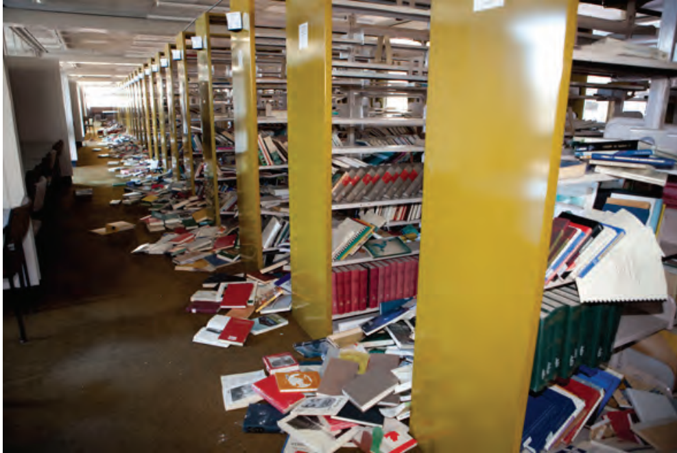
Figure 6.5.2.2-4 Shelving units with longitudinal ties did not fall over but all of the contents spilled to the floor in the 2010 Canterbury Earthquake. The use of lips or wires would have prevented the damage.(Photo courtesy of University of Canterbury).
