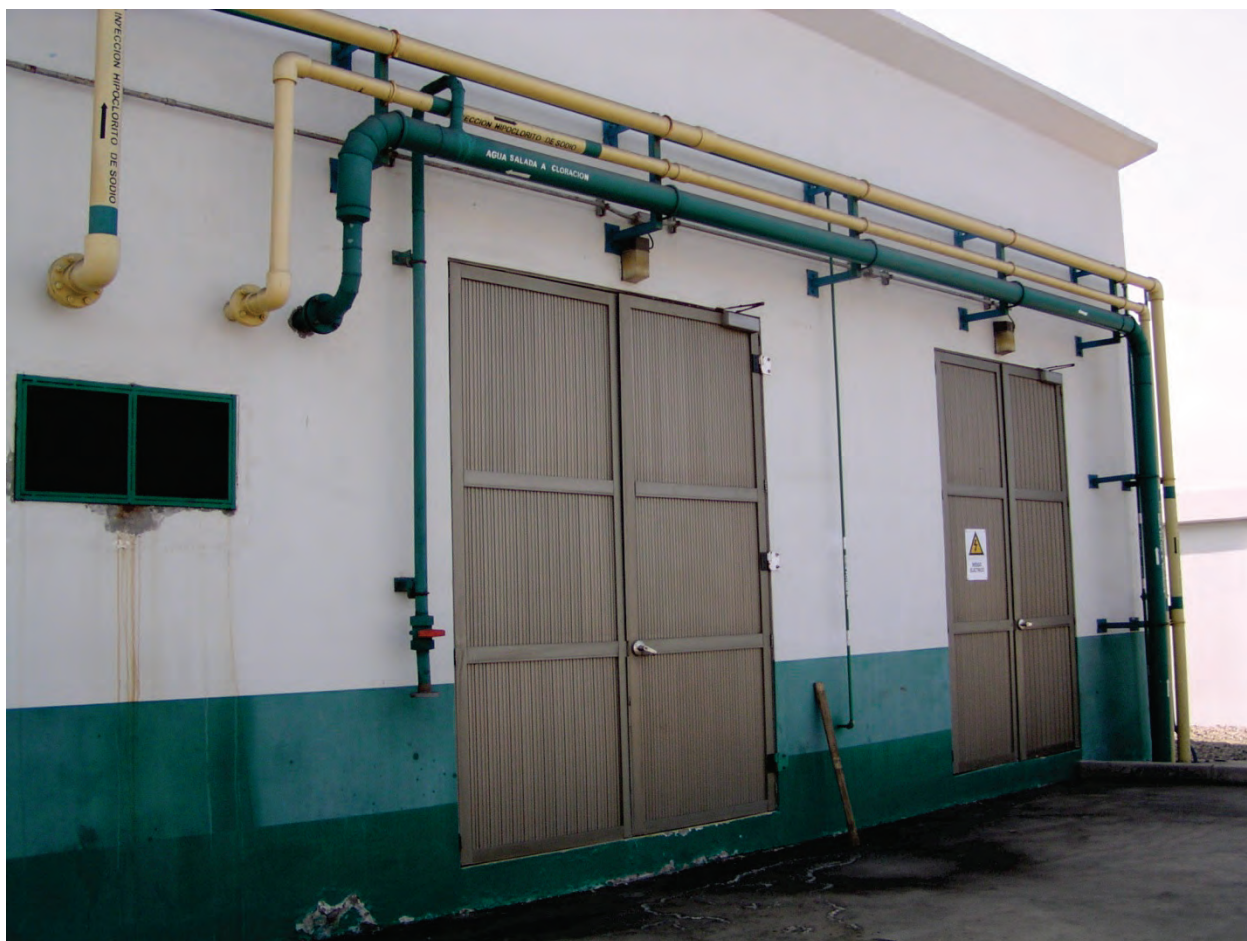
Figure 6.4.3.7-1 Wall-mounted supports for horizontal and vertical pipe runs with exterior exposure. Photo shows minor damage at wall penetration of green pipe and minor movement at some U-bolts, but restraints generally performed well (Photo courtesy of Eduardo Fierro, BFP Engineers). Note that lateral restraint near an elbow can be used to provide longitudinal restraint for a perpendicular pipe run.
