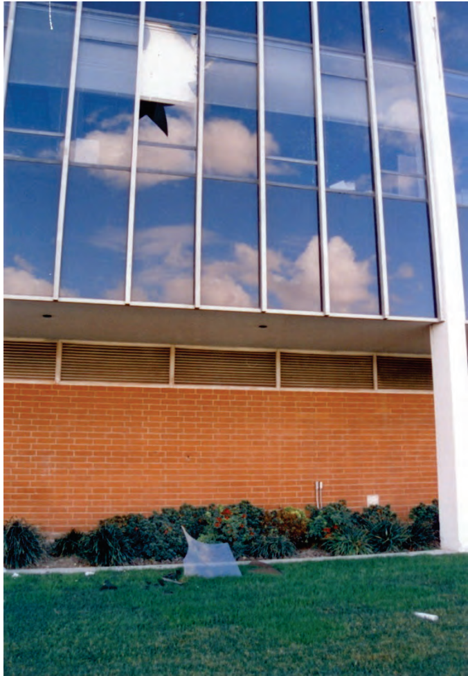
Figure 6.3.1.4-1 Shard of broken untempered glass that fell several stories from a multistory building in the 1994 Northridge Earthquake (Photo courtesy of Wiss, Jenney, Elstner Associates).
