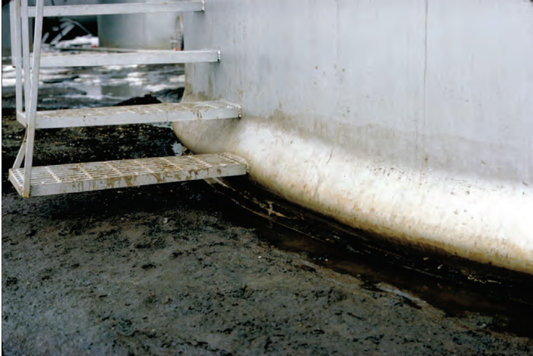
Figure 6.4.2.2-2 Tank with “elephant’s foot” buckle at the base in the 1964 magnitude-9.2 Anchorage, Alaska earthquake (Photo courtesy of PEER, Steinbrugge Collection, No. S2508)
