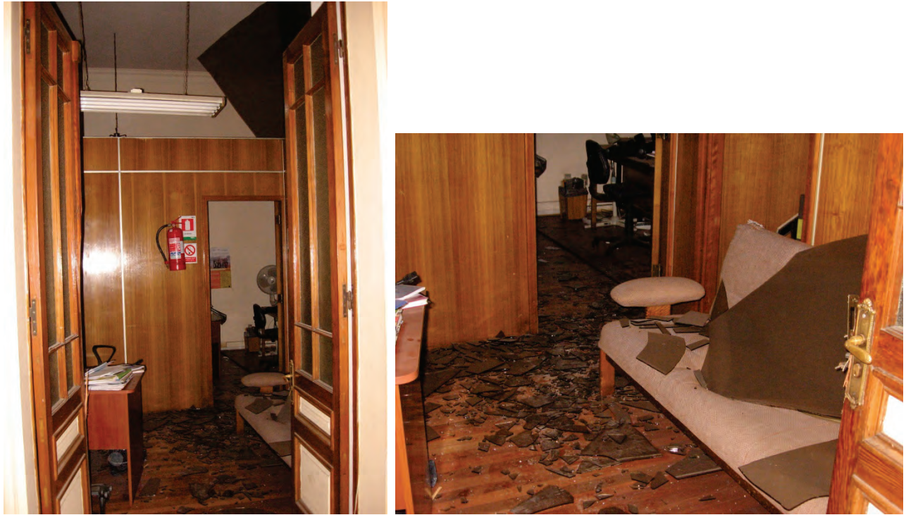
Figure 6.3.2.3-1 Glass shards fallen from the top of partial height office partitions in the reception area during the magnitude-8.8 2010 Chile Earthquake (Photo courtesy of Rodrigo Retamales, Rubén Boroscchek & Associates).
