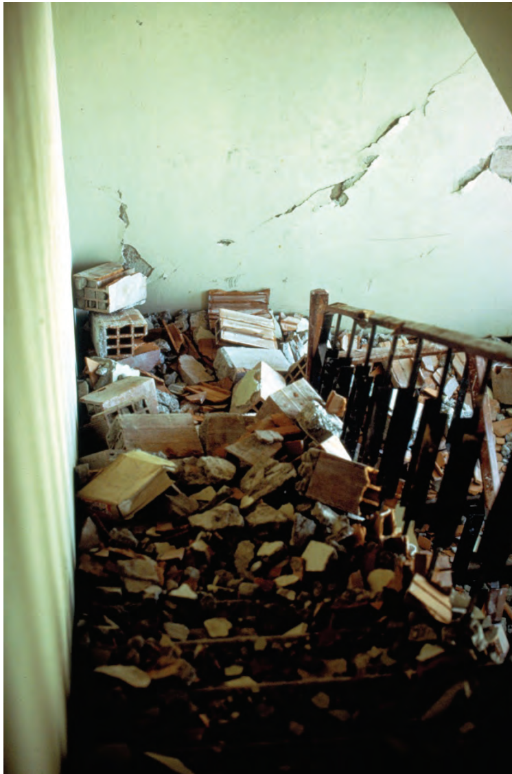
Figure 6.3.8.1-2 View of stairway in the Banco Central Building, Managua, Nicaragua after the 1972 magnitude-6.2 Managua Earthquake. Most of the stairs were covered with debris that resulted from the failure of the hollow tile partitions surrounding the stairs. This photograph highlights the need to not only prevent direct damage to stairway framing and connections, but also to protect against damage to surrounding walls (Photo courtesy of PEER Godden Collection, No. J94).
