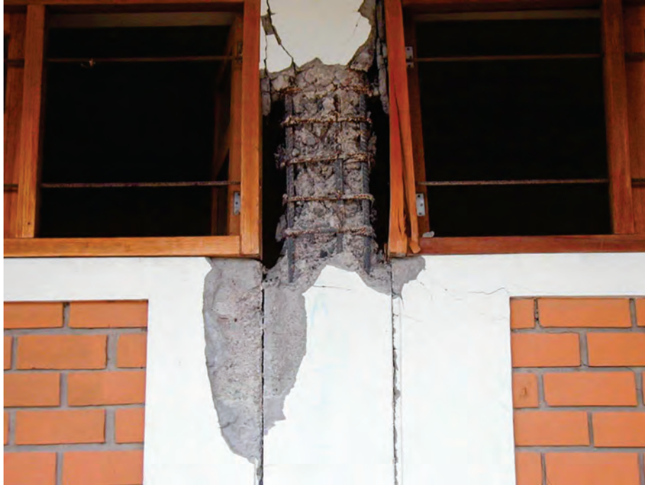
Figure 6.3.2.1-3 Damage to structural column (“captive column”) due to restraint caused by partial height masonry wall in the 2001 Peru Earthquake (Photo courtesy of Eduardo Fierro, BFP Engineers).
