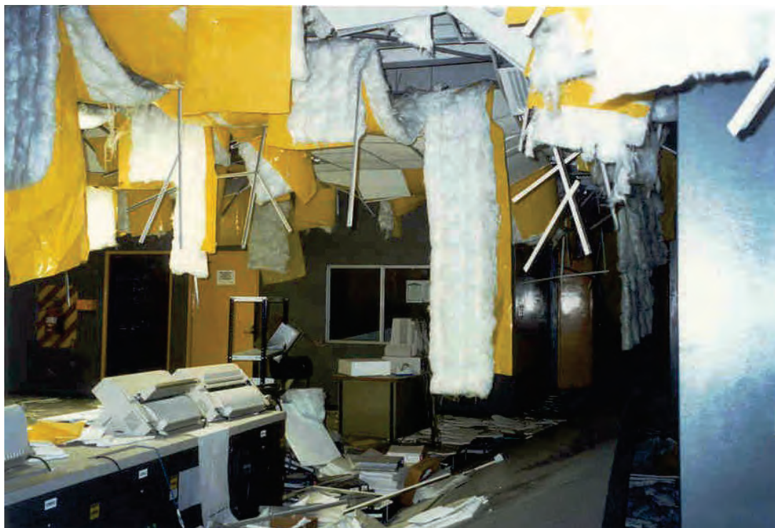
Figure 6.3.4.1-1 Failure of suspended ceiling system including lights, air diffusers, and insulation in control room of an industrial plant in the 2001 magnitude-8.4 Peru Earthquake (Photo courtesy of BFP Engineers).
