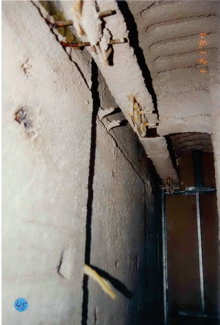
Figure 6.3.1.3-4 Interior view of precast panel showing response of three sets of push-pull connections in the 1994 Northridge Earthquake (Photo courtesy of OSHPD).
