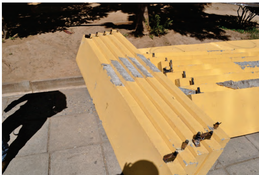
Figure 6.3.1.3-7 Numerous precast panels removed to prevent falling; detail from residential building in Rancagua, Chile above. These panels had a bearing seat at the center and supported on steel dowels at either end (Photo courtesy of Eduardo Fierro, BFP Engineers).
