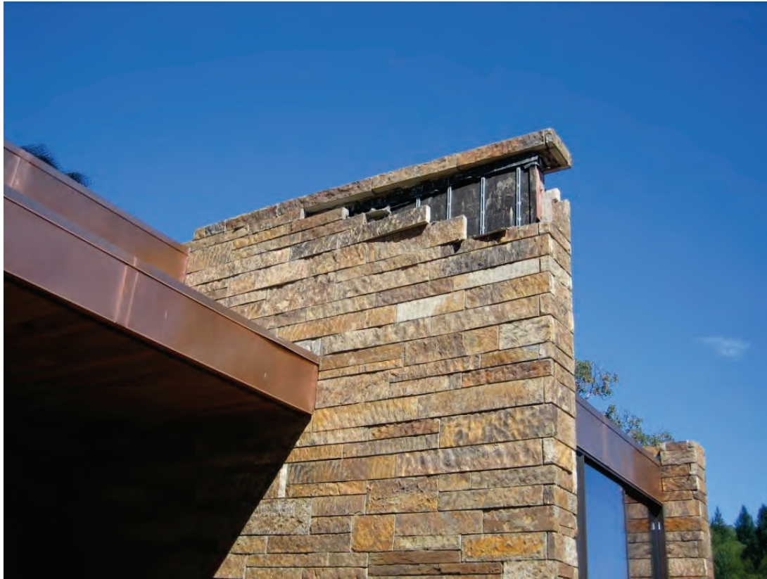
Figure 6.3.1.2-1 Fallen sandstone veneer as a result of a magnitude-4.4 earthquake in northern California. Post-earthquake investigation revealed missing dovetail anchors, missing pencil rods, and weak stone-to-mortar bond (Photo courtesy of Simpson Gumpertz and Heger).
