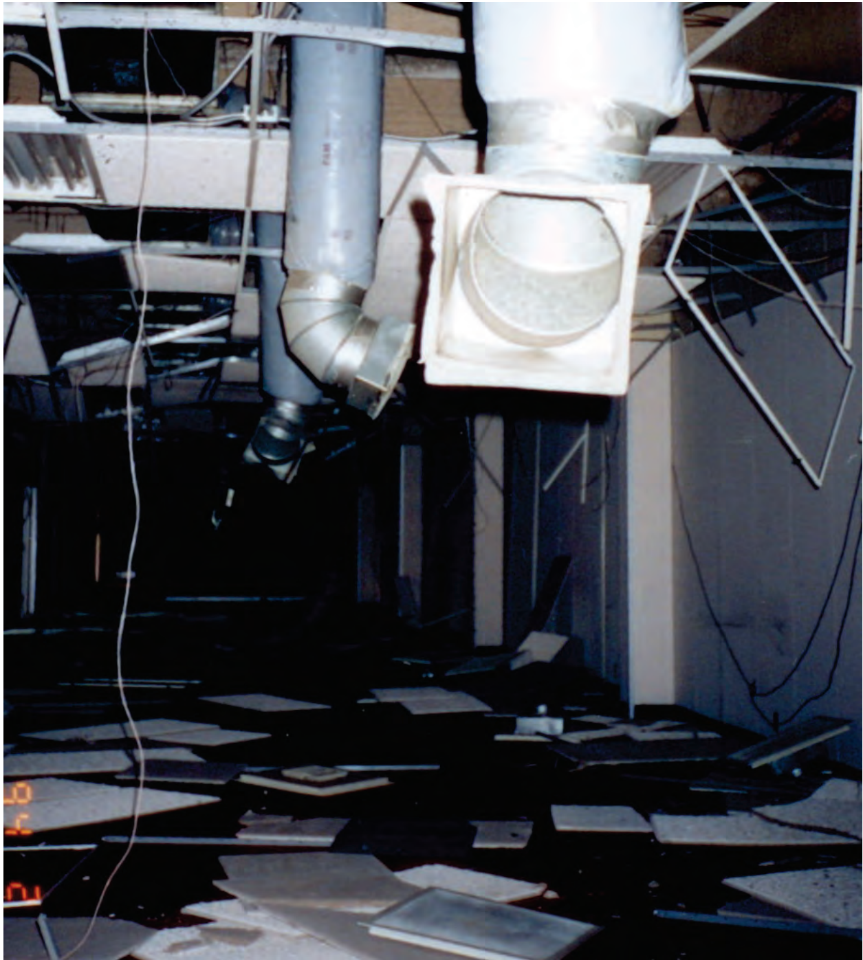
Figure 6.4.6.2-1 Air diffusers fell to the floor; ducts hanging through ceiling grid as a result of the 1994 Northridge Earthquake (FEMA 74, 1994).
