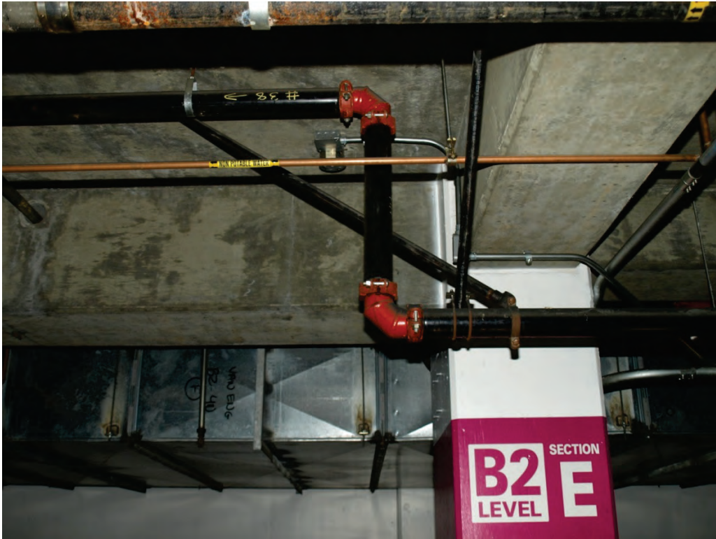
Figure 6.4.4.1-9 Transverse and longitudinal restraints on fire protection distribution line (Photo courtesy of Cynthia Perry, BFP Engineers).
