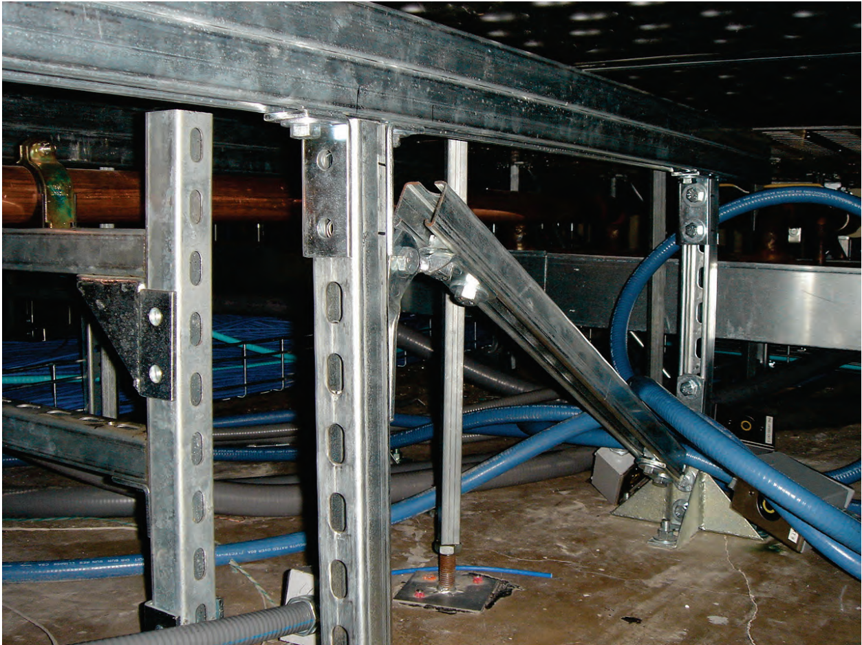
Figure 6.5.3.1-8 Strut framing added to brace data cabinet located on access floor. Bolts from angles above are connected to strut framing below (Photo courtesy of Maryann Phipps, Estructure).
