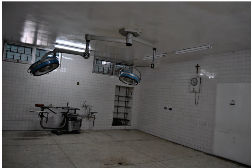
Figure 6.4.9.4-1 Operating room lights undamaged although hospital evacuated due to collapse of adjacent wing in the 2010 magnitude-7 Haiti Earthquake. Fixture anchored to underside of concrete slab (Photo courtesy of Ayhan Irfanoglu, Purdue University).
