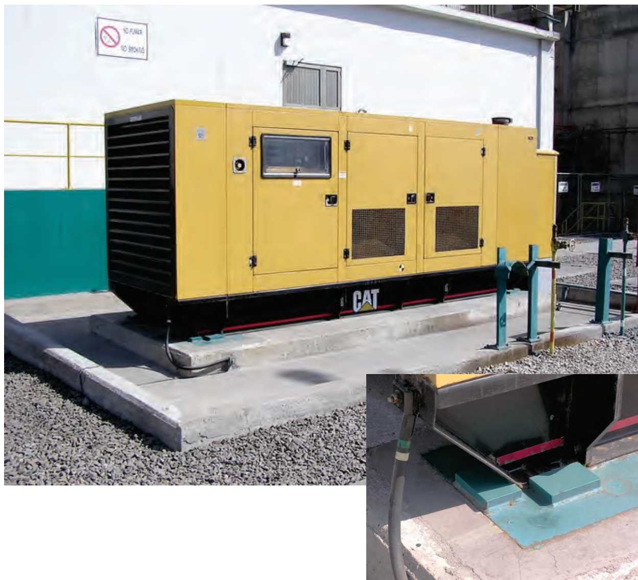
Figure 6.4.7.2-2 Emergency generator with skid mount on housekeeping pad; shear lugs added following the 2001 Peru Earthquake (Photo courtesy of Eduardo Fierro, BFP Engineers).
