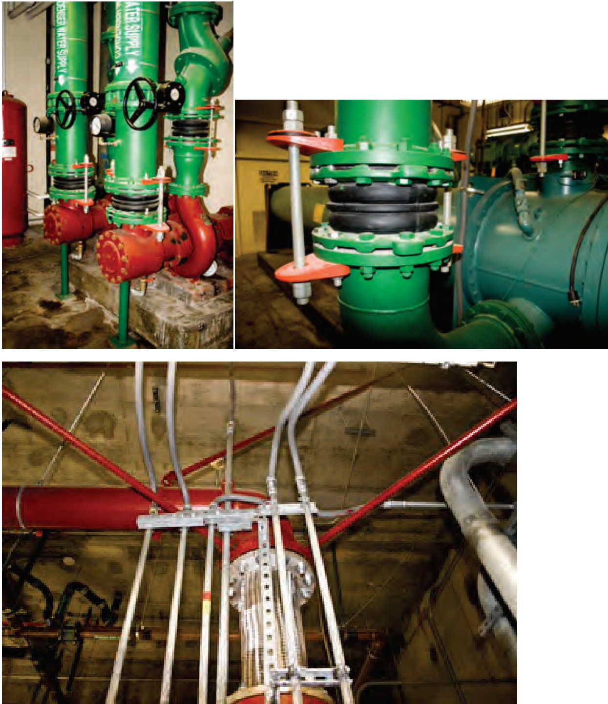
Figure 6.4.3.3-2 Examples of flexible couplings that performed well in the 2010 magnitude-7 Haiti Earthquake; the building suffered relatively minor damage (Photo courtesy of Tom Sawyer, Engineering News Record).
