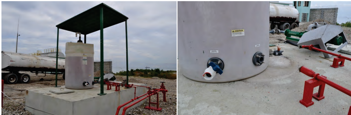
Figure 6.4.4.1-5 Unanchored holding tank slid on concrete pad, breaking fire protection piping and disabling the fire protection system in the 2010 Haiti Earthquake. In this case, the piping was well anchored but the tank was unrestrained (Photo courtesy of Eduardo Fierro, BFP Engineers).
