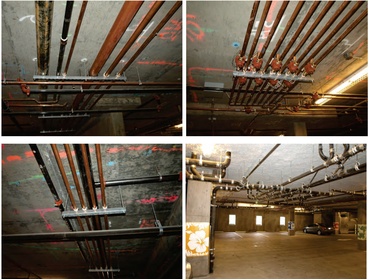
Figure 6.4.5.2-6 Piping installation in garage of mixed commercial/residential building San Francisco Bay Area completed in 2010. Note piping and trapeze supports do not have lateral restraints as all hangers were kept under 12" in length; only the sprinkler lines were laterally restrained. (Photo courtesy of Cynthia Perry, BFP Engineers).
