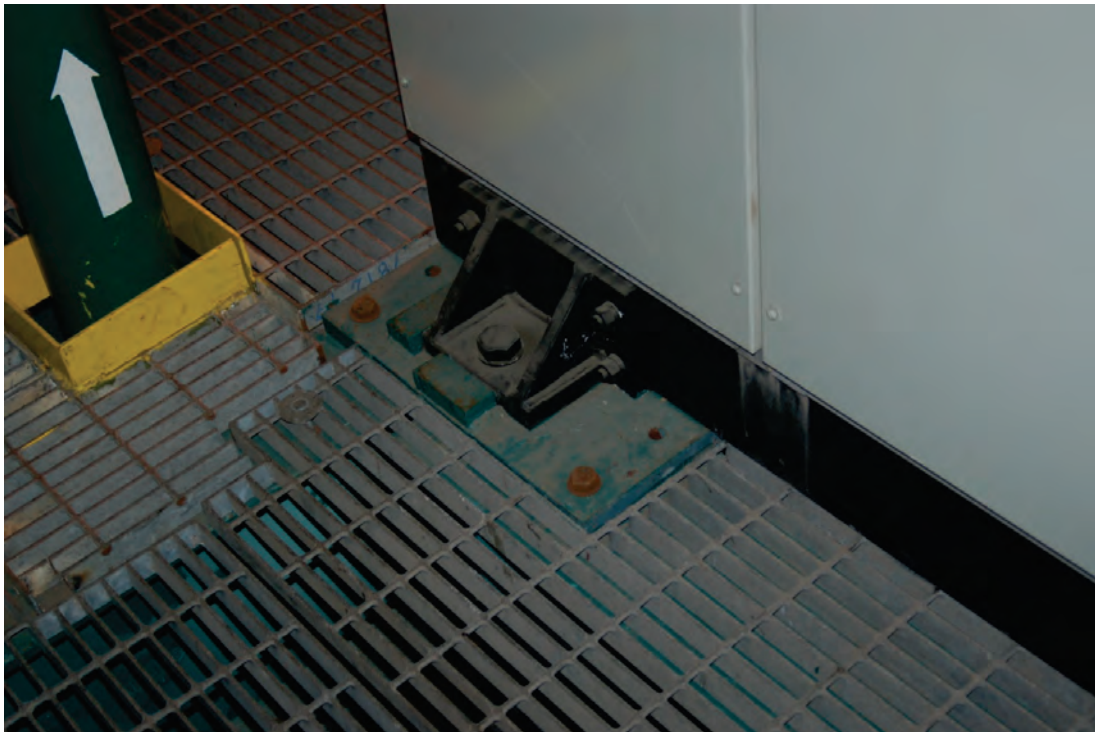
Figure 6.4.1.1-4 Bolted connection to steel skid with added shear lugs (Photo courtesy of Eduardo Fierro, BFP Engineers).
