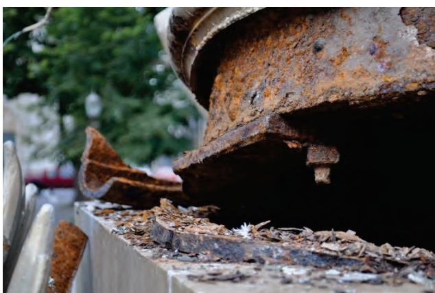
Figure 6.5.6.3-2 Leaning fountain after the 2010 Chile Earthquake; corrosion was a factor (Photos courtesy of Eduardo Fierro, BFP Engineers).
