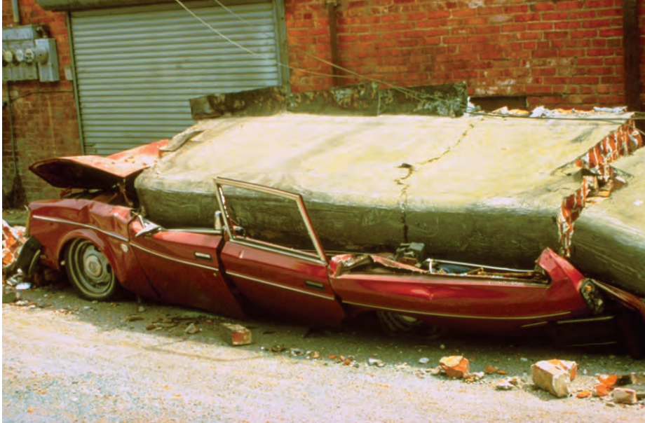
Figure 6.3.5.1-1 URM parapet fell and smashed two cars in the 1992 magnitude-7.2 Petrolia Earthquake. A parapet at same location in Ferndale, California failed in 1906 and killed two cows (NGDC, 2009).
