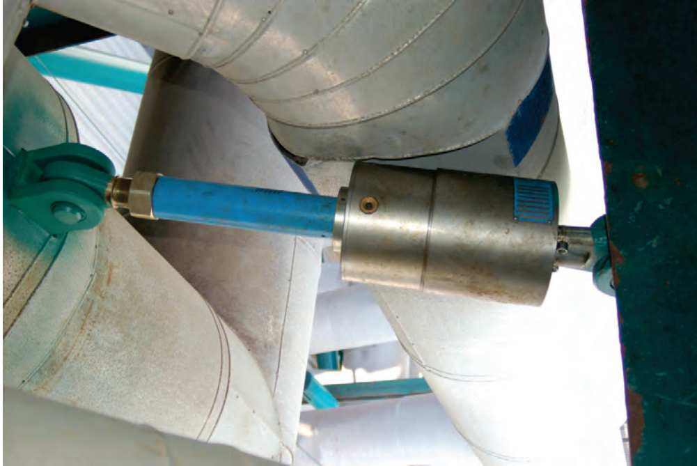
Figure 6.4.3.1-8 Viscous damper used as restraint on large insulated pipe (Photo courtesy of Eduardo Fierro, BFP Engineers).
