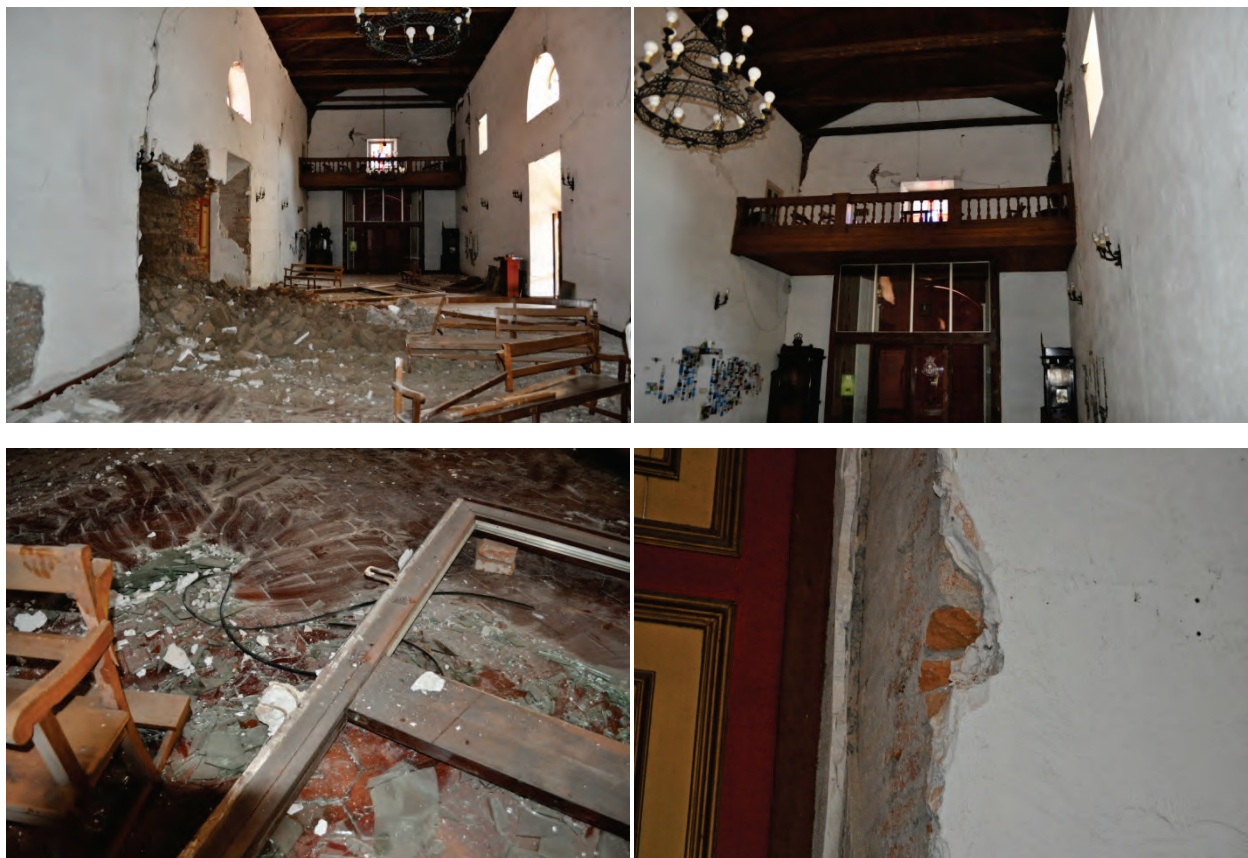
Figure 6.3.2.3-3 Failed wood framed glazing assembly in the 2010 Chile earthquake (Photo courtesy of Eduardo Fierro, BFP Engineers). The wood framing was held in place by metal or rebar brackets embedded in the masonry wall. The adobe wall on the left of the door collapsed and the brackets on the right side pulled out of the brick masonry wall (lower right). The glazing assembly at the rear entrance of the chapel was anchored overhead to the wood balcony framing and was undamaged.
