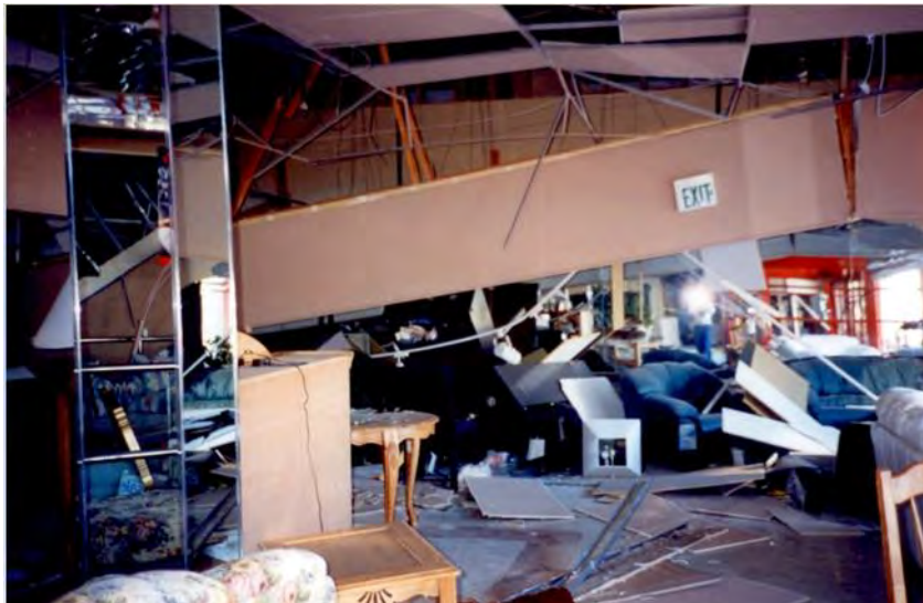
Figure 2.4.1-3 Failure of suspended ceilings and light fixtures in a furniture store (FEMA 74, 1994).
