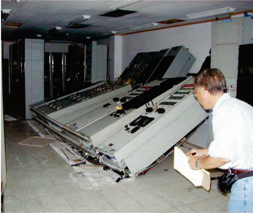
Figure 6.4.7.1-1 Overturned equipment in the 1985 magnitude-8 Mexico Earthquake, note absence of anchorage of equipment base to floor (Photo courtesy of Degenkolb Engineers).
