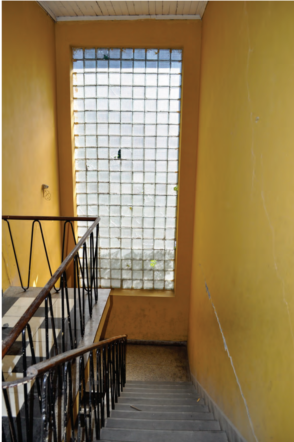
Figure 6.3.1.5-2 Damage to glass block with rigid mortar on all sides and in all joints in the 2010 Chile Earthquake (Photo courtesy of Eduardo Fierro, BFP Engineers). About 25% of the glass block units are cracked or broken but entire panel will need to be removed and replaced.
