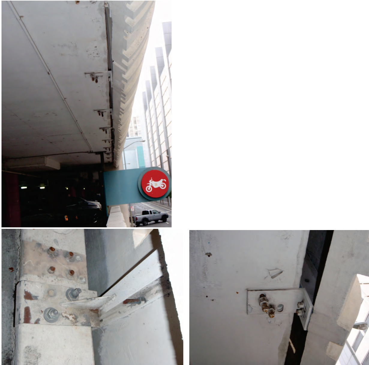
Figure 6.3.1.3-9 Precast spandrel panel in San Francisco parking garage supported by bearing connections near top of panel (left) and slotted connections at bottom of panel (right); panels have four connections each. The remnants of a previous nonductile connection detail are visible in the photo at left (Photo courtesy of Cynthia Perry, BFP Engineers).
