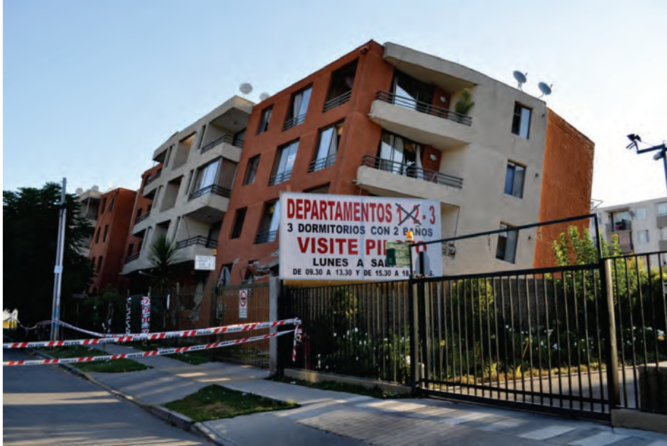
Figure 6.4.7.6-1 Most antennae are designed for wind and able to resist seismic loading. In spite of the collapse of the first story of this residential building complex, the roof-mounted antennae appear intact in the 2010 magnitude-8.8 Chile Earthquake (Photo courtesy of Eduardo Fierro, BFP Engineers).
