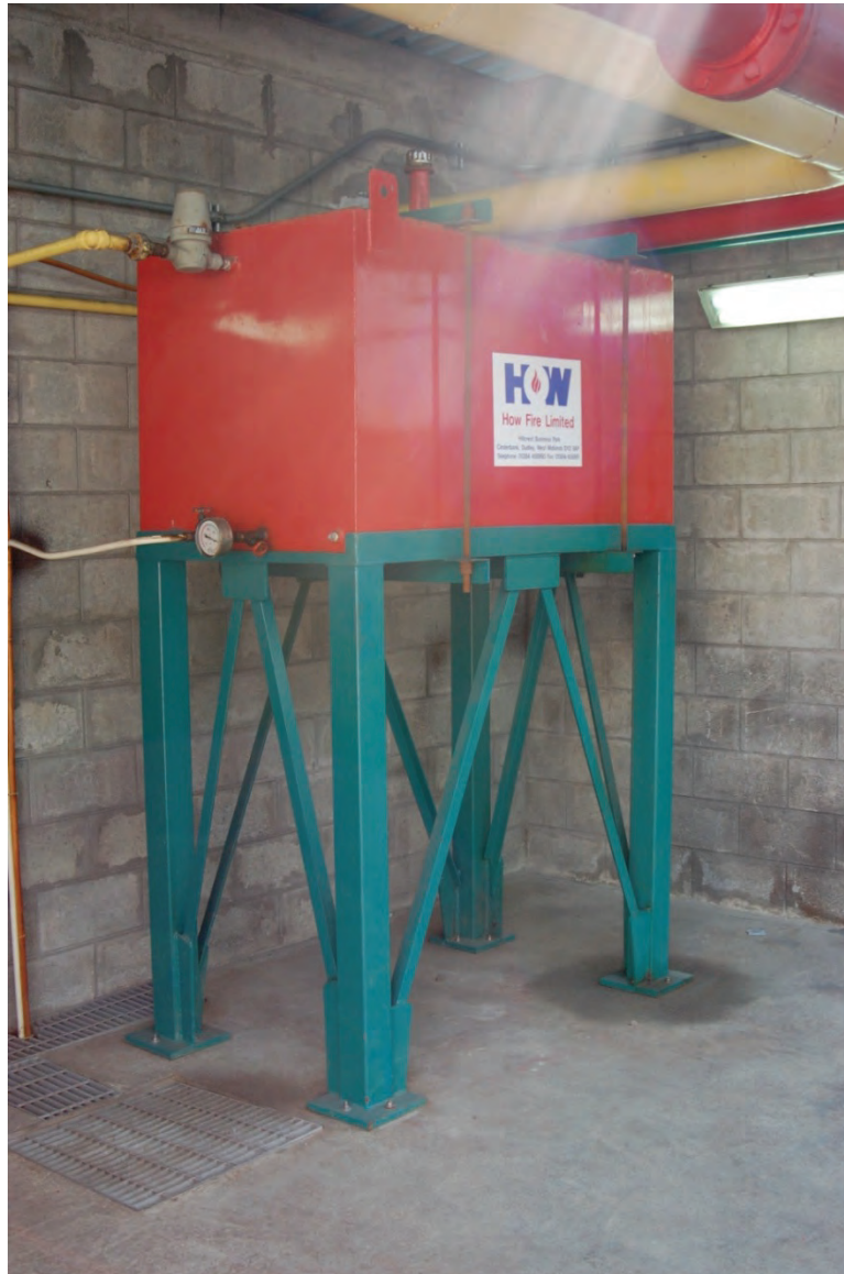
Figure 6.4.2.1-6 Braces added to four sides of tank support structure (Photo courtesy of Eduardo Fierro, BFP Engineers).
