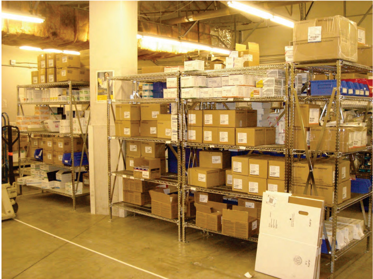
Figure 6.5.1.1-7 Fixed base shelving units anchored directly to concrete slab through base plate (Photo courtesy of Maryann Phipps, Estructure).
