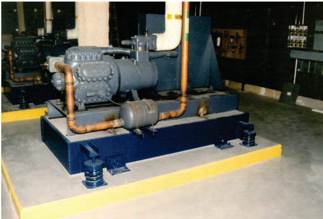
Figure 6.4.1.3-6 Open springs and snubbers used to support equipment (Photo courtesy of Mason Industries).
