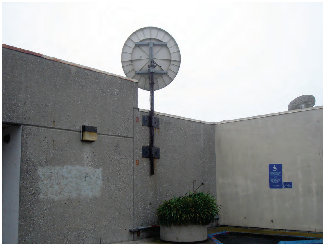
Figure 6.4.7.6-5 Antenna mast mounted to concrete wall surface at top floor of building (Photo courtesy of (Photo courtesy of Maryann Phipps, Estructure). Note that two wall brackets are used to resist moments produced by wind or seismic forces. This antenna is larger than most standard residential versions.
