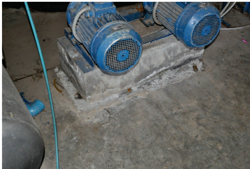
Figure 6.4.1.1-2 Pumps with rigid anchorage to housekeeping pad in the 2010 magnitude-8.8 Chile Earthquake; housekeeping pad not anchored to base slab and slid horizontally several inches (Photo courtesy of Eduardo Fierro, BFP Engineers).
