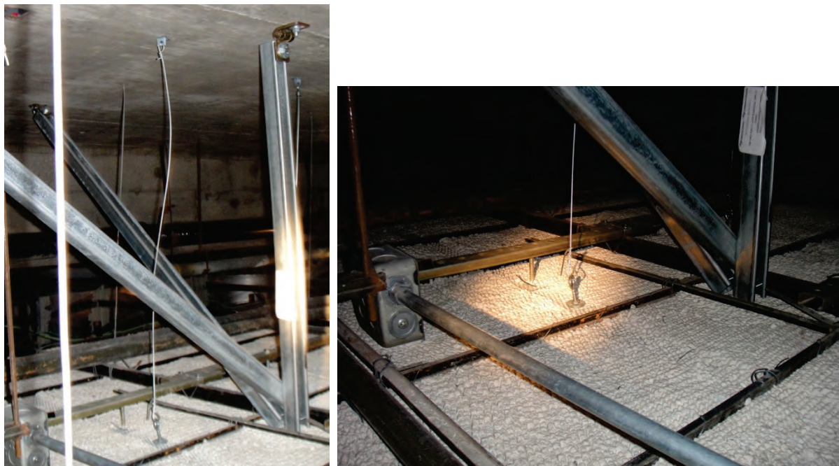
Figure 6.4.9.2-3 Independent vertical support for surface-mounted light fixture in suspended gypsum board ceiling located in California hospital. Eye hook and slack wire from fixture is tied to concrete slab above. The rigid bracing in the photos is attached to the ceiling grid, not the light fixture (Photos courtesy of Maryann Phipps, Estructure).
