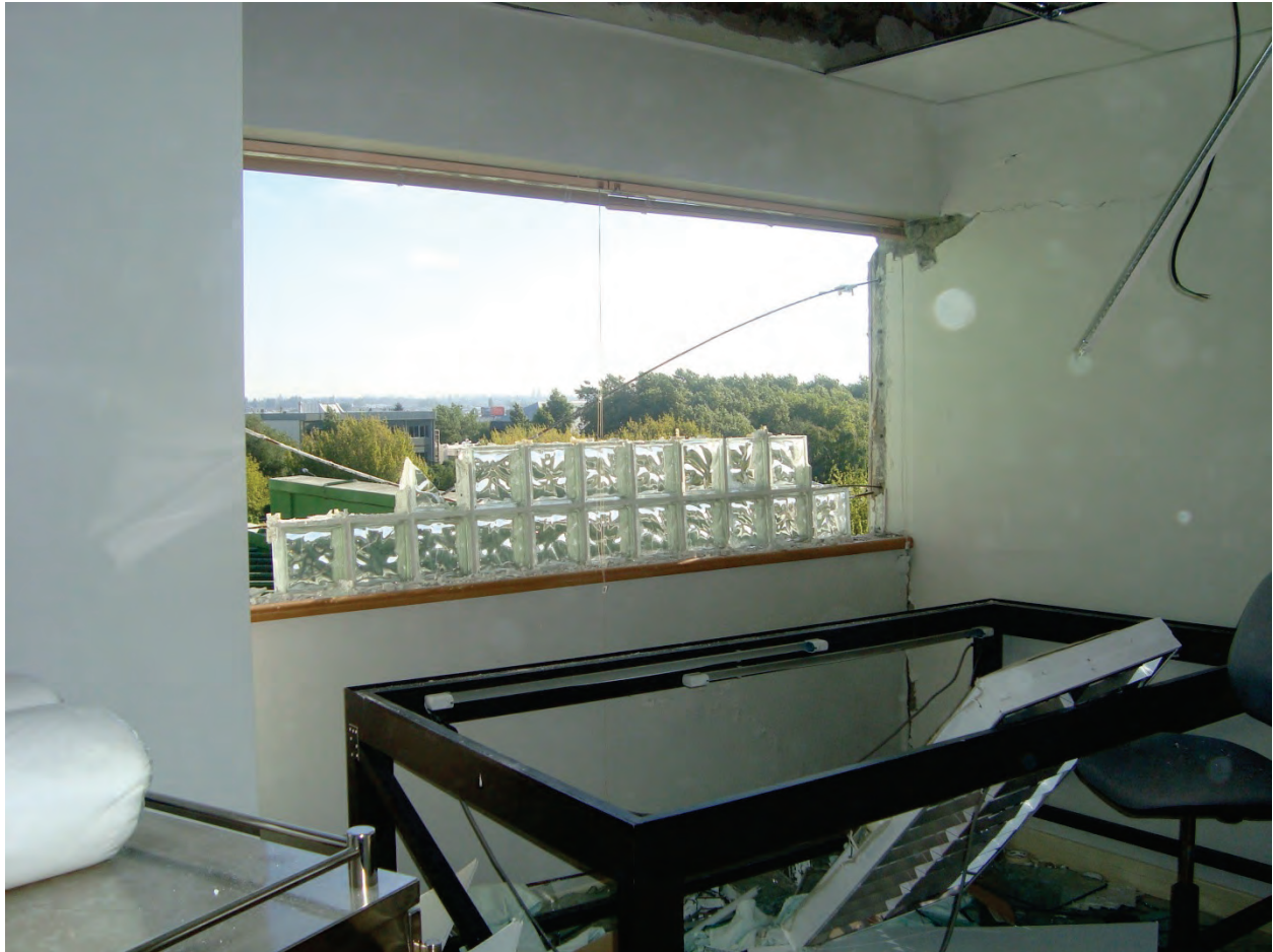
Figure 6.3.1.5-3 Damaged glass block panel from the Los Angeles Hospital in the 2010 Chile Earthquake; relatively new hospital building that had to be evacuated for repairs (Photo courtesy of Bill Holmes, Rutherford & Chekene). Blocks were installed with steel reinforcing bars in the top and bottom horizontal joints.
