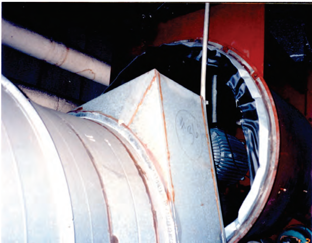
Figure 6.4.1.5-2 Sheet metal duct separated from suspended fan unit (Photo courtesy of Wiss, Jenney, Elstner Associates).
