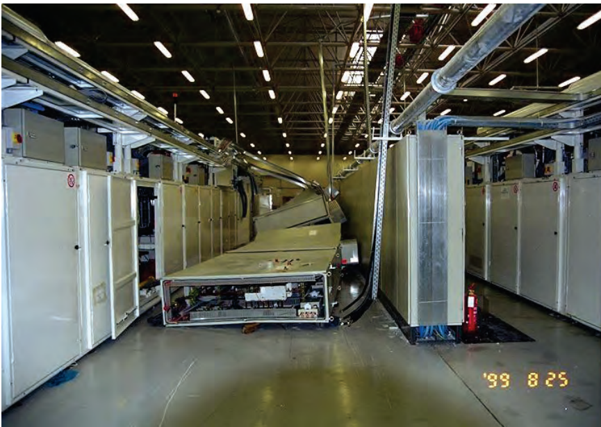
Figure 6.4.7.1-2 Unanchored electrical cabinets overturned in a paper products plant during the 1999 magnitude-7.4 Izmit, Turkey earthquake (Photo courtesy of NISEE Izmit Collection, No. IZT-682, photograph by Halil Sezen).
