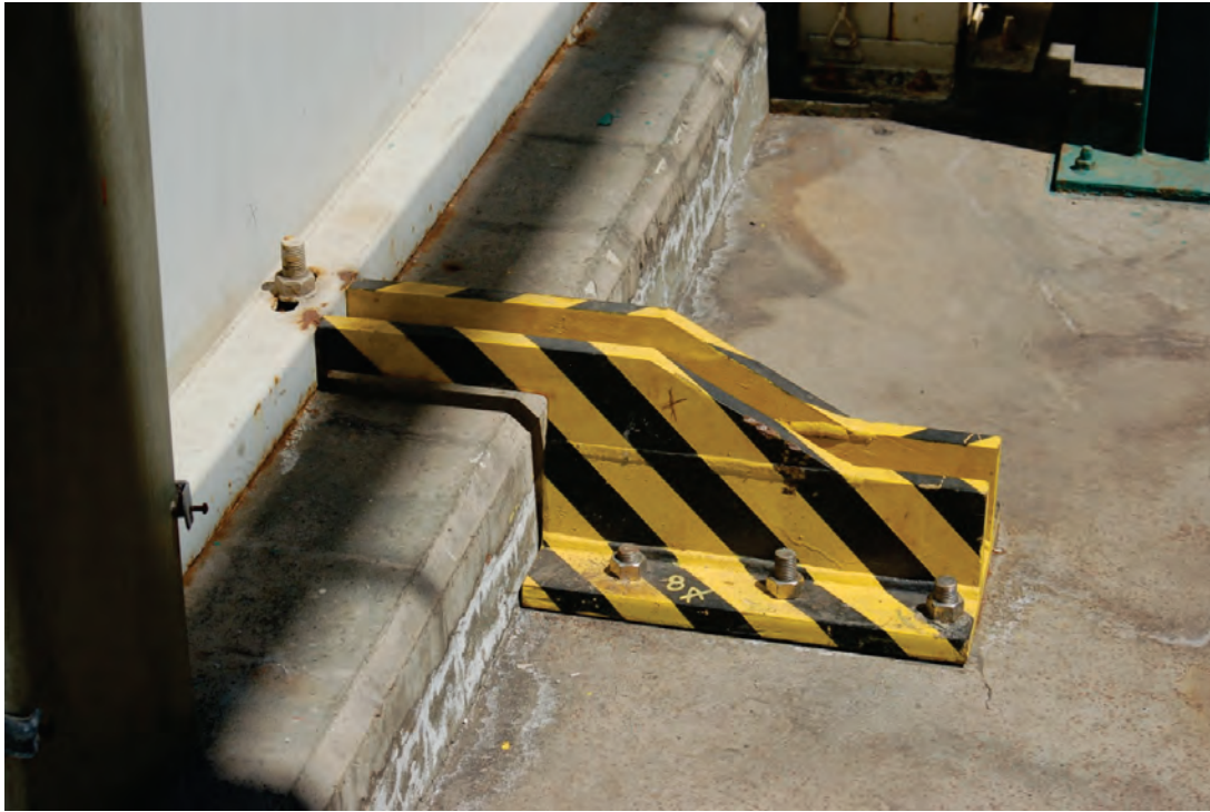
Figure 6.4.1.1-3 Added lateral capacity provided for skid-mounted equipment added following the 2001 Peru Earthquake (Photo courtesy of Eduardo Fierro, BFP Engineers).
