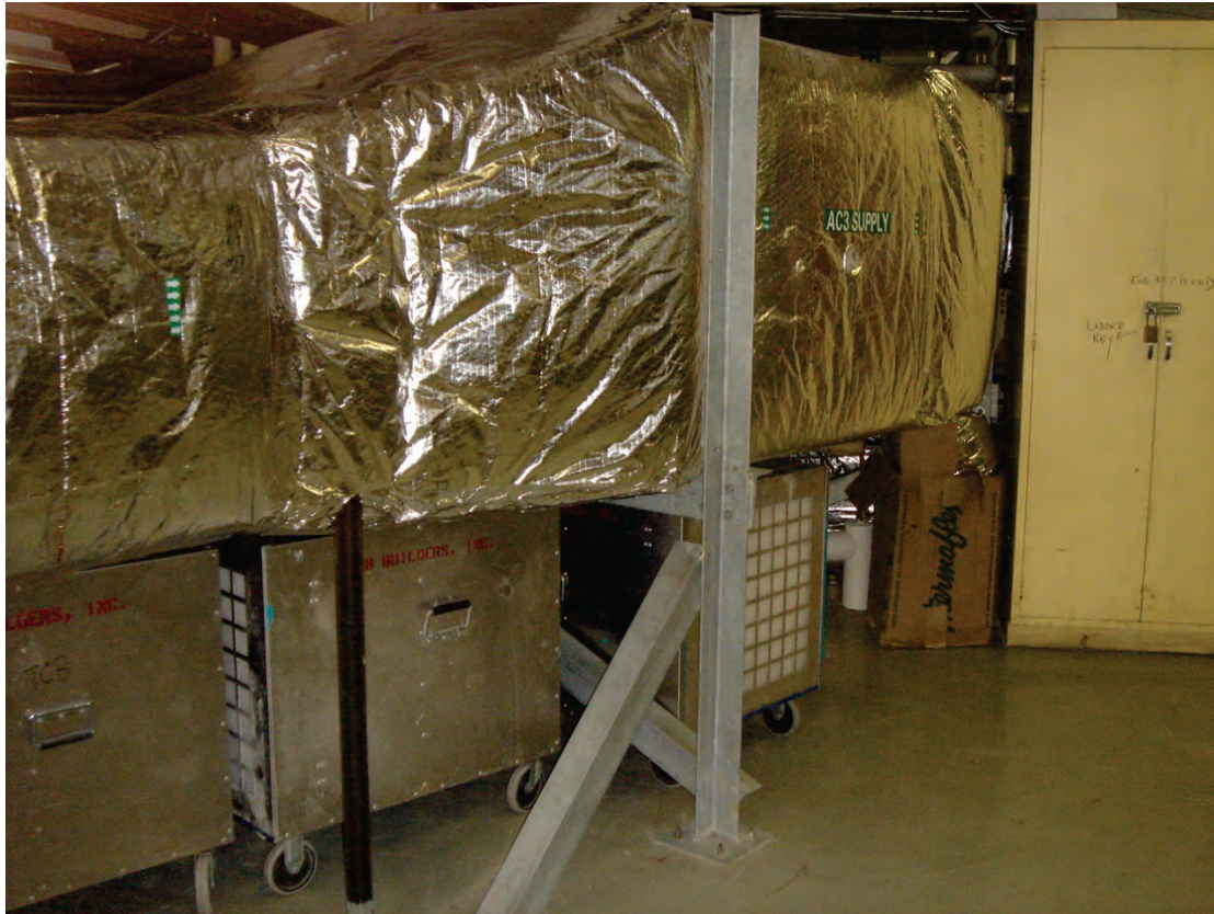
Figure 6.4.6.1-5 Floor-mounted rectangular duct supported on braced support stand built up from steel angles (Photo courtesy of Maryann Phipps, Estructure).
