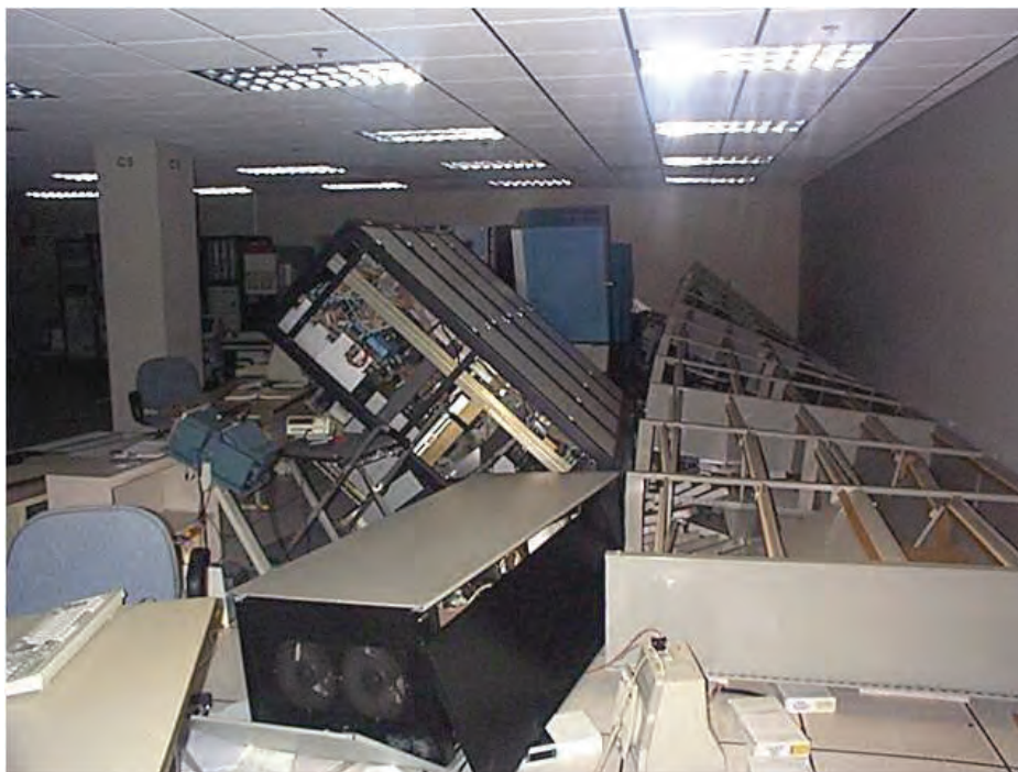
Figure 6.5.3.2-1 Damage to communication and computer racks (Photo courtesy of Degenkolb Engineers).
