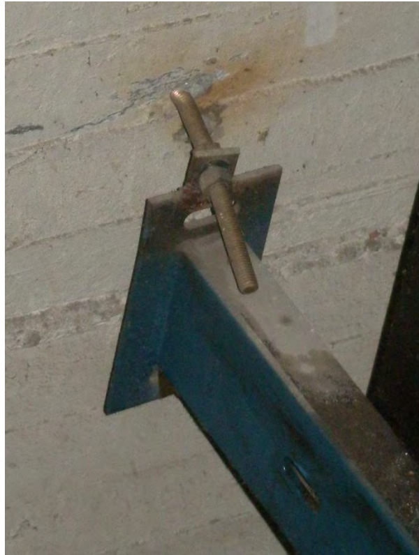
Figure 6.4.10.2-8 Damage to guide rail support brackets in the 2010 Chile Earthquake (Photo courtesy of Gilberto Mosqueda, SUNY Buffalo).
