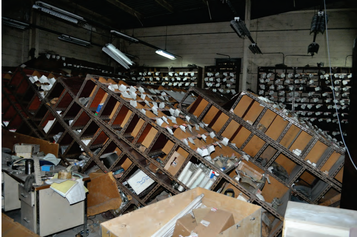
Figure 6.5.1.1-1 Collapse of row of unanchored freestanding shelving units containing spare parts at an electric power plant in Port-au-Prince in the 2010 magnitude-7 Haiti Earthquake (Photo courtesy of Eduardo Fierro, BFP Engineers).
