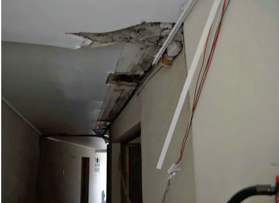
Figure 6.3.4.2-1 Damage to metal lath and plaster ceiling applied to the underside of the concrete slab in 10-story residential building in the 2010 magnitude-8.8 Chile Earthquake (Photo courtesy of Eduardo Fierro, BFP Engineers). The damage occurred due to pounding at the interface between two wings of the structure.
