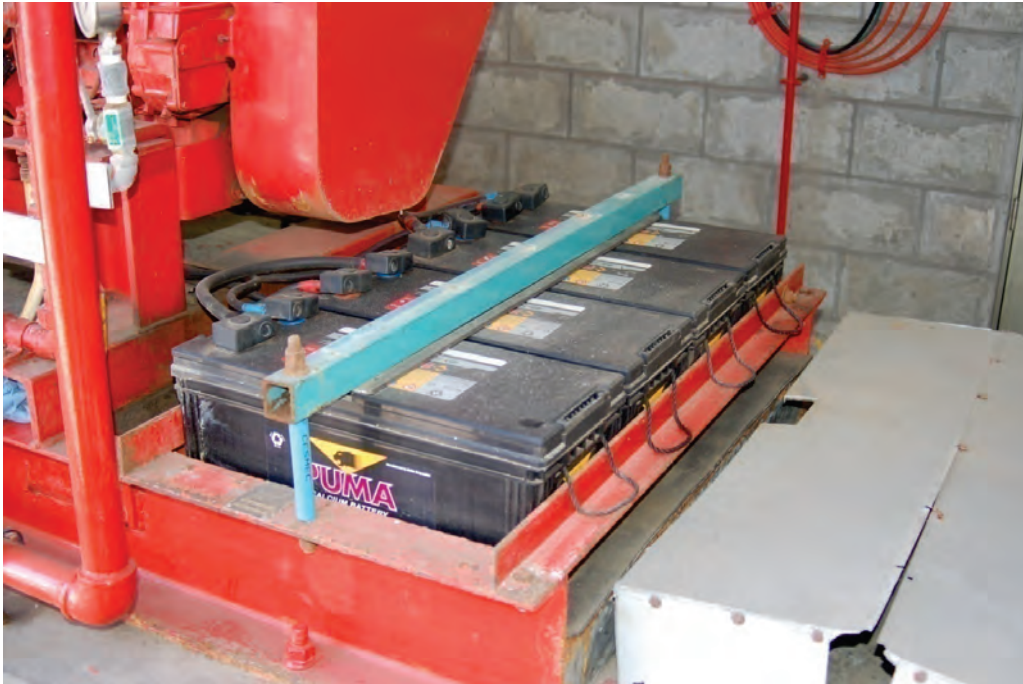
Figure 6.4.7.4-3 Batteries anchored with equipment skid (Photo courtesy of Eduardo Fierro, BFP Engineers).
