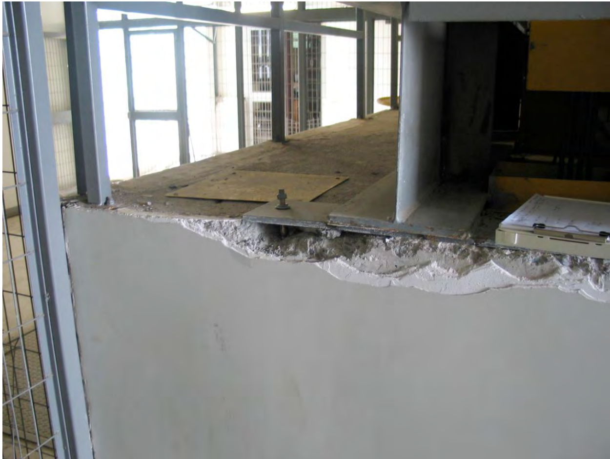
Figure 6.4.10.2-12 Anchor bolt failure of the elevator generator set due to inadequate edge distance for the bolts at the Los Angeles Regional Public Hospital in the 2010 Chile Earthquake (Photo courtesy of Bill Holmes, Rutherford & Chekene).
