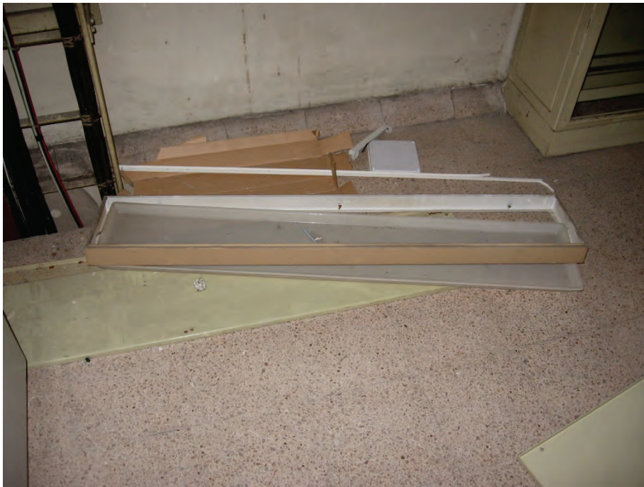
Figure 6.4.9.2-2 Overhead surface-mounted fixture anchored to underside of concrete slab damaged in the 2010 Chile Earthquake. Back of fixture housing remained anchored to the concrete slab above and the bulbs remained in place but the lens and sides of housing fell indicating that internal connections in the fixture were inadequate (Photos courtesy of Rodrigo Retamales, Rubén Boroschek & Associates).
