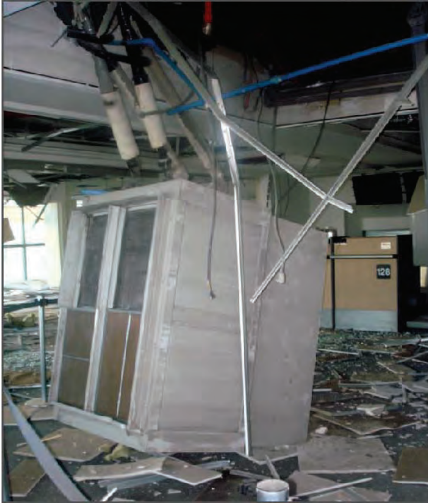
Figure 6.4.1.5-3 Suspended HVAC equipment came down at the Santiago airport terminal in the 2010 magnitude-8.8 Chile Earthquake (Photo courtesy of Gokhan Pekcan).
