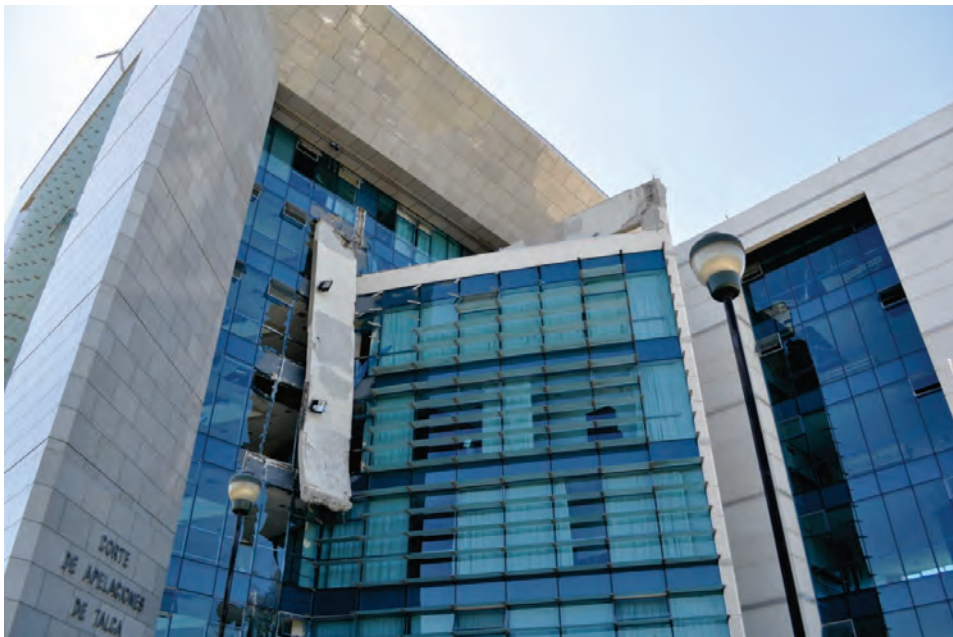
Figure 6.3.6.1-2 Reinforced concrete appendage dangling from connection on one side; impact damaged the curtain wall and created a serious hazard above the entrance of the Corte de Apelaciones de Talca in the 2010 magnitude-8.8 Chile Earthquake (Photo courtesy of Eduardo Fierro, BFP Engineers).
