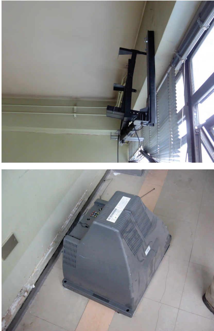
Figure 6.5.3.4-1 Wall-mounted monitor fell from the bracket in a hospital in the 2010 magnitude-8.8 Chile Earthquake; bracket still anchored to the wall (Photos courtesy of Rodrigo Retamales, Rubén Borosc hek & Associates)
