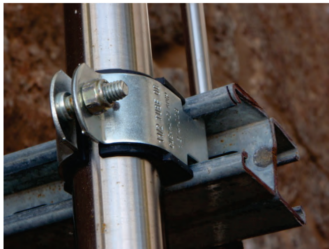
Figure 6.4.5.1-7 Process nitrogen piping outside engineering building on the UC Berkeley campus; strut clamp has rubber fittings to protect the stainless steel piping (Photos courtesy of Cynthia Perry, BFP Engineers).
