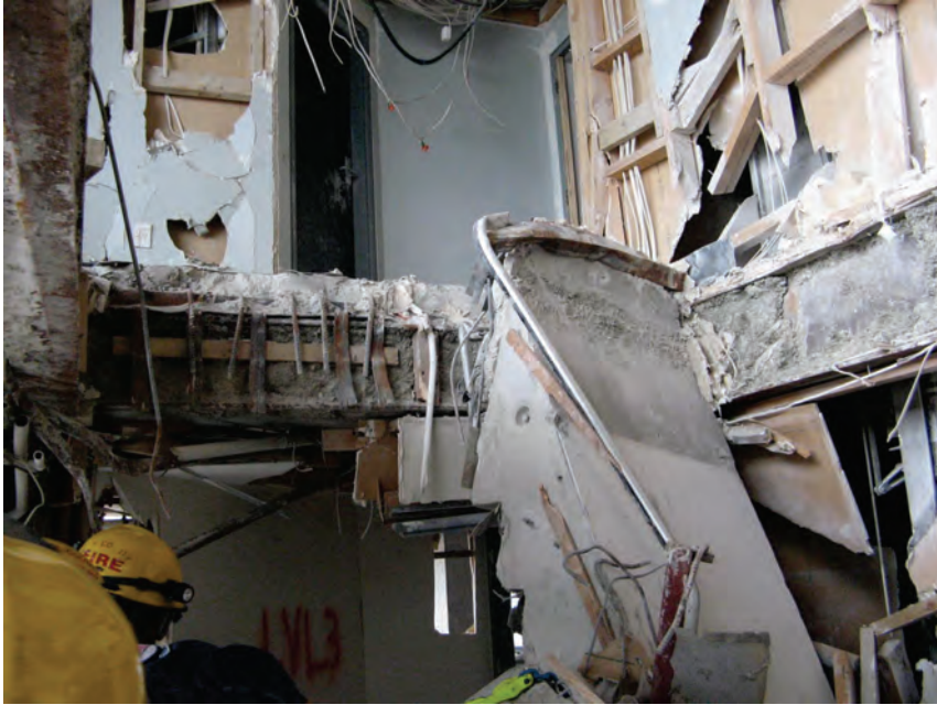
Figure 6.3.8.1-4 Stair support condition at Forsyth-Barr Building in Christchurch, New Zealand. Precast stair runs have completely pulled off supports and collapsed into stairwell (Photo courtesy of Des Bull, Holmes Consulting Group).
