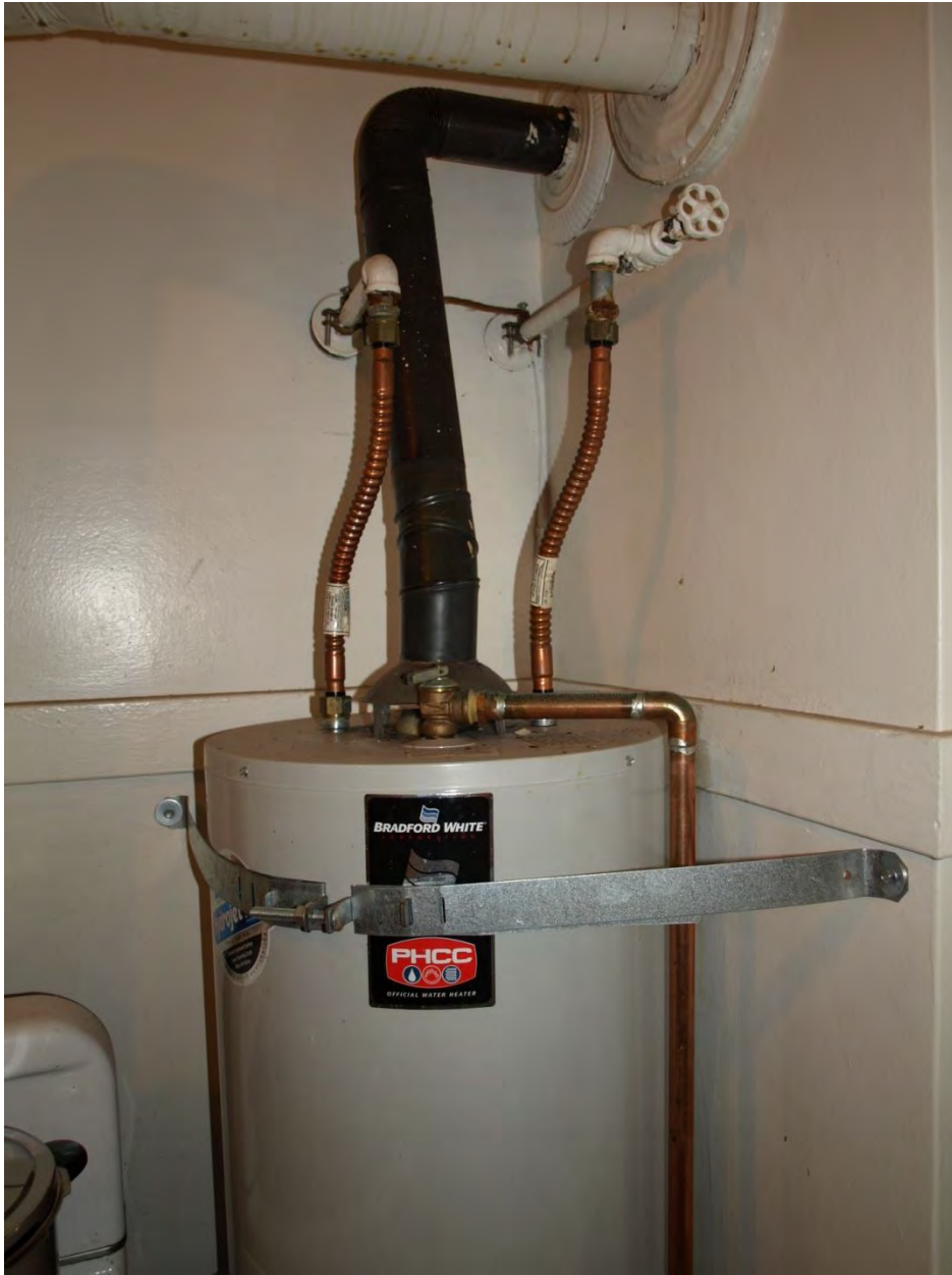
Figure 6.4.2.4-4 Corner installation using a commercially available strap; note flex copper tubing for water hook up (Photo courtesy of Cynthia Perry, BFP Engineers).
