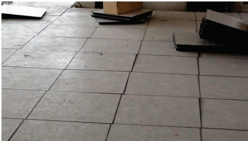
Figure 6.5.3.1-2 Damage to access floor with short anchored pedestals in the 2010 magnitude-6.7 Chile Earthquake; floor did not have lateral bracing. Note many tiles misaligned (Photos courtesy of Antonio Iruretagoyena, Rubén Boroschek & Associates).
