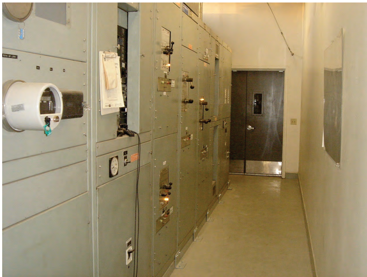
Figure 6.4.7.1-9 Anchorage for electrical cabinets. Anchorage to wall at top of cabinets is also present but not visible (Photo courtesy of Maryann Phipps, Estructure).
