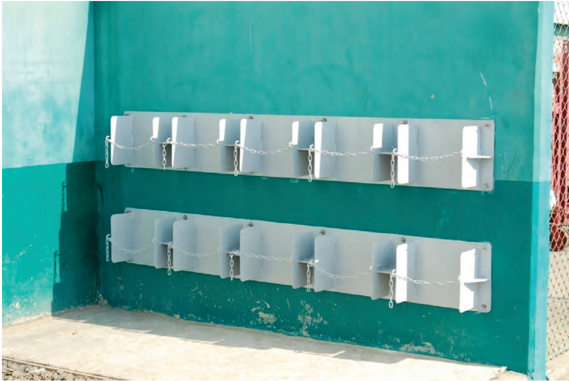
Figure 6.4.2.3-4 Wall-mounted cylinder restraints upgraded with stiffener plates following the 2001 Peru Earthquake (Photo courtesy of Eduardo Fierro, BFP Engineers).
