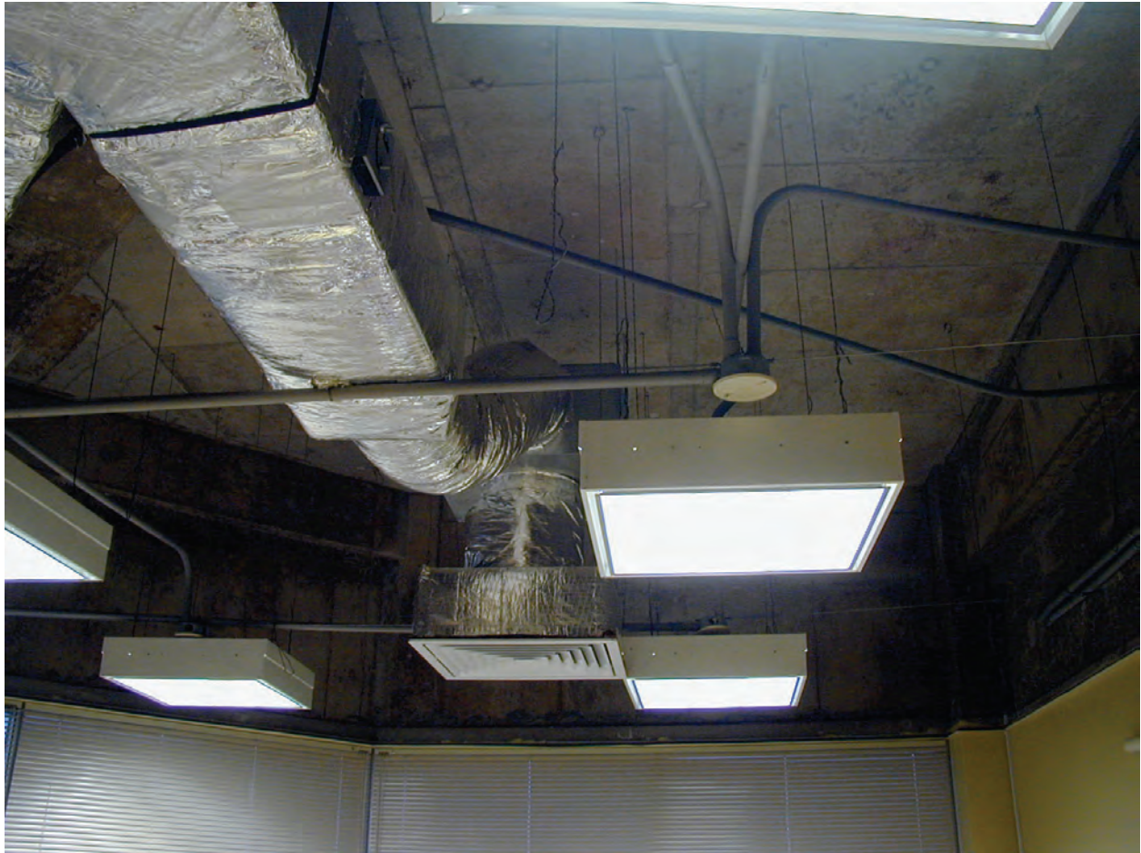
Figure 6.4.9.1-2 Overhead lights with four vertical hangers to the structure. Unbraced acoustic ceiling system was damaged beyond repair in the 2001 magnitude-8.4 Peru Earthquake but none of the diffusers or lights fell because they had independent supports. Ceiling was demolished prior to photo (Photo courtesy of Eduardo Fierro, BFP Engineers).
