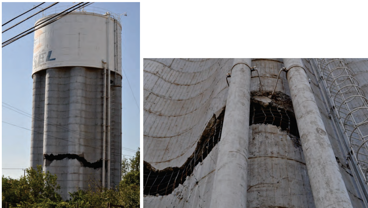
Figure 6.4.3.7-2 Pipe supports attached to wall of damaged silo (Photo courtesy of Eduardo Fierro, BFP Engineers). In spite of structural damage to silo, cast-in-place pipe supports were still intact and the piping did not fall.
