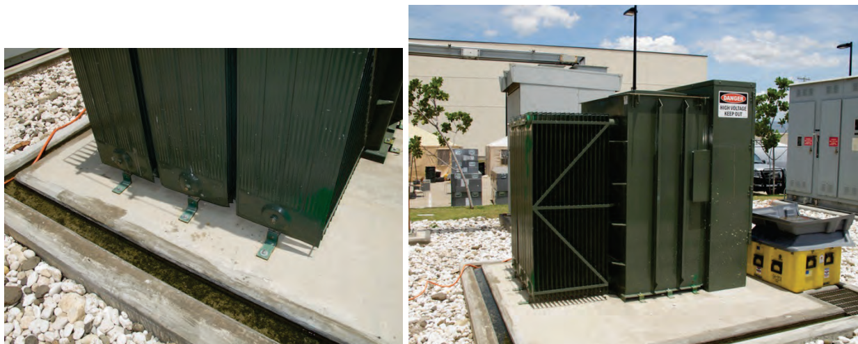
Figure 6.4.7.3-5 Outdoor liquid type electrical power transformer which converts incoming medium voltage to 480 volt utilization voltage for critical facility. Note use of manufacturer supplied diagonal elements on cooling fin assembly to minimize dynamic loading on liquid filled fin assembly which contains numerous welded connections. Post earthquake photo from the 2010 M 7.0 Haiti Earthquake (photos courtesy of Philip J. Caldwell).
