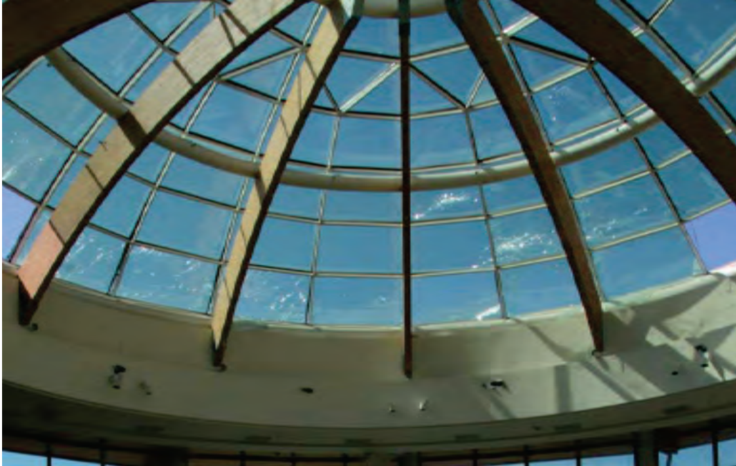
Figure 6.3.1.4-5 Overhead glazing damage from the 2010 Chile Earthquake (Photo courtesy of Eduardo Miranda, Stanford University).
