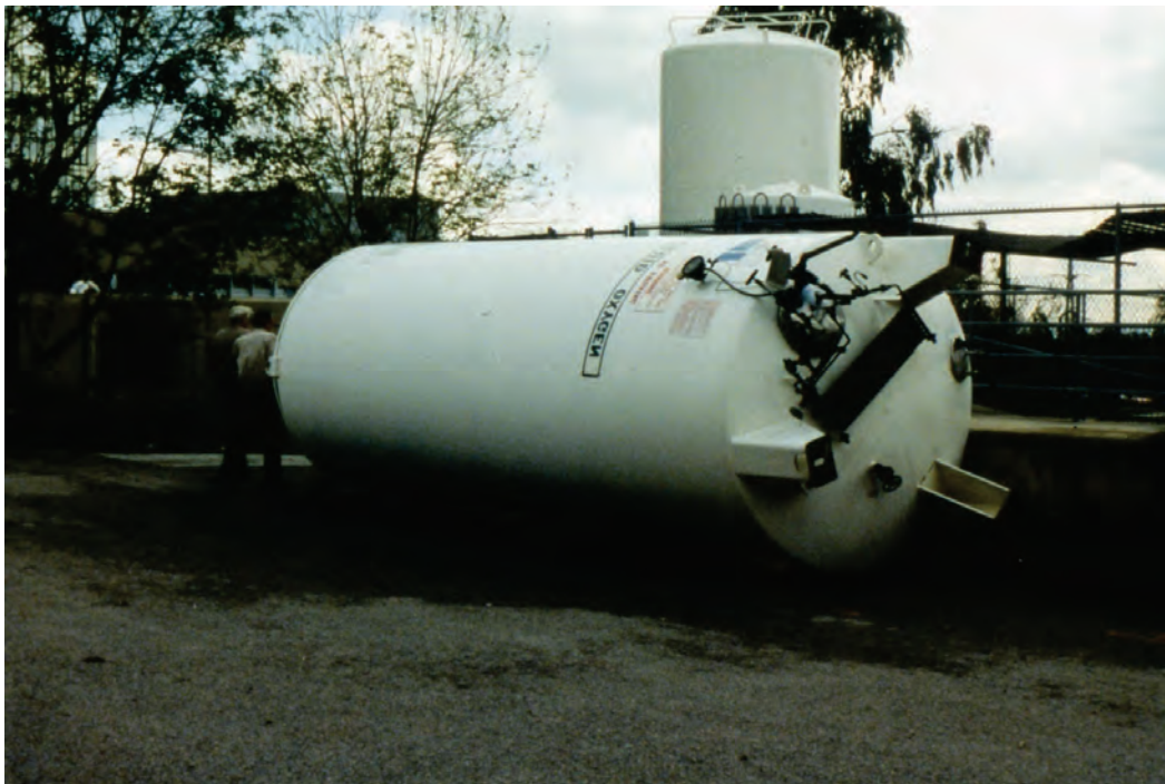
Figure 6.4.2.1-2 A vertical tank at hospital overturned due to inadequate anchorage in the 1994 Northridge Earthquake (Photo courtesy of OSHPD).
