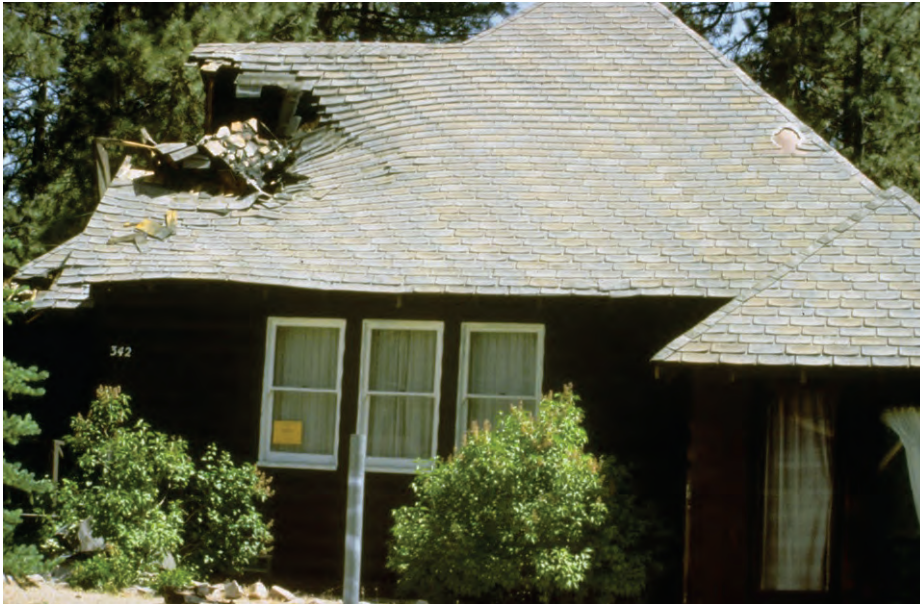
Figure 6.3.7.1-1 Chimney collapsed and fell through the roof; approximately 2,600 chimneys were destroyed in the 1992 Big Bear City, California earthquake (NGDC, 2009).
