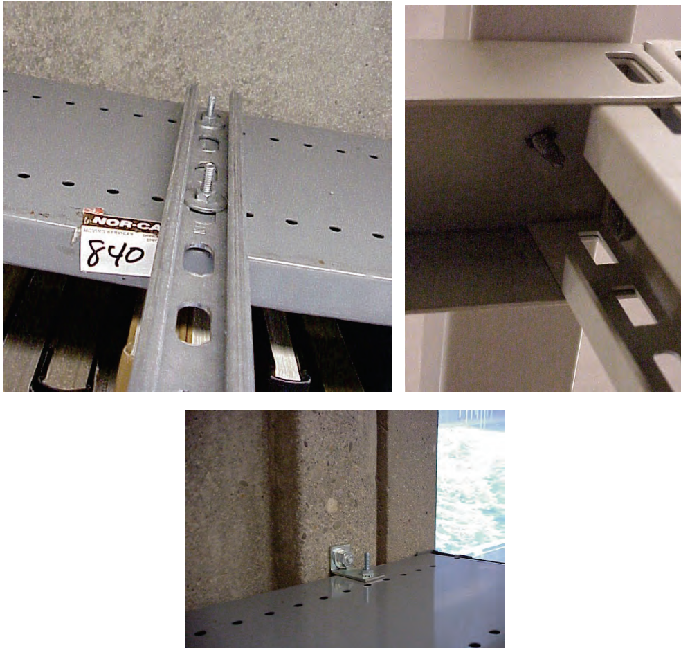
Figure 6.5.2.2-6 Examples of struts and hardware used to retrofit library shelving at the University of California, Berkeley (Photos courtesy of Mary Comerio, Dept. of Environmental Design, University of California Berkeley).
