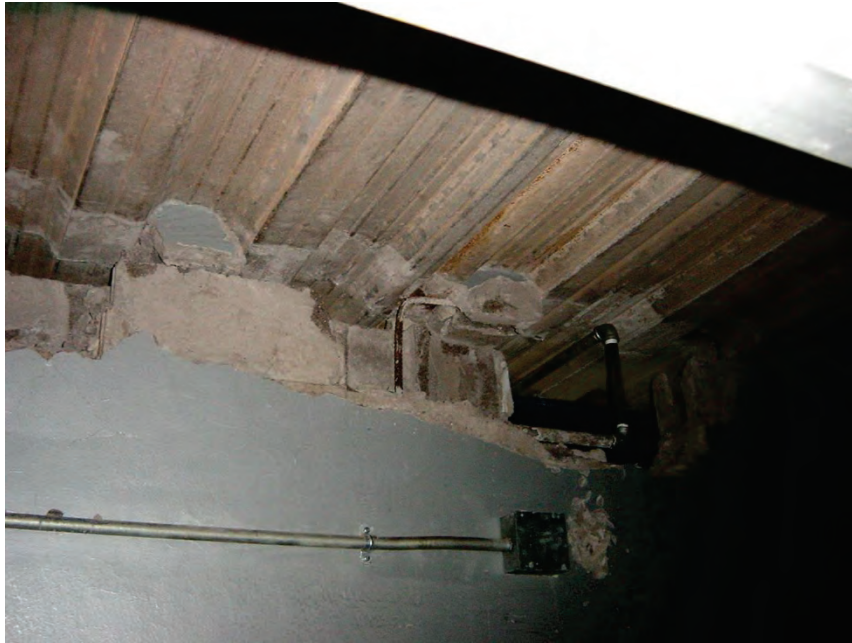
Figure 6.3.2.1-1 Damage along the top of a reinforced concrete masonry unit partition built flush with soffit of metal deck at an industrial facility in the 2001 magnitude-8.4 Peru Earthquake (Photo courtesy of Eduardo Fierro, BFP Engineers).
