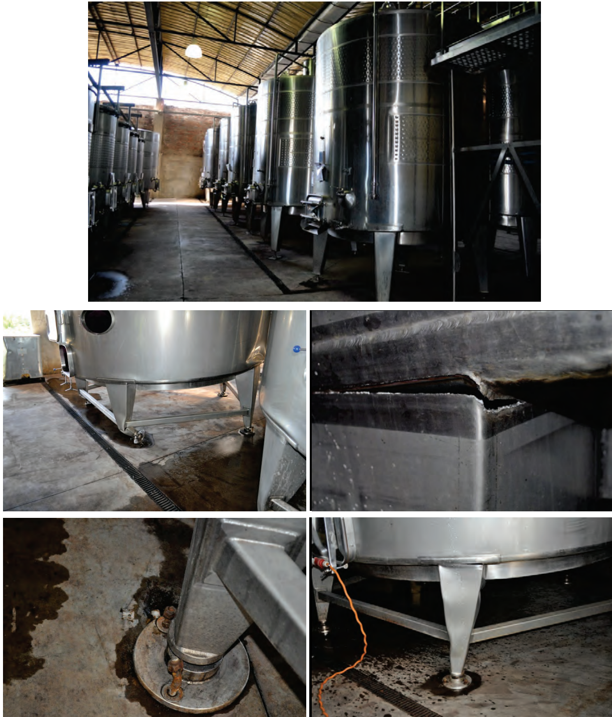
Figure 6.4.2.1-4 Wineries suffered extensive damage in the 2010 magnitude-8.8 Chile Earthquake with many barrels of wine spilled. This winery had damage to anchored tanks; tank anchorage failed, legs buckled, welds tore, anchor bolts pulled up, etc. The tank legs all have leveling bolts at the bottom, creating a weak zone between the bottom of the leg and the anchor plate. Similar unanchored tanks in this facility shifted position but were undamaged (Photos courtesy of Eduardo Fierro, BFP Engineers).
