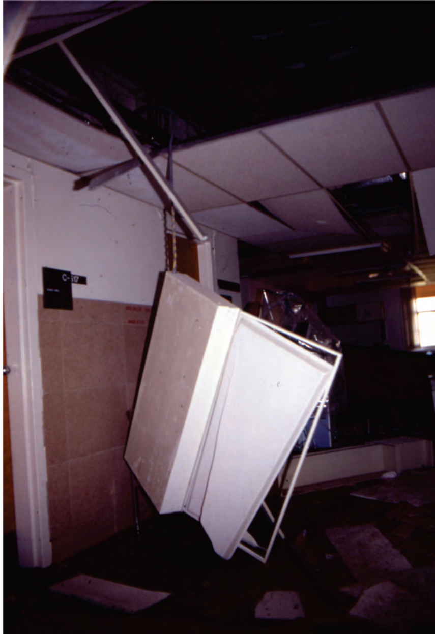
Figure 6.4.9.1-4 Light fixture without independent support dangling from conduit as a result of the 1994 Northridge Earthquake (Photo courtesy of Degenkolb Engineers).
