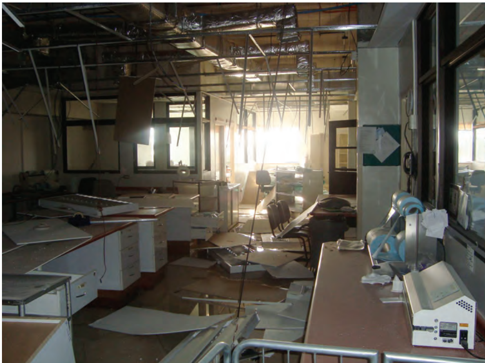
Figure 6.3.4.1-3 Generalized failure of ceiling grid, tiles, lights, and diffusers at the Los Angeles Hospital in the 2010 magnitude-8.8 Chile Earthquake (Photo courtesy of Bill Holmes, Rutherford & Chekene).
