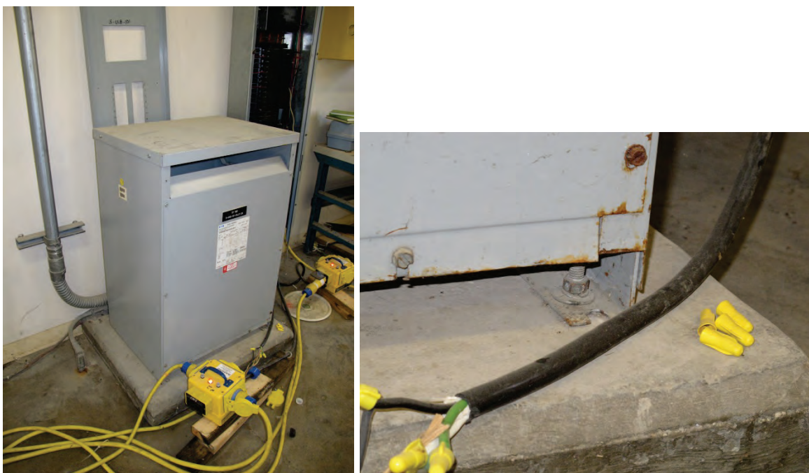
Figure 6.4.7.3-2 Typical electrical distribution dry type transformer. Note the use of manufacturer supplied anchor locations on base channels. Post earthquake photo from the 2010 Haiti M 7.0 Earthquake (photos courtesy of Philip J. Caldwell).
