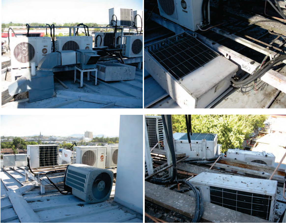
Figure 6.4.1.4-3 Numerous poorly anchored rooftop units toppled in the 2010 Chile Earthquake (Photos courtesy of Rodrigo Retamales, Rubén Boroschek & Associates).
