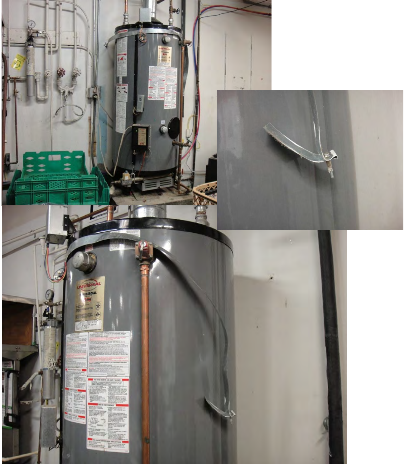
Figure 6.4.2.4-3 Damaged water heater in the 2010 magnitude-6.5 Eureka Earthquake. The water heater strap pulled out from the supporting concrete wall as a result of inadequate anchorage. The tank moved sufficiently to break interconnected water lines which were rigidly connected to the tank.
