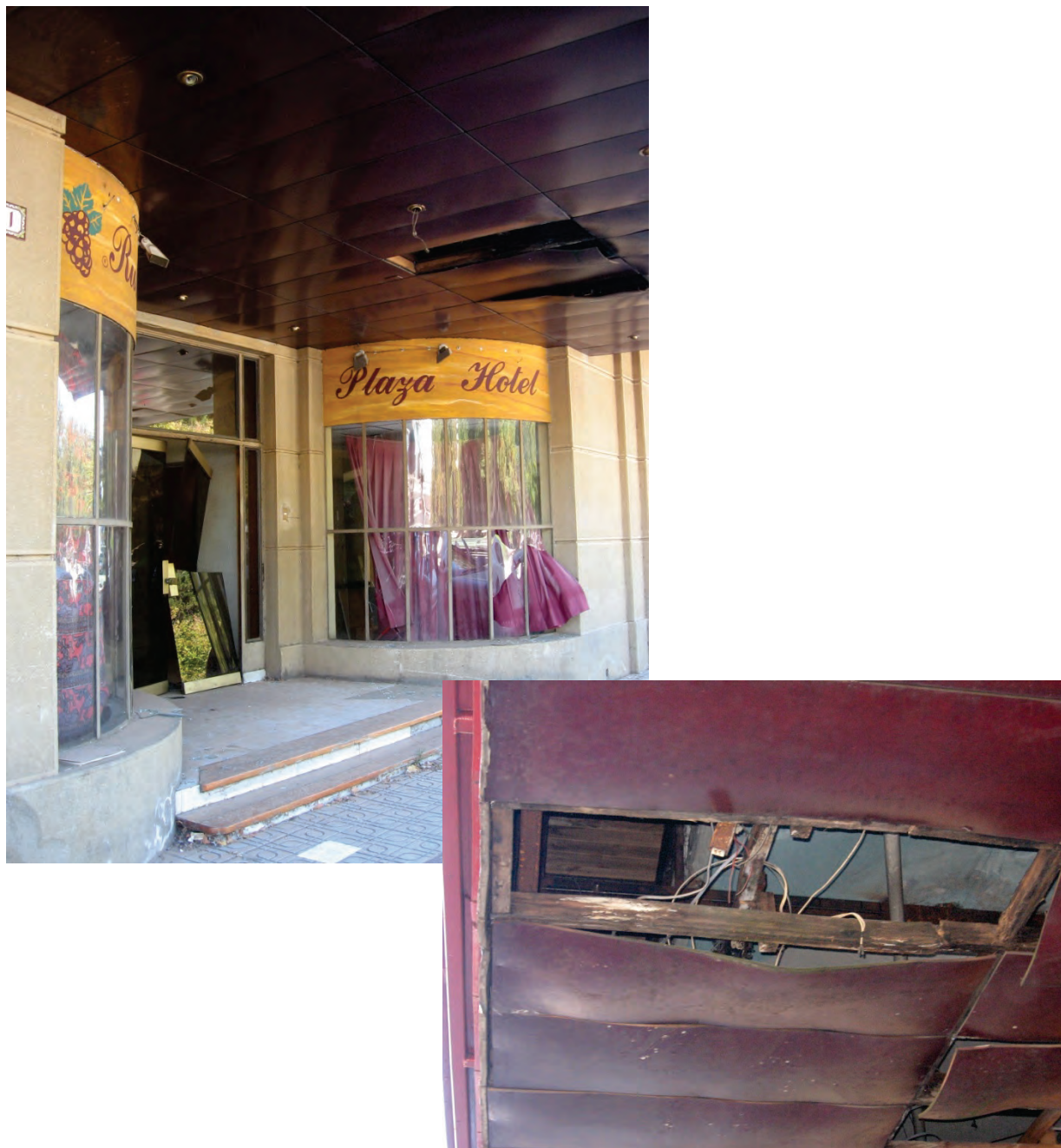
Figure 6.3.4.2-3 Damage to soffit paneling and wood framing at hotel in the 2010 Chile Earthquake; panels and wood framing show signs of prior water damage and deterioration. Note also damage to storefront glazing and glass doors (Photos courtesy of Rodrigo Retamales, Rubén Boroscchek & Associates).
