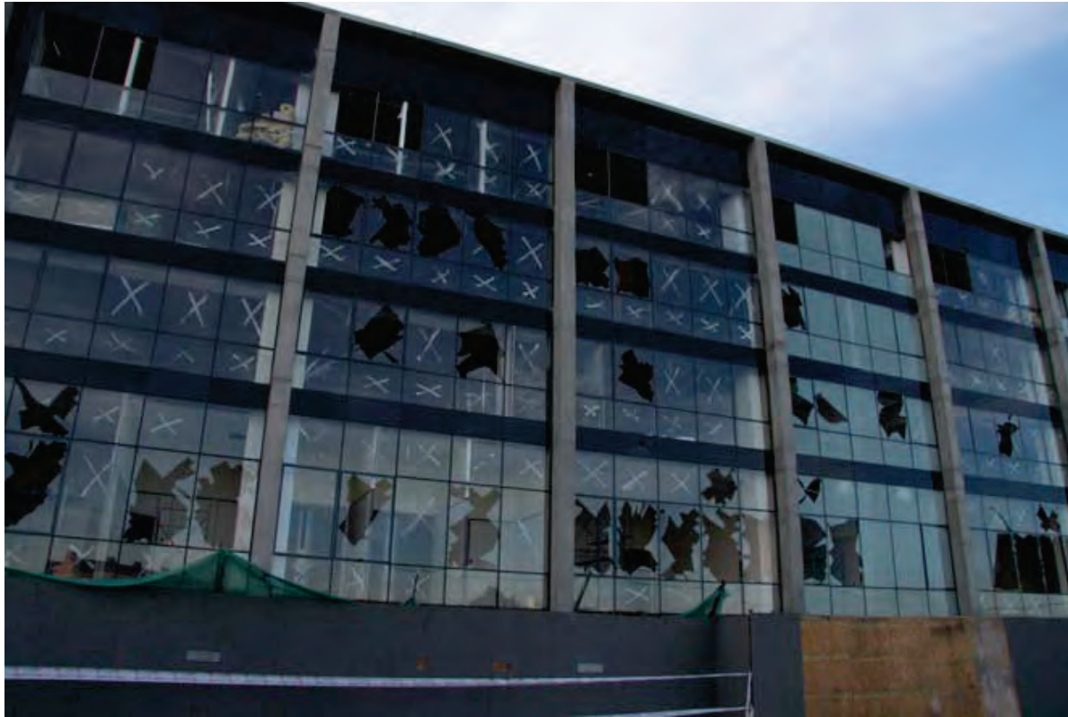
Figure 6.3.1.4-3 Glazing damage was observed in many residential and commercial buildings and hospitals throughout central Chile following the 2010 magnitude-8.8 Chile Earthquake (Photo courtesy of Eduardo Miranda, Stanford University).
