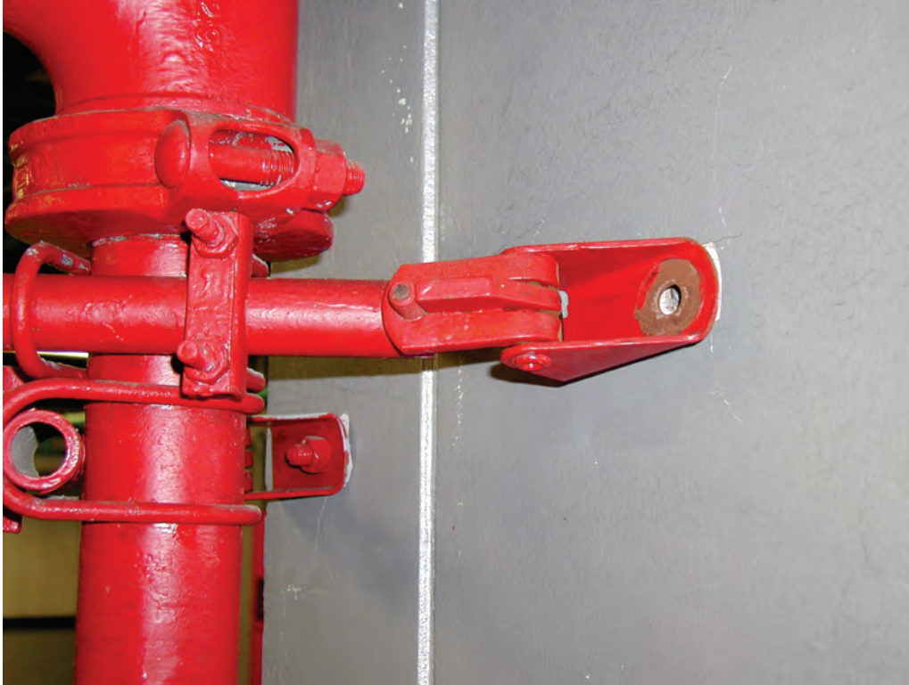
Figure 6.4.4.1-2 Wall-mounted pipe restraint failed due to inadequate connection to structural framing in the 2001 magnitude-8.4 Peru Earthquake (Photo courtesy of Eduardo Fierro, BFP Engineers).
