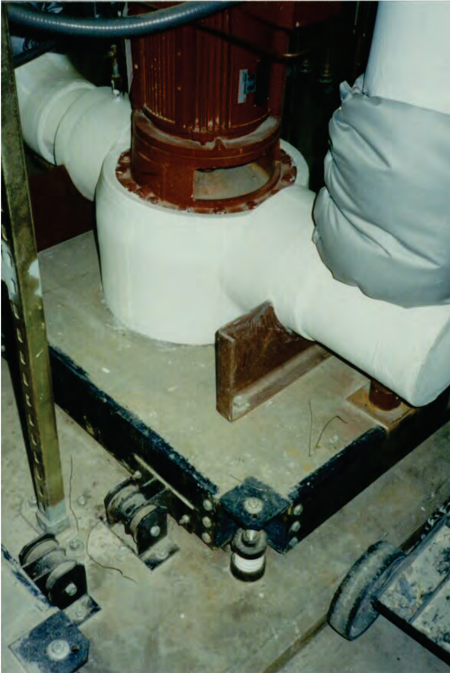
Figure 6.4.3.2-1 In-line pump mounted on independent concrete inertia pad with vibration isolation and seismic snubbers (Photo courtesy of Mason Industries).
