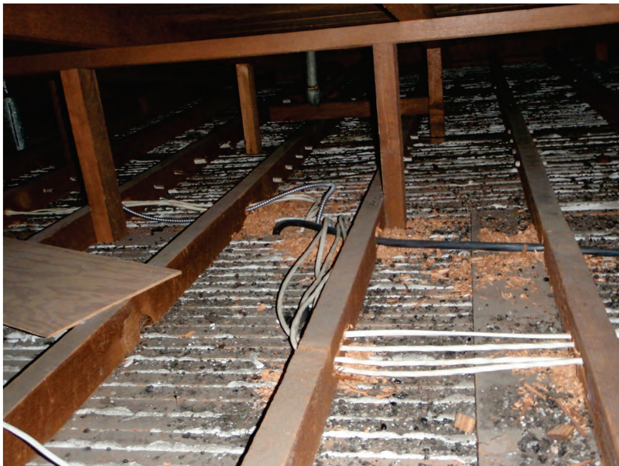
Figure 6.3.4.2-7 View of typical wood lath and plaster ceiling from the 1920's from above (Photo courtesy of Cynthia Perry, BFP Engineers). The wood lath is well nailed to the underside of the ceiling joists. This type of ceiling typically remains intact during an earthquake but may require crack repair and painting. Where the plaster has delaminated from the lath due to age or water leakage, wood strips could be installed from below as in Figure 6.3.4.2-8.
