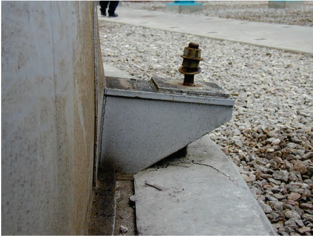
Figure 6.4.2.2-1 Damage to ductile connection at base of a 5000 cubic meter diesel fuel tank in the 2001 magnitude-8.4 Peru Earthquake. All eight connections were damaged; damage included bolt elongation, deformation of tank wall, and cracked concrete pad (Photo courtesy of Eduardo Fierro, BFP Engineers).
