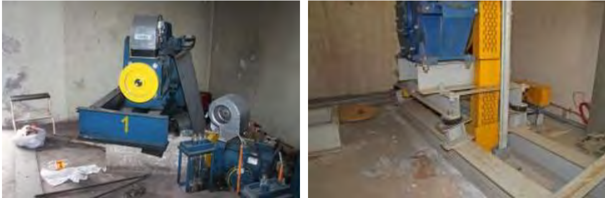
Figure 6.4.10.2-4 Examples of damage to elevator machines produced by inadequate anchorage to the structure (Photos courtesy of Eduardo Miranda, Stanford University).
