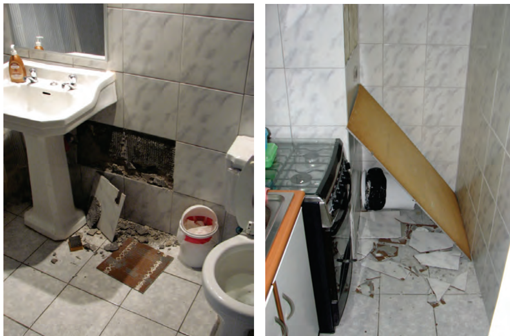
Figure 6.3.3.1-1 Damage to adhered tile veneer in residential bathroom and kitchen in the 2010 magnitude-8.8 Chile Earthquake (Photo courtesy of Antonio Iruretagoyena, Ruben Boroschek & Associates). Tile is adhered to CMU infill partitions.
