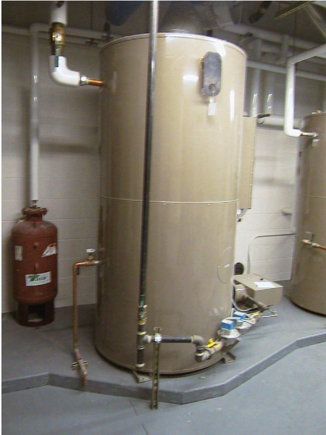
Figure 6.4.2.4-5 Base-mounted water heater located in a school; equipment supplied with metal base for mounting (Photo courtesy of EQE for the Salt Lake City School District).
