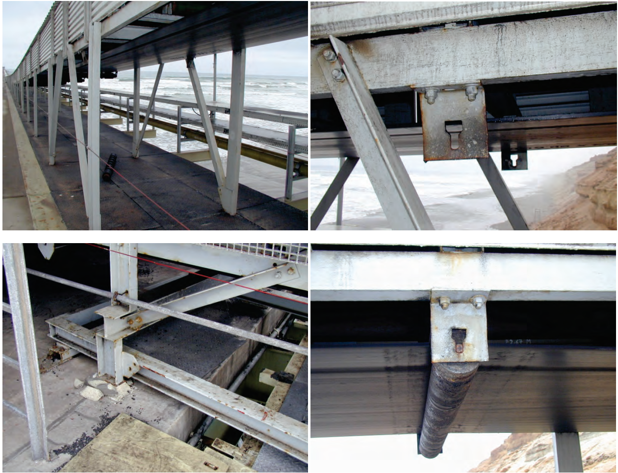
Figure 6.4.11.1-3 Damage to industrial coal conveyor on jetty in southern Peru in the 2001 magnitude-8.4 Peru Earthquake (Photos courtesy of Eduardo Fierro, BFP Engineers). Conveyor was well anchored along entire length but detailing at the seismic joint between the jetty and platform did not allow sufficient movement, resulting in misalignment at end of conveyor and damage to the supports as shown at lower left. Approximately 10% of the rollers fell; these were held in place with friction fittings and did not have positive connections.
