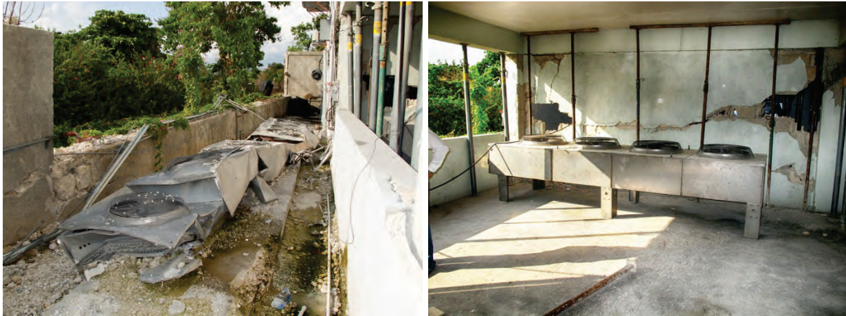
Figure 6.4.7.3-7 Heat rejection mechanical units which provide cooling for servers in cellular carrier central network facility (left photo). Collapsing security wall during the 2010 M 7.0 Haiti Earthquake crushed these units and resulted cyclical total failure of the cellular network as the servers hit temperature limits, shut down, rebooted and heated up again. System stability was restored by replacing the damaged units with temporary ones (right photo). Example of how the reliability of a critical facility essential system is both dependent upon adequate seismic restraints and a location which is free of structural and nonstructural falling hazards (photos courtesy of Philip J. Caldwell).
