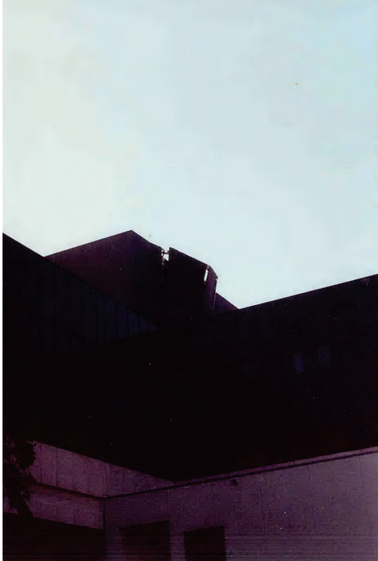
Figure 6.3.1.3-2 Precast panel failure at the top floor of a hospital in the 1994 magnitude-6.7 Northridge Earthquake (Photo courtesy of OSHPD).
