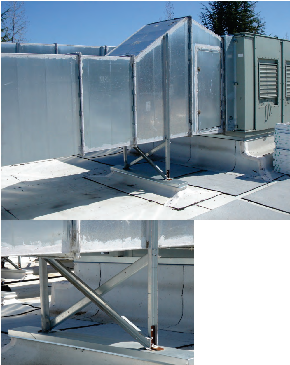
Figure 6.4.6.1-6 Roof-mounted rectangular duct supported on braced support stand built up from steel channels (Photo courtesy of Maryann Phipps, Estructure).
