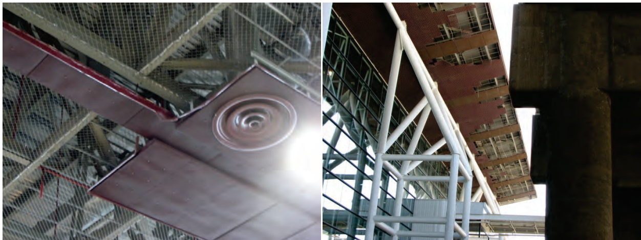
Figure 6.3.4.2-5 Extensive failure of ceiling in the main terminal of the Santiago airport in the 2010 Chile Earthquake. Metal panels with lights and diffusers hung from furring on short metal tabs; these remained in place but detail at lower left shows they also sustained some damage. Furring channels still in place throughout ceiling but majority of lightweight ceiling panels and much of the cross furring came down as shown at lower right photo of exterior soffit with same system (Photos courtesy of Antonio Iruretagoyena, Rubén Boroscchek & Associates).
