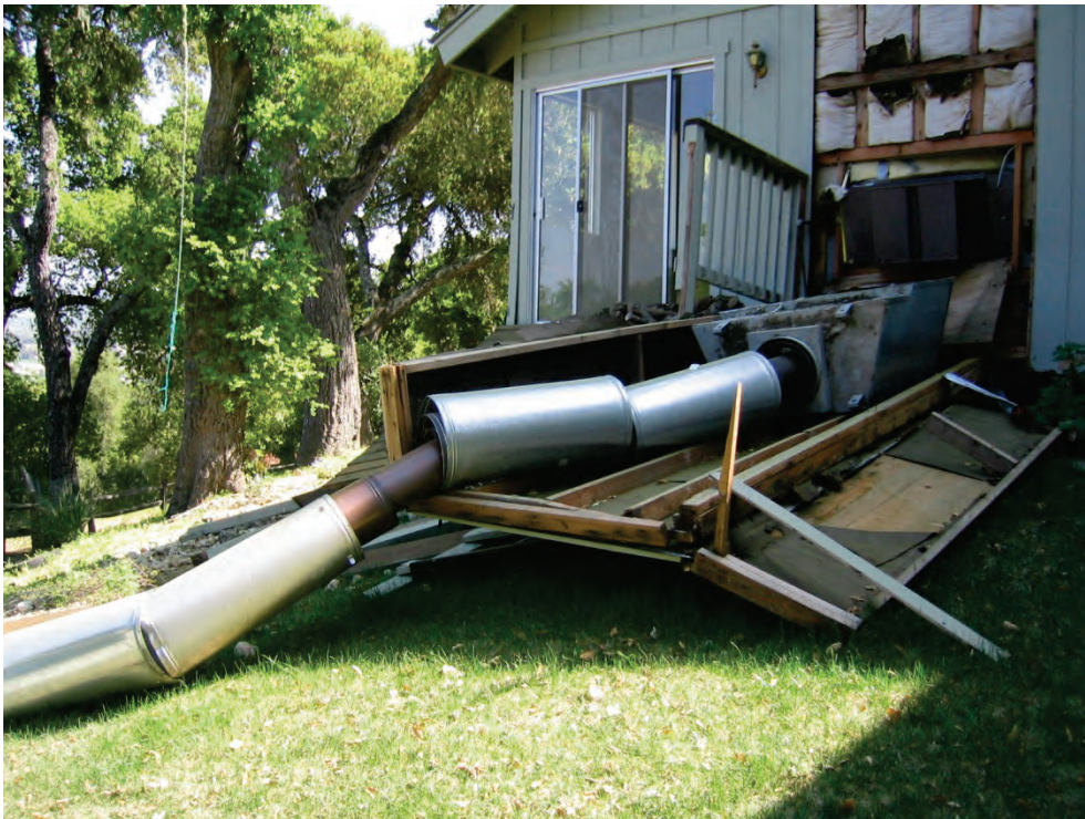
Figure 6.3.7.1-2 Residential metal flue in wood frame chimney that failed in the 2003 magnitude-6.5 San Simeon earthquake. The house fell off its cripple wall, pushing over the chimney (Photo courtesy of Michael Mahoney).
