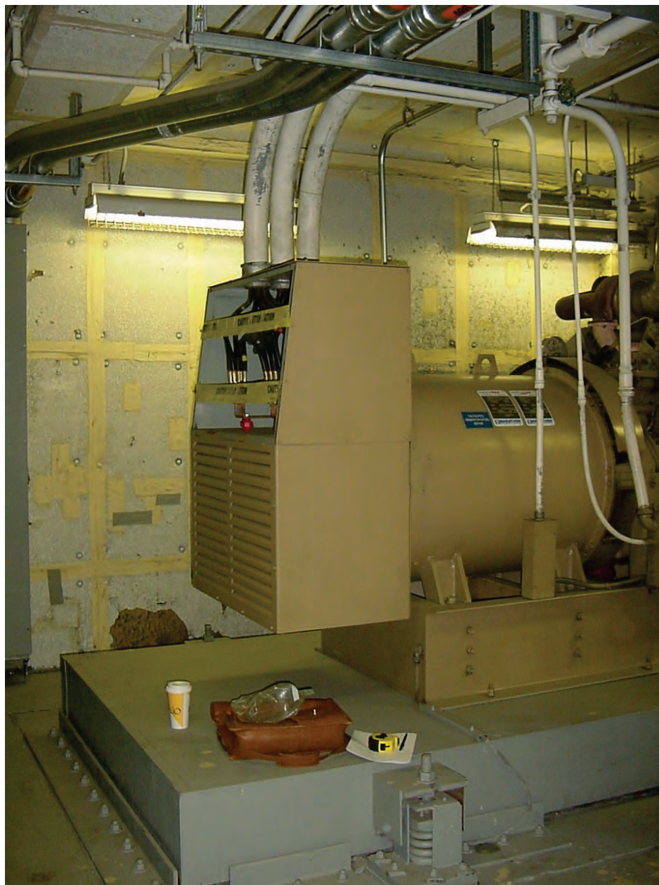
Figure 6.4.7.2-1 Emergency generator is anchored to a concrete inertia base. The inertia base is mounted on spring isolators and restrained by steel angle snubbers on all sides (Photo courtesy of Maryann Phipps, Estructure).
