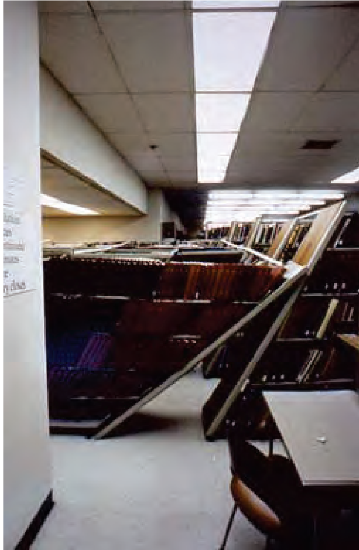
Figure 6.5.2.2-3 Longitudinal failure of library shelving units (Photo courtesy of NISEE-PEER, U.C. Berkeley). Transverse ties used to tie units together but this was not enough to prevent longitudinal failure.
