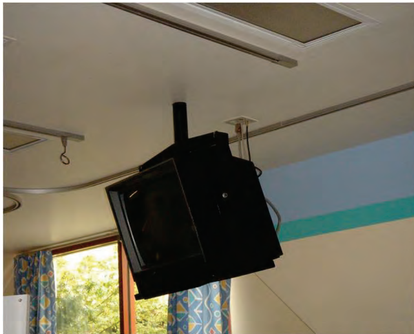
Figure 6.5.3.4-3 Mounting plate above ceiling for overhead television bracket in a hospital room. Television or monitor must be securely attached to the bracket (Photos courtesy of Maryann Phipps, Estructure).
