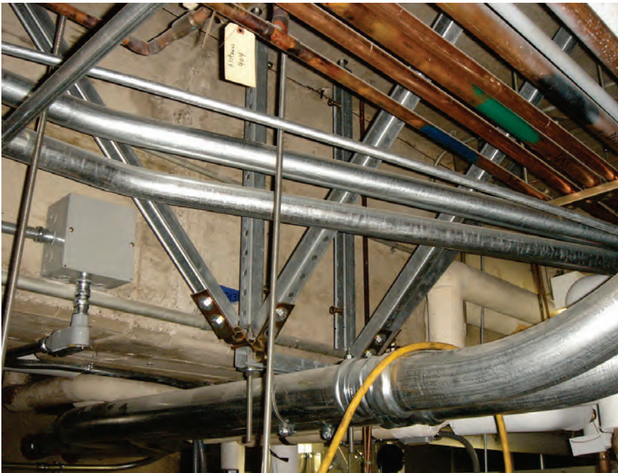
Figure 6.4.8.1-3 Rigid strut bracing for trapeze supporting electrical conduit; conduit attached to trapeze with conduit clamp that provides lateral and longitudinal restraint (Photo courtesy of Maryann Phipps, Estructure).
