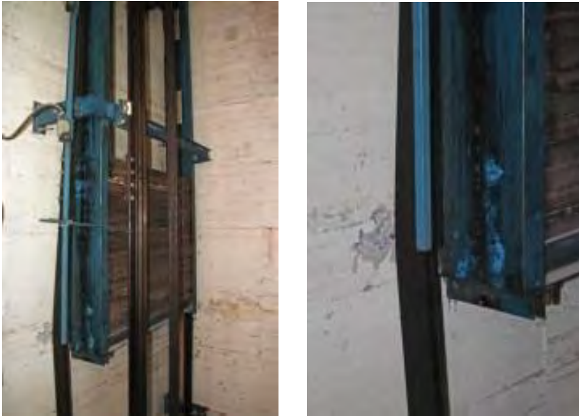
Figure 6.4.10.2-7 Damage to guide rails caused by derailment of the counterweight in a hospital in Chillan during the 2010 Chile earthquake (Photos courtesy of Eduardo Miranda, Stanford University).
