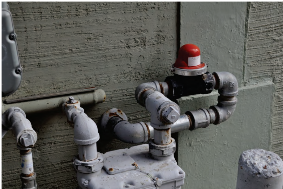
Figure 6.4.5.1-8 Two examples of seismic shut-off valves in San Francisco Bay Area. Top photo at Marine Mammal Center; lower photo at six unit apartment building in Oakland (Photos courtesy of Cynthia Perry, BFP Engineers).
