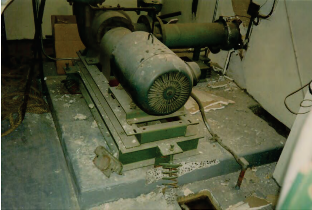
Figure 6.4.1.3-2 Failure of pump mounted on three vibration isolators and damage at wall penetration (Photo courtesy of Mason Industries).
