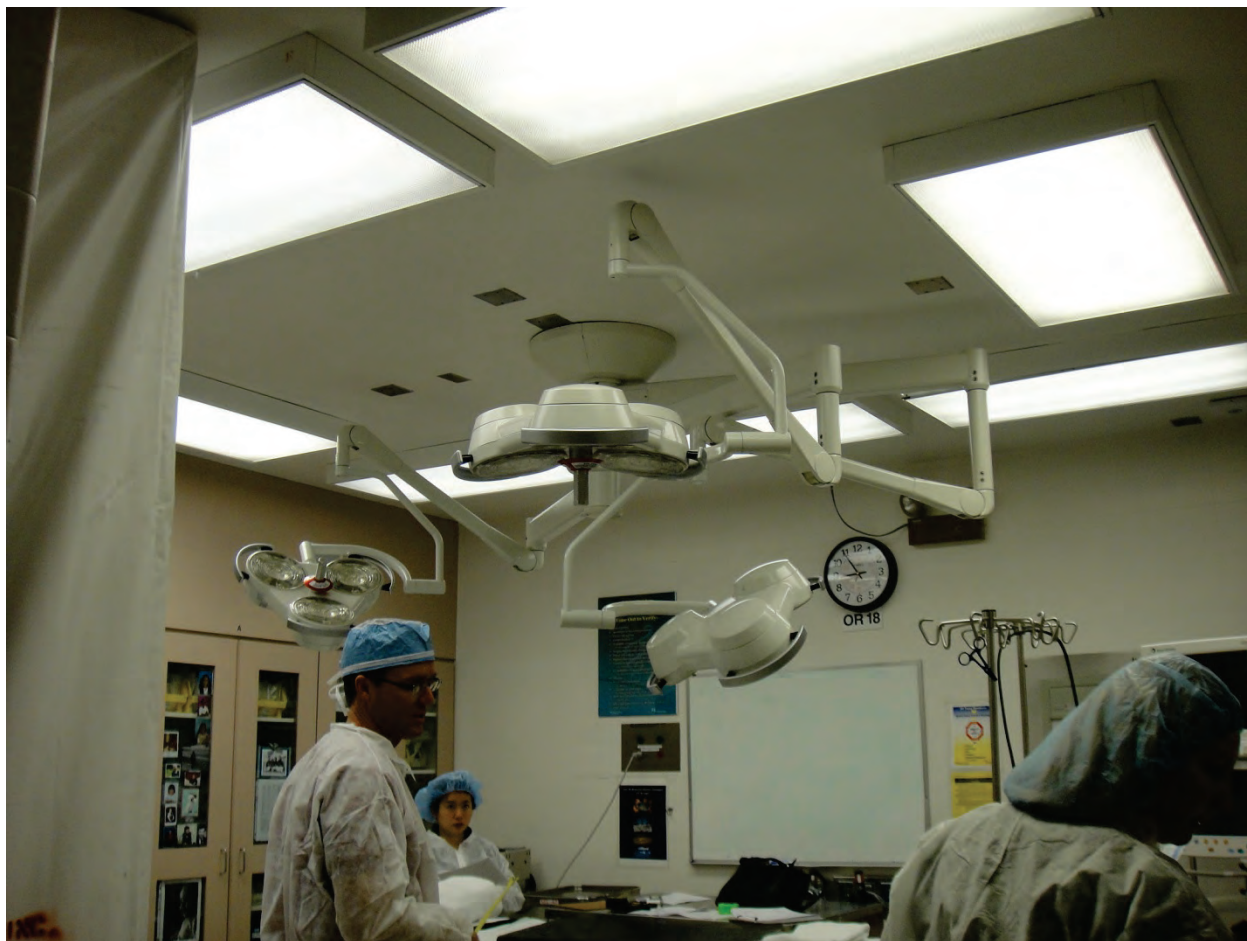
Figure 6.4.9.4-2 Engineered support and bracing are required for heavy operating room lights. The arms, joints, lenses and bulbs must be capable of resisting seismic forces. Hospital fixtures require certification. Photo also shows surface mounted fluorescent fixtures in a suspended gypsum board ceiling; each of these requires independent safety wires to the structure above; see Section 6.4.9.2 (Photo courtesy of Maryann Phipps, Estructure).
