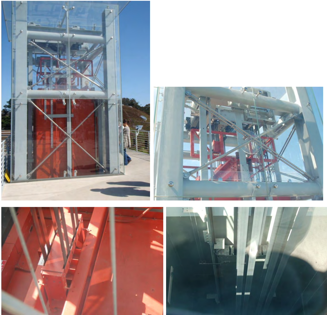
Figure 6.4.10.2-13 Small “machine-roomless” traction elevator with flat belts at the Academy of Sciences, San Francisco, California (Photos courtesy of Eduardo Fierro, BFP Engineers). Clockwise: Overview of elevator at roof; view of guide rails and sheaves; top of cab showing belts; view down shaft at belts, counterweight, guide rails and guide rail brackets.
