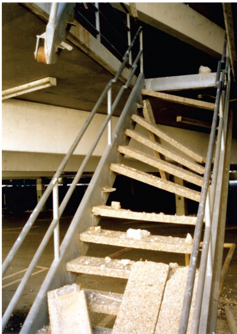
Figure 6.3.8.1-1 Stairway damaged by drift in the 1994 magnitude-6.7 Northridge, California earthquake (Photo courtesy of Wiss, Jenney, Elstner Associates).
