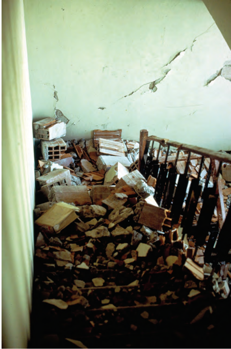
Figure 6.3.2.1-4 View of stairway in the Banco Central Building, Managua, Nicaragua after the 1972 magnitude 6.2 Managua Earthquake. Most of the stairs were covered with debris that resulted from the failure of the hollow tile partitions surrounding the stairs (Photo courtesy of PEER Godden Collection, No. J94).
