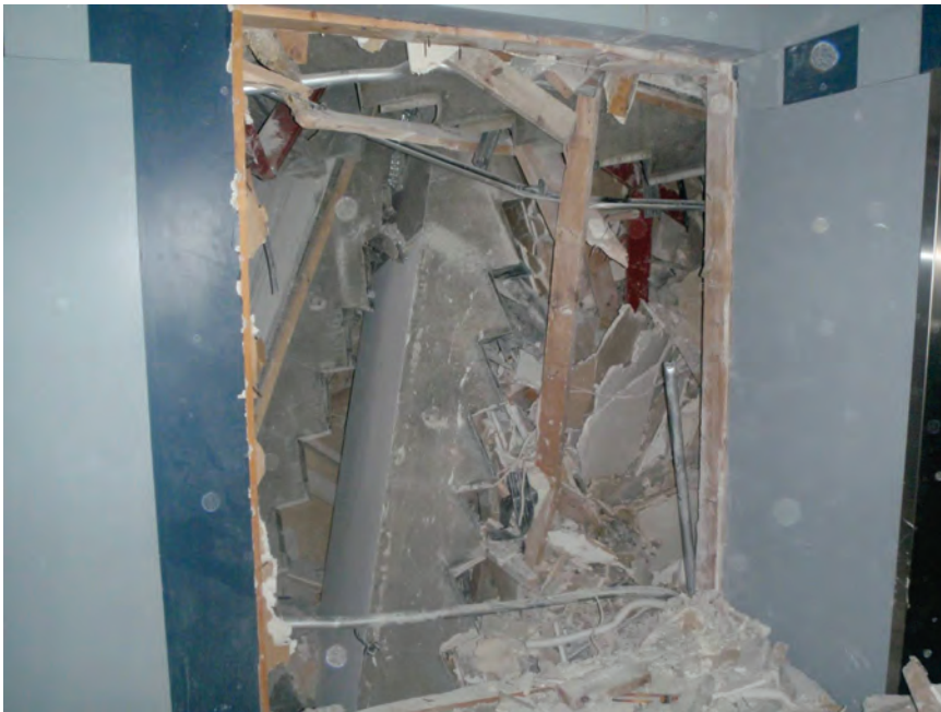
Figure 6.3.8.1-5 One story precast stair units stacked up at base of stairwell after falling off the sliding end supports and collapsing into stairwell (Photo courtesy of Des Bull, Holmes Consulting Group).
