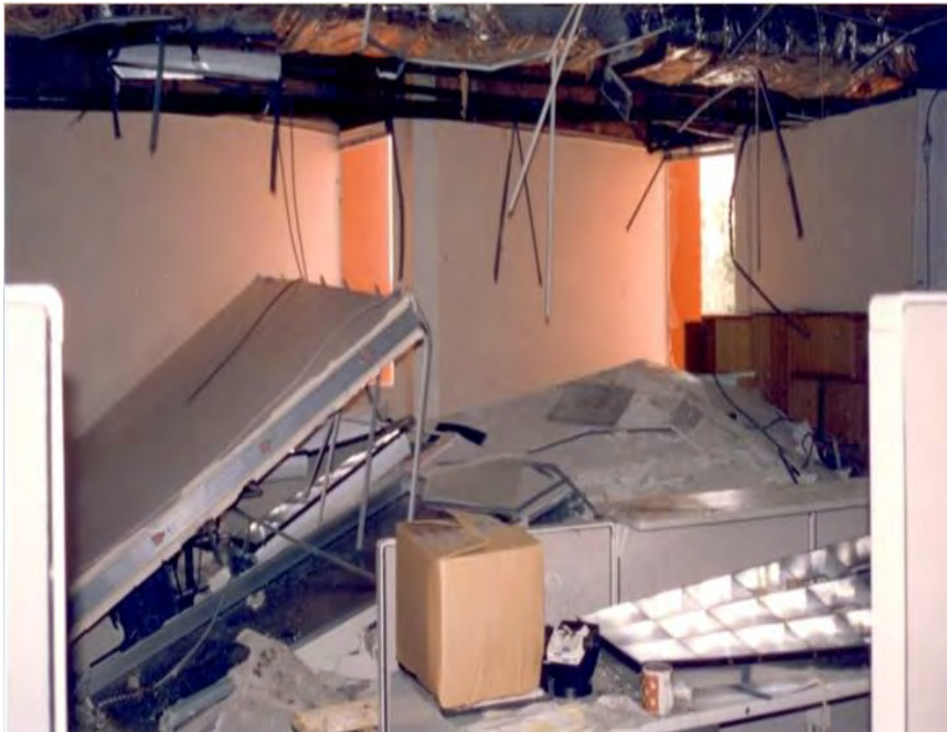
Figure 2.4.1-1 Failure of office partitions, ceilings, and light fixtures in the 1994 Northridge Earthquake (FEMA 74, 1994).
