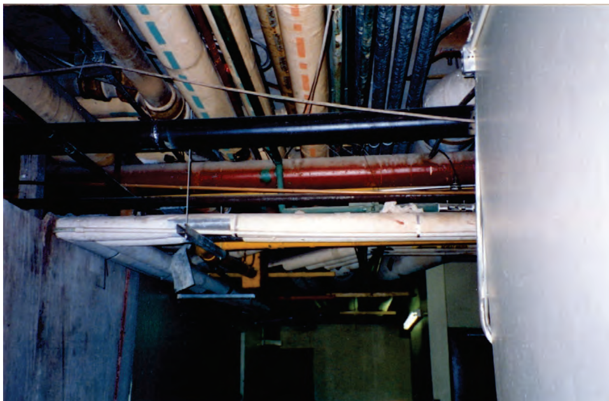
Figure 6.4.8.1-1 Unbraced suspended piping and conduit (Photo courtesy of Wiss, Janney, Elstner Associates).
