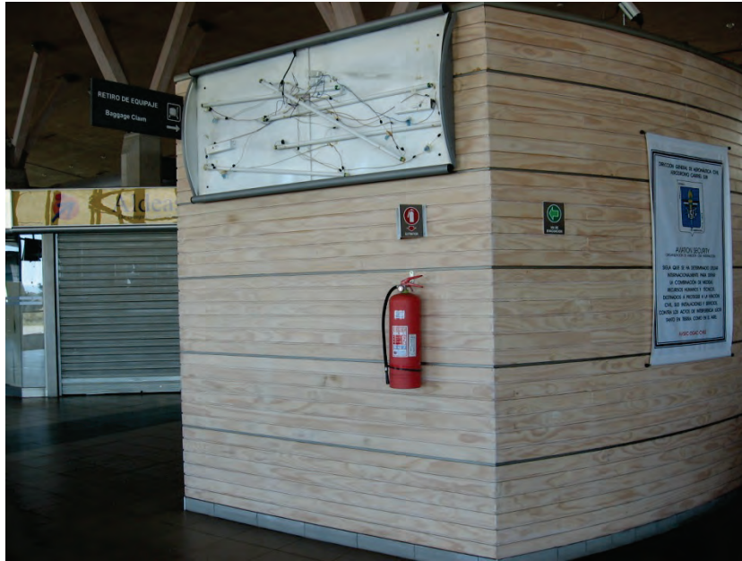
Figure 6.4.9.2-1 Numerous failures of ceilings and lights were observed at the Concepción airport in the 2010 magnitude-8.8 Chile Earthquake. Photo shows surface-mounted fixture on wall that remained in place but the lens fell and the bulbs were dislodged (Photo courtesy of Rodrigo Retamales, Rubén Boroschek & Associates).
