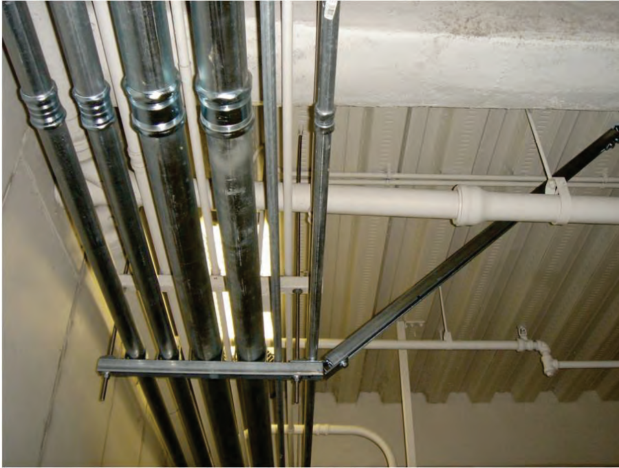
Figure 6.4.8.1-2 Rigid strut bracing provides restraint against earthquake forces perpendicular to the piping. Similar bracing is required in the direction parallel to the conduit (Photo courtesy of Maryann Phipps, Estructure).
