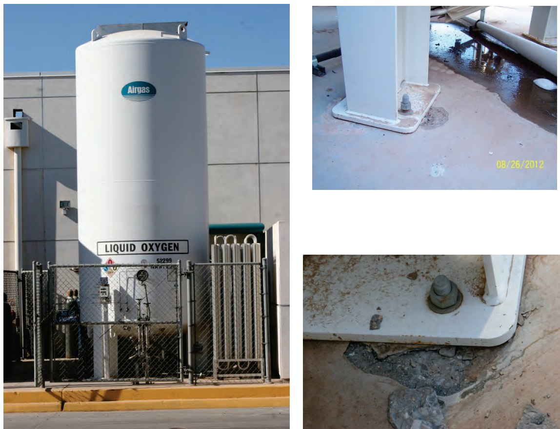
Figure 6.4.2.1-5 Damage to tanks at the Pioneer Memorial Hospital at the 2012 Brawley Earthquake (Photo courtesy of Chris Tokas, OSHPD)
