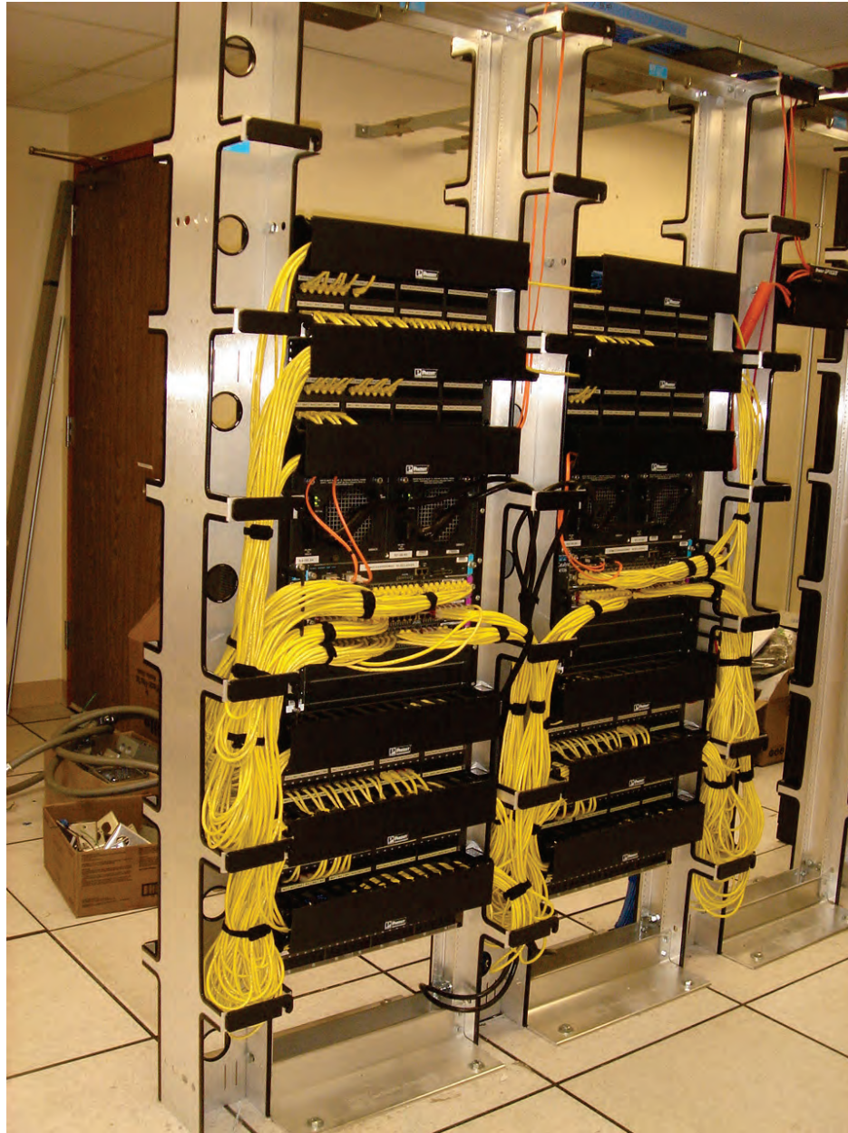
Figure 6.5.3.1-5 Data rack bolted through access floor to supplemental strut bracing below (Photo courtesy of Maryann Phipps, Estructure).
