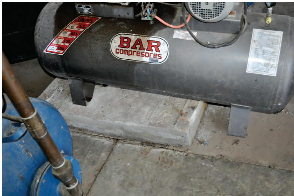
Figure 6.4.1.4-1 Poorly anchored compressor jumped off the undersized anchor bolts in the 2010 magnitude-8.8 Chile Earthquake (Photo courtesy of Eduardo Fierro, BFP Engineers).
