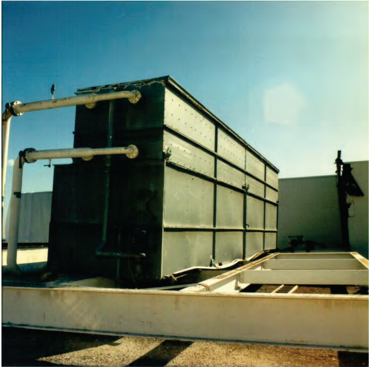
Figure 6.4.1.3-4 Rooftop equipment on isolators collapsed onto skid (Photo courtesy of Mason Industries).
