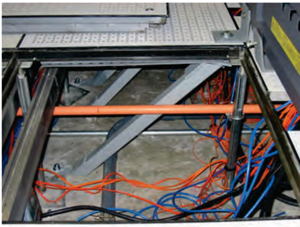
Figure 6.5.3.1-4 Raised floor braced with strut (Photo courtesy of Maryann Phipps, Estructure).
