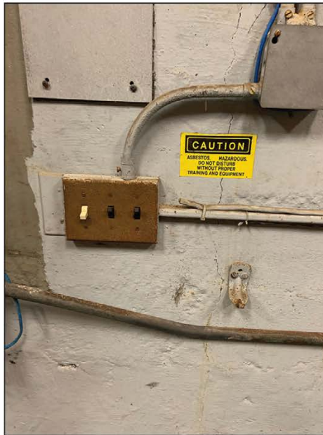
An asbestos warning posted in a school in Michigan.
