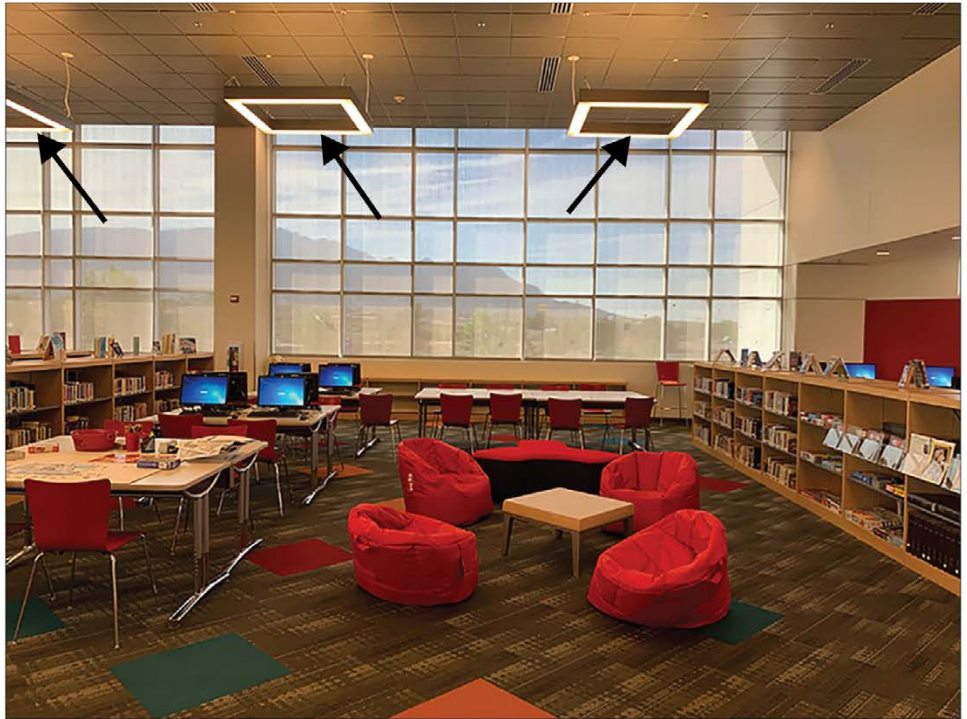
Energy efficient lighting in a New Mexico school
