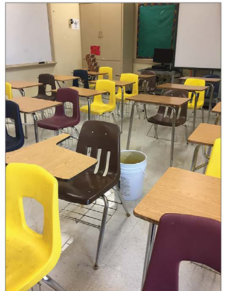
Bucket full of water in the middle of a Florida classroom with a roof leak.
