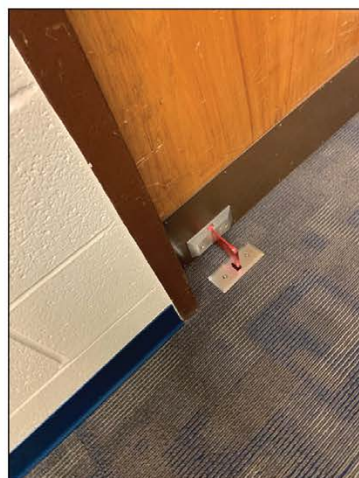
A supplemental barricade on a classroom door in a school in Michigan. Students are trained on how to use this in an emergency.
