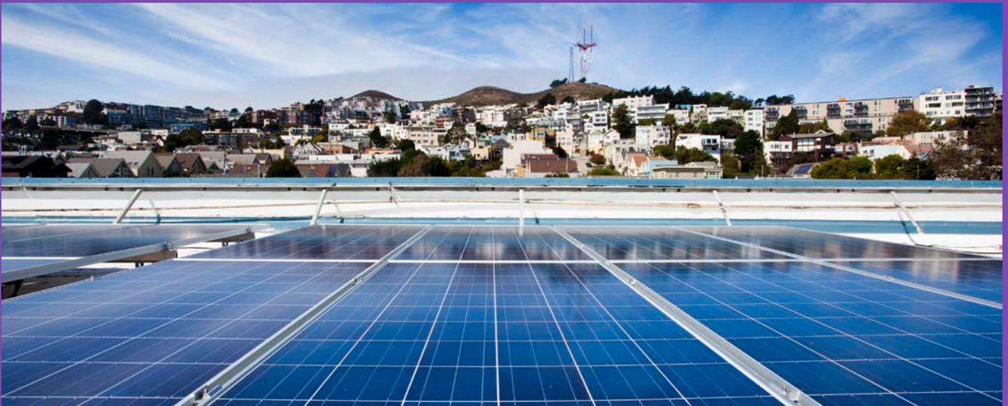
The 50-kW PV system on Alvarado Elementary School in San Francisco provides 20%–30% of the school's electricity and is a tool for teaching students about environmental stewardship. Photo by SFPUC
